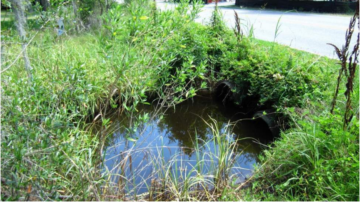
Southside Boulevard triple 30-inch crossline pipes
