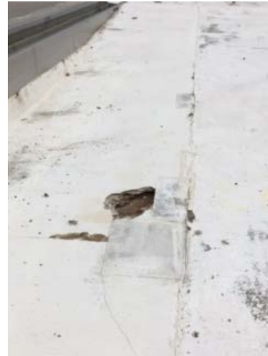
Example of some concrete work needed on pool shell
