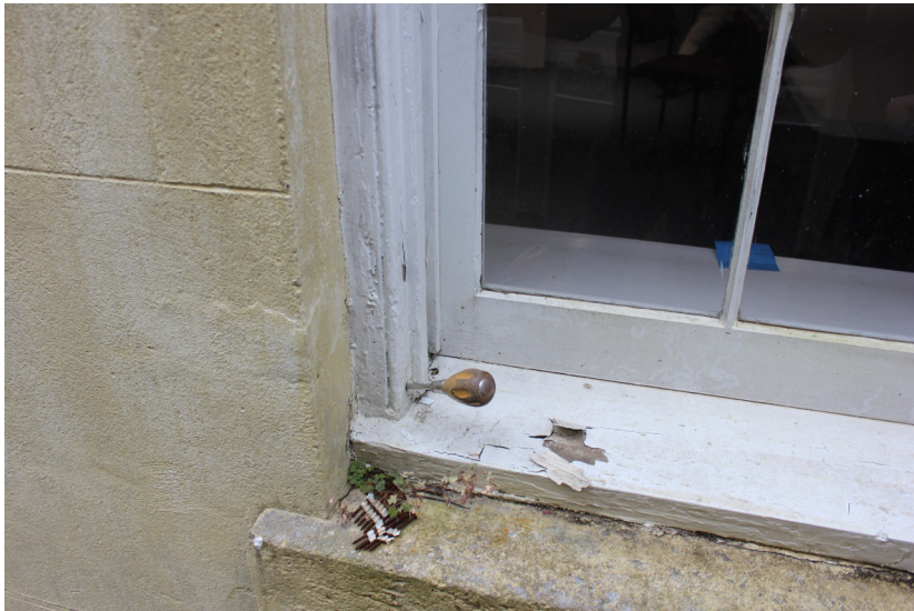
Figure 5: Detail of typical deterioration.
