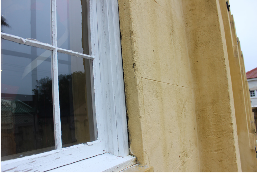
Figure 27: There is a small gap between the casing and the exterior stucco.
