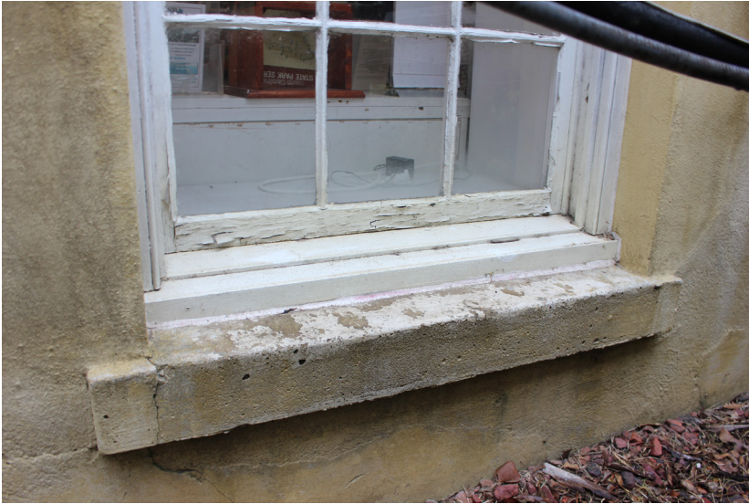
Figure 80: Glazing putty and paint failure is present throughout the window.
