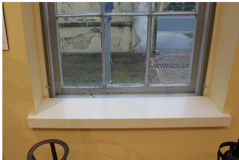
Figure 37: The lower sash is completely deteriorated and visible on the interior of the window.
