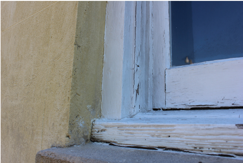
Figure 143: Separation was noted within the lower sash.
