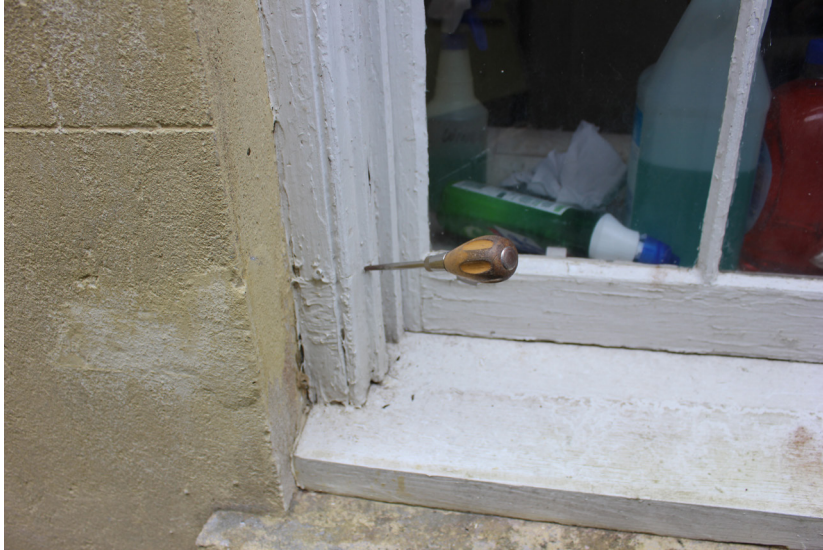
Figure 131: The casing and jamb are deteriorated at this location.
