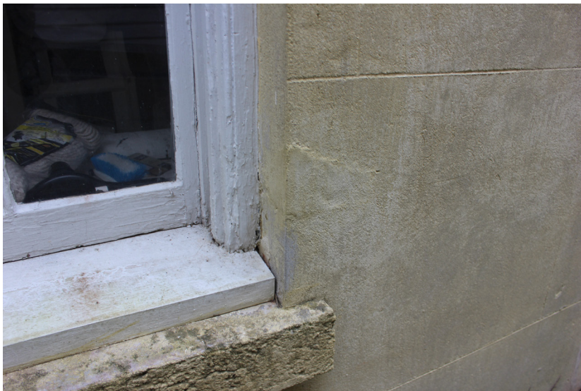
Figure 132: Detail of inappropriate repairs.
