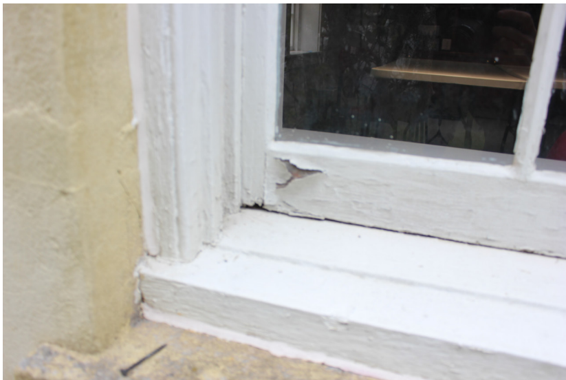
Figure 151: Detail of paint failure.
