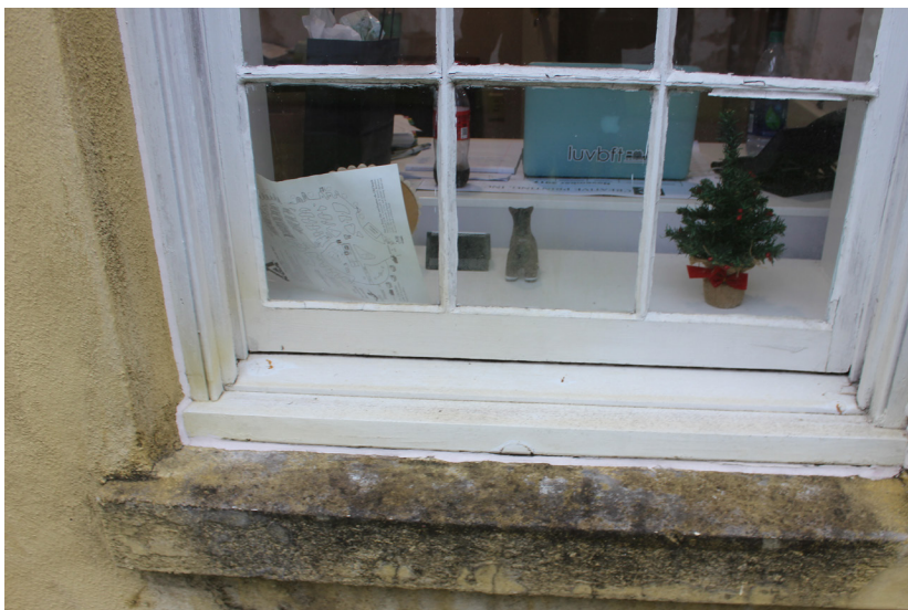
Figure 160: Detail of interior conditions and sill. A knot is present within the sill.
