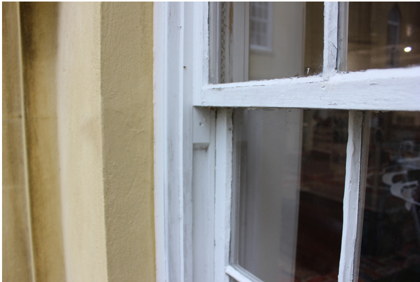
Figure 64: Glazing putty and paint failure is present throughout the window.
