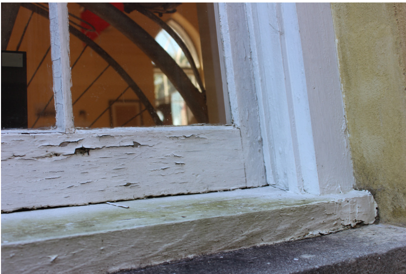
Figure 108: The bottom rail of the lower sash is deteriorated.
