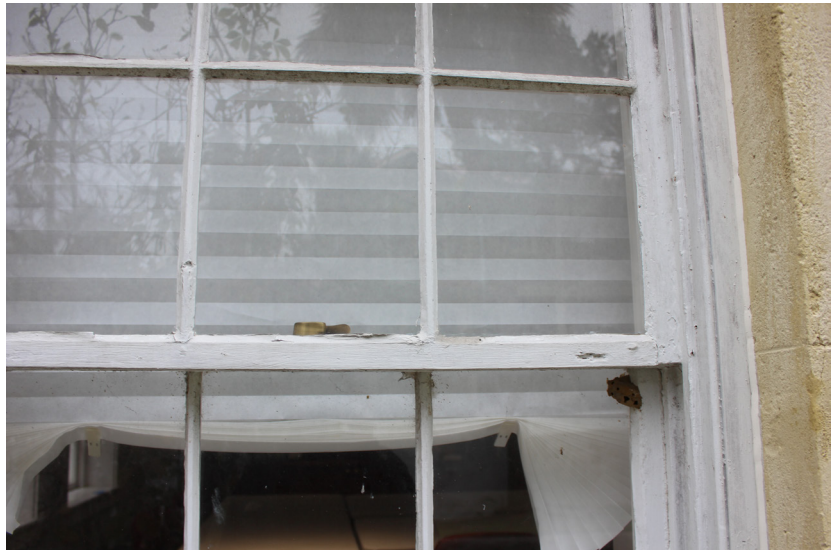
Figure 2: Glazing putty failure is prominent feature on all the inspected windows.
