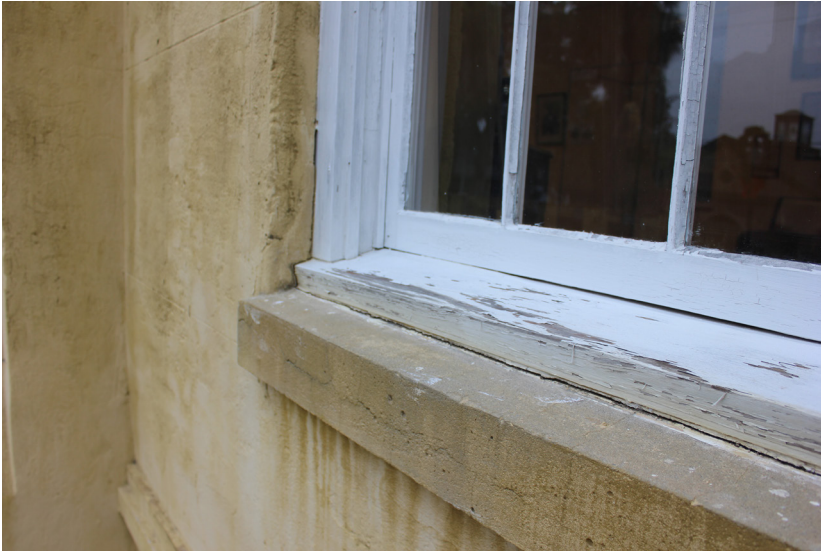
Figure 32: The bottom rail of the lower sash is deteriorated and requires replacement.
