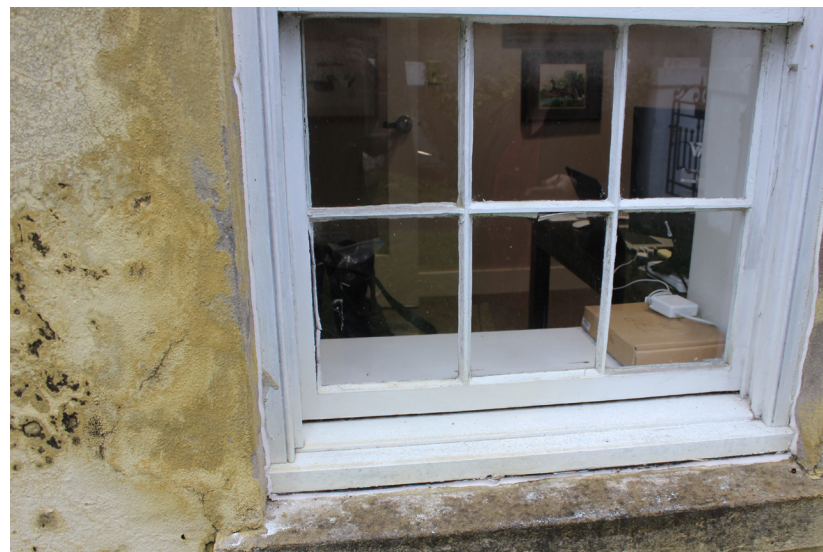
Figure 164: Detail of interior conditions at the stool the location of the and gap between sill and lower sash.
