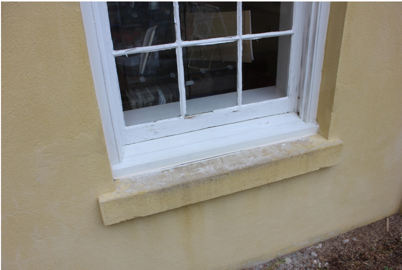
Figure 68: The bottom rail of the lower sash is weathered but sound.
