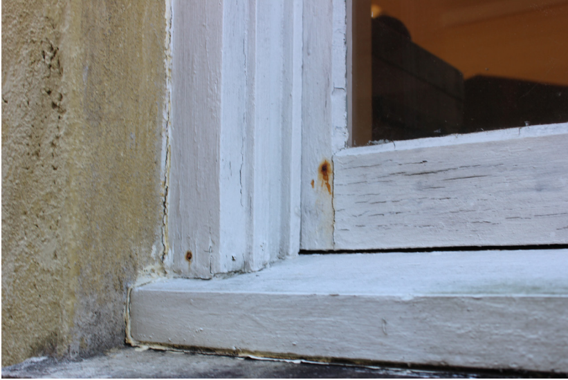
Figure 119: The ferrous fasteners within the window are actively corroding.
