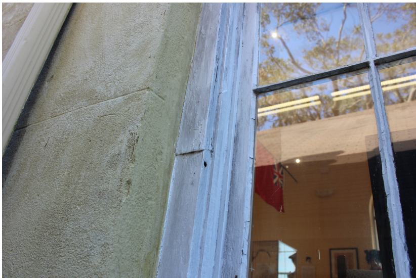
Figure 6: Category 2 windows commonly contain dutchman repairs that are actively separating.
