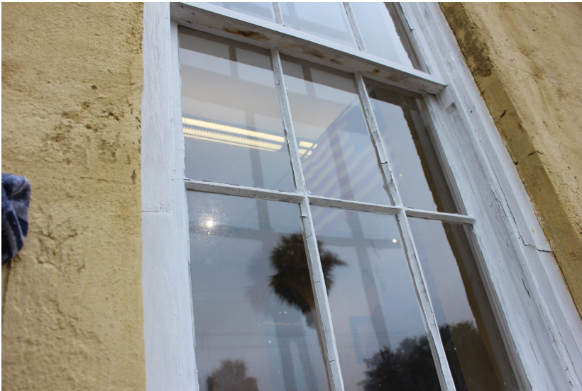
Figure 24: There is extensive paint and glazing failure throughout the window.
