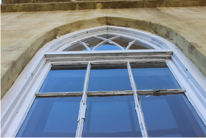
Figure 99: A dutchman repair is present within the transom casing.
