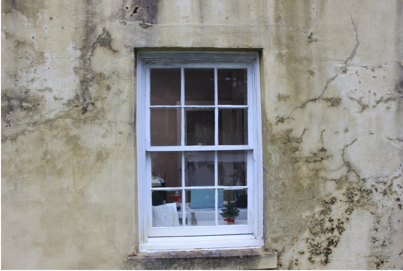
Figure 158: Biogrowth is present throughout the masonry opening.
