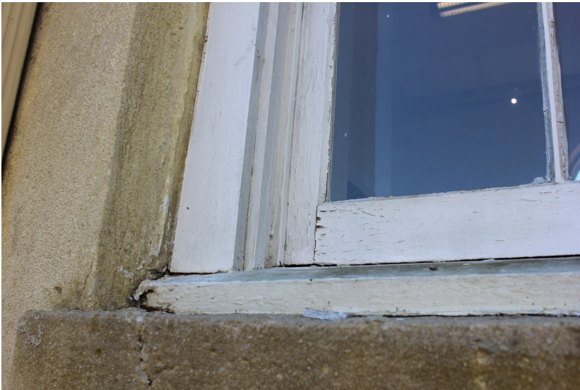
Figure 96: Detail of separation at the joints within the lower sash.
