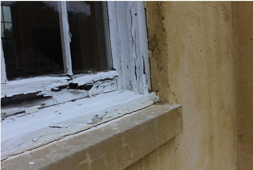
Figure 36: The lower sash is completely deteriorated.
