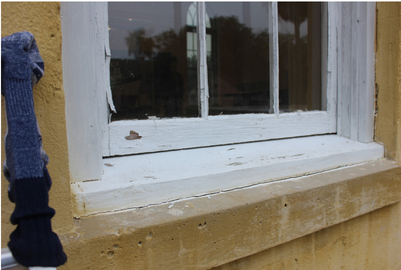
Figure 40: The lower sash is weathered but appears sound.
