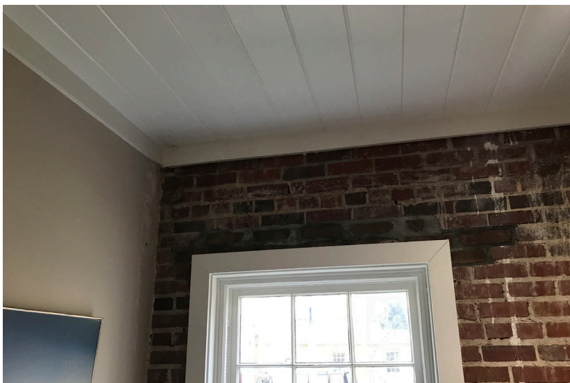
Figure 57: Detail of interior conditions. A leak is present within the masonry above this window.
