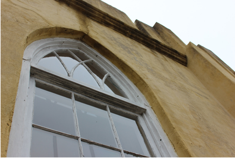
Figure 43: The transom casing is slightly proud of the lower window casing. A pane of glass is broken within the transom.
