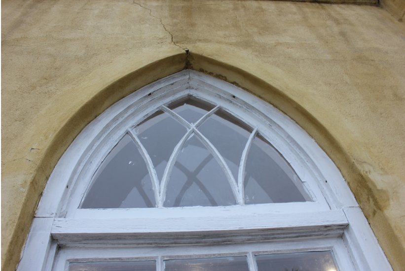
Figure 51: The transom casing is beginning to separate at the joints. The glass is in good condition.
