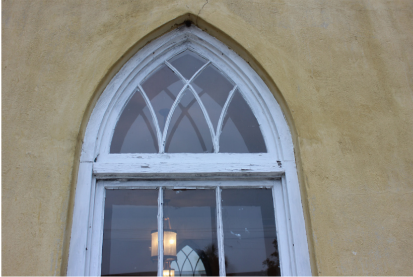
Figure 47: The transom bar is heavily weathered.
