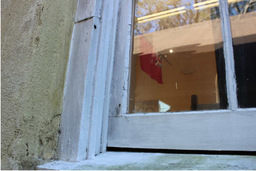
Figure 111: Detail of dutchman repair that is separating at the joints.
