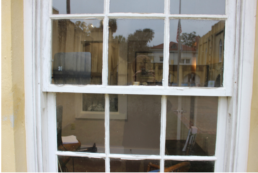
Figure 55: Glazing putty and paint failure are present throughout the window.
