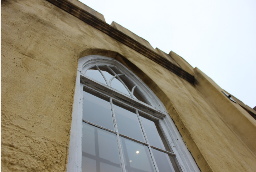
Figure 35: The transom casing is proud of the lower window casing.
