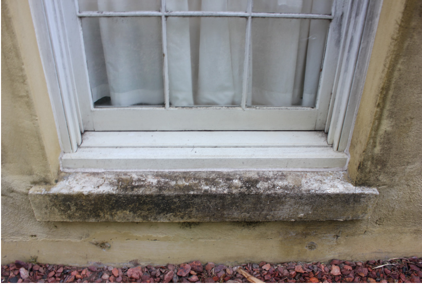
Figure 71: Biogrowth is present throughout the window.
