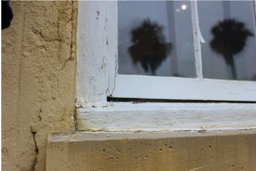
Figure 4: Category 2 windows typically have evidence of deterioration or excessive weathering on the casing and the sills.
