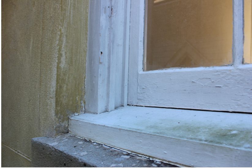
Figure 123: The sill is in good condition. Biogrowth is present throughout.
