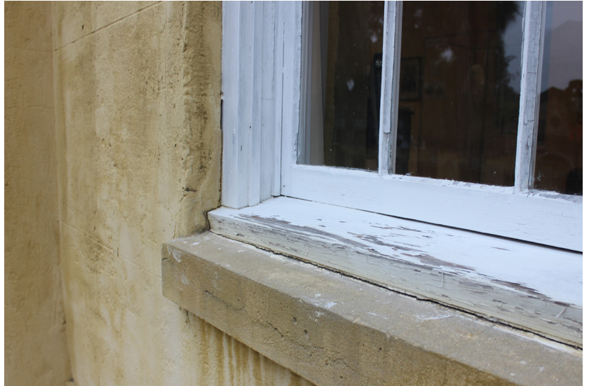
Figure 1: Category 1 windows typically have extensive paint loss.
