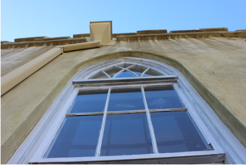
Figure 91: There is extensive glazing and paint failure throughout the window.
