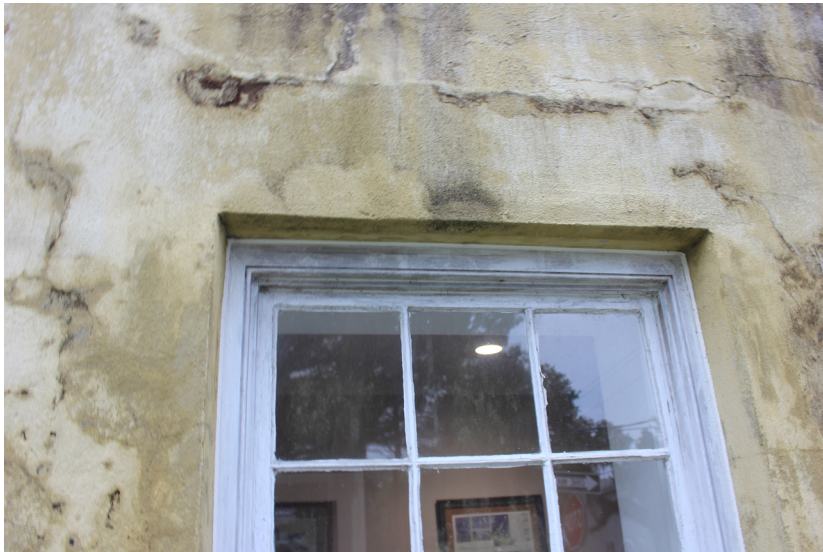
Figure 163: Biogrowth is present throughout the window and the masonry opening.
