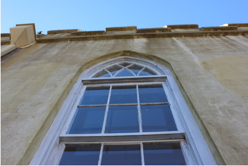
Figure 87: There is extensive glazing and paint failure throughout the window.
