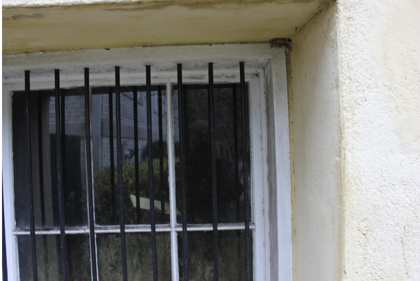
Figure 83: The head of the window is in fair condition.
