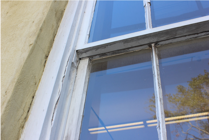
Figure 100: Detail of paint and glazing failure.
