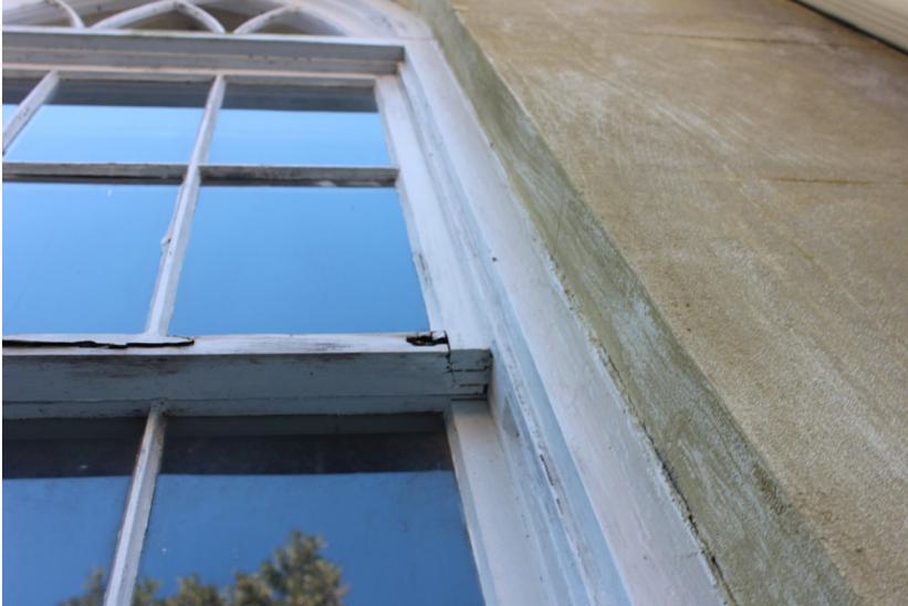
Figure 127: The lower rail of the upper sash is deteriorated.
