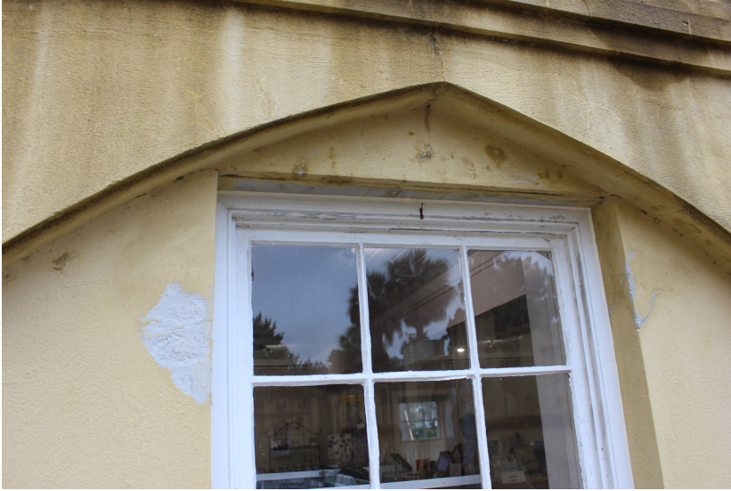
Figure 67: A small gap is present between the steel lintel and the wood casing at the head of the window.
