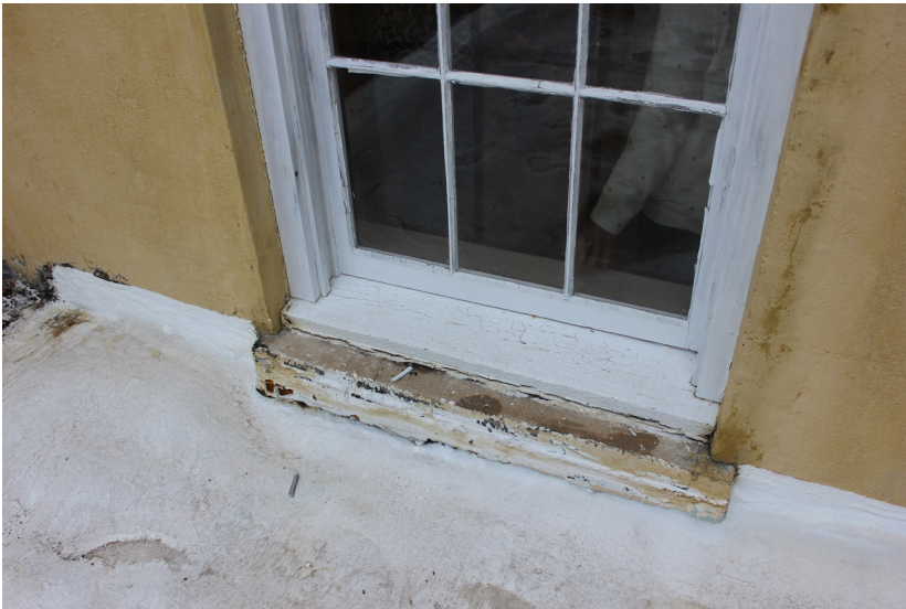
Figure 48: The sill is heavily weathered.
