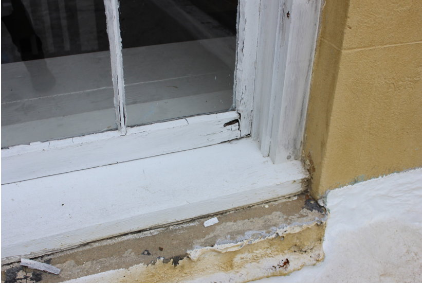
Figure 15: The lower sash is deteriorated along the bottom rail.
