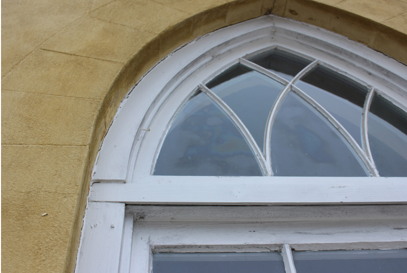
Figure 11: The casing of the transom window does not align with the lower casing.
