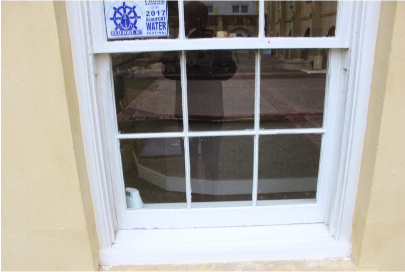
Figure 60: The bottom of the jamb and casing where it intersects the masonry sill is not caulked.
