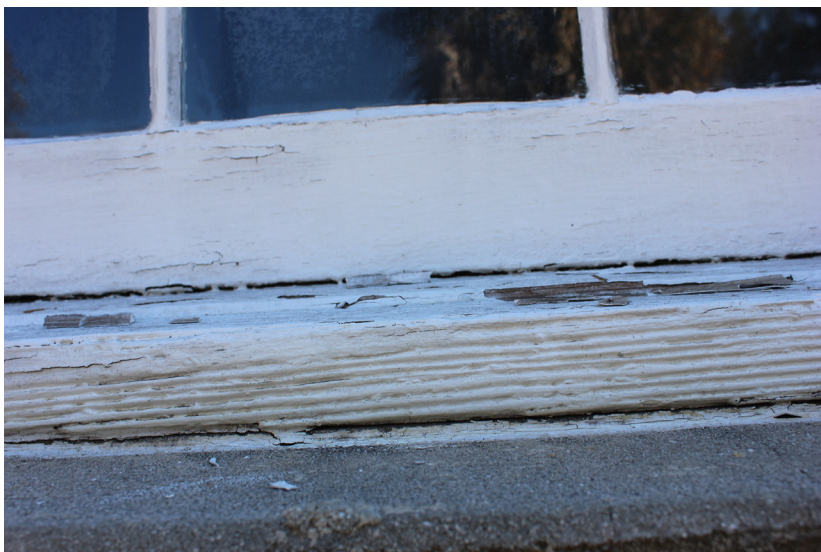
Figure 144: The sill is heavily weathered.
