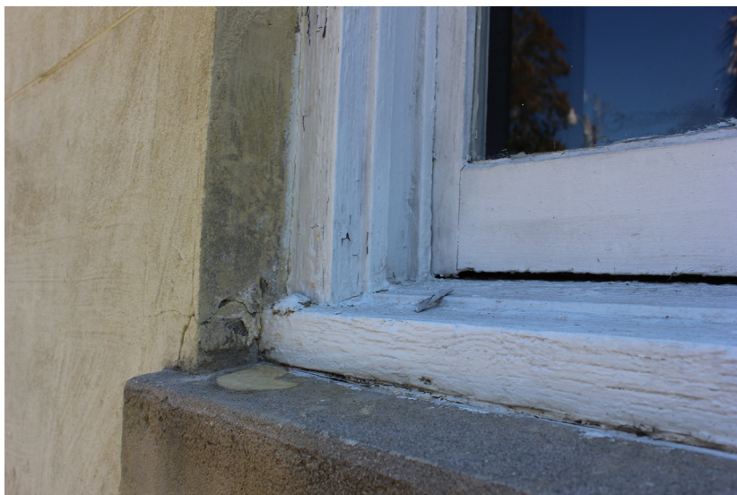
Figure 148: The sill is weathered but sound.
