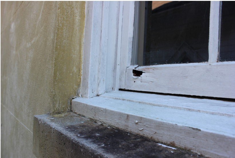
Figure 128: The bottom rail of the lower sash is deteriorated.
