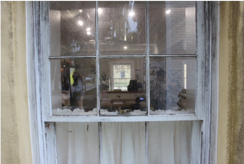
Figure 72: The woodwork is in fair condition. Biogrowth is present on the wooden elements.
