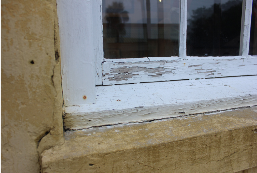
Figure 28: The bottom rail of the lower sash is heavily weathered and is separating at the joints.
