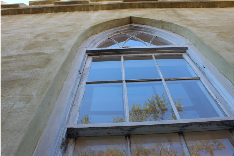
Figure 107: The transom casing is proud of the lower casing.
