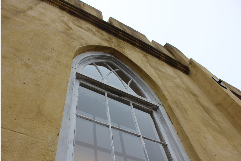
Figure 39: The transom casing is slightly proud of the lower window casing.
