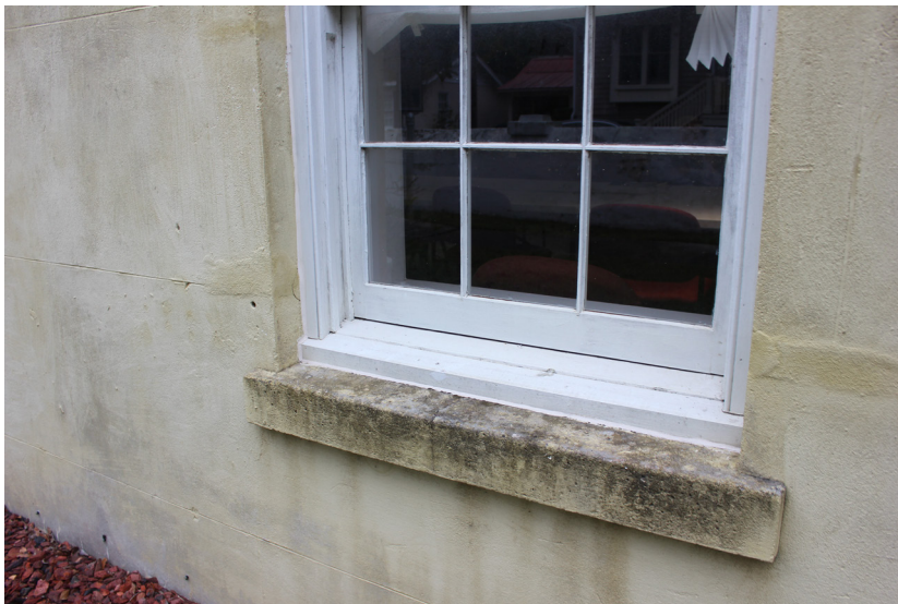
Figure 155: A small gap is present between the lower sash and the wood will.
