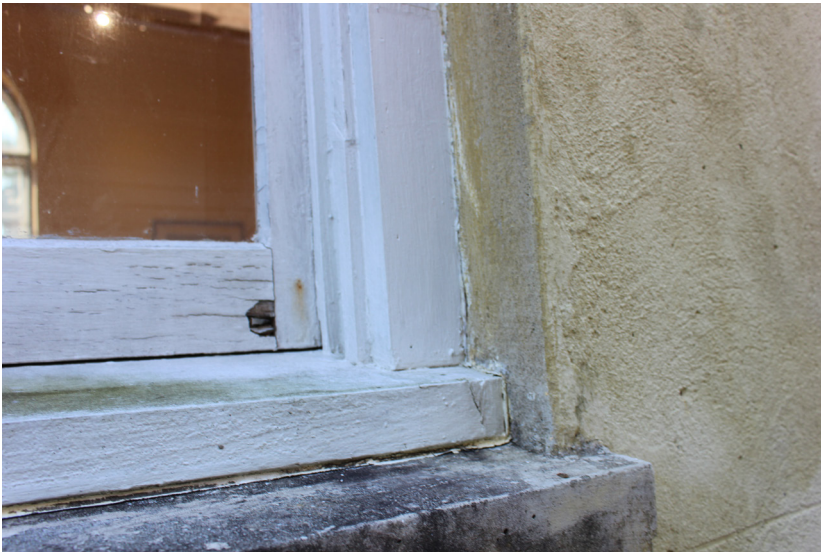
Figure 120: Detail of sash deterioration.
