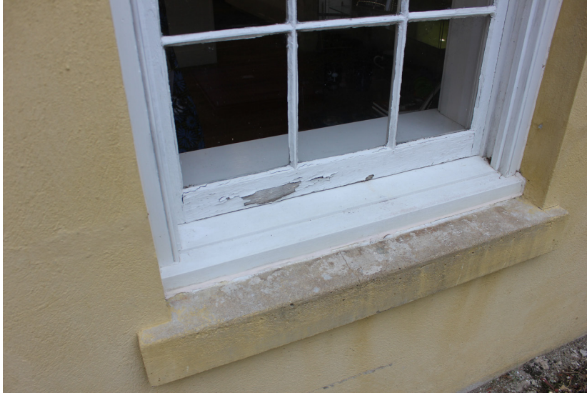
Figure 63: The bottom rail of the lower sash is heavily weathered.
