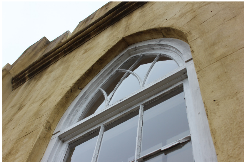
Figure 3: Detail of casing of transom windows that is proud of the lower casing. This condition is typical on the second-floor windows.
