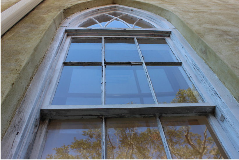
Figure 103: The casing on the left and right hand sides of the window are deteriorated.
