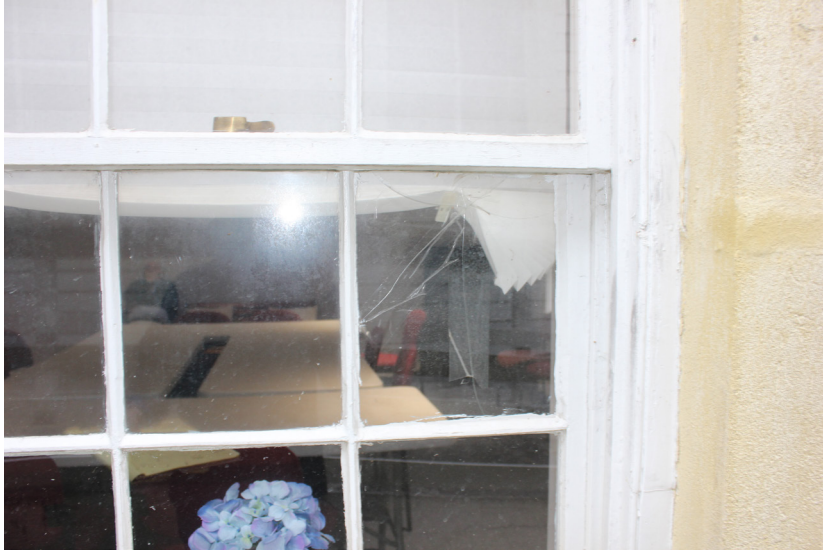
Figure 138: Detail of broken glass.
