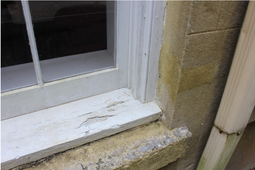
Figure 135: The sill is heavily weathered and checked but is sound.
