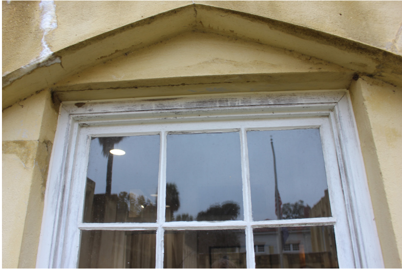
Figure 56: The masonry opening is cracked above the head of the window.
