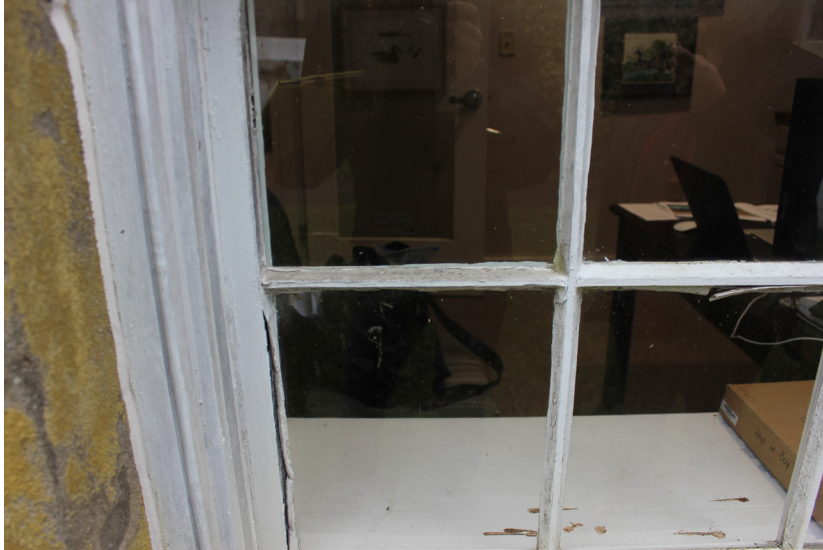
Figure 162: Detail of glazing failure
