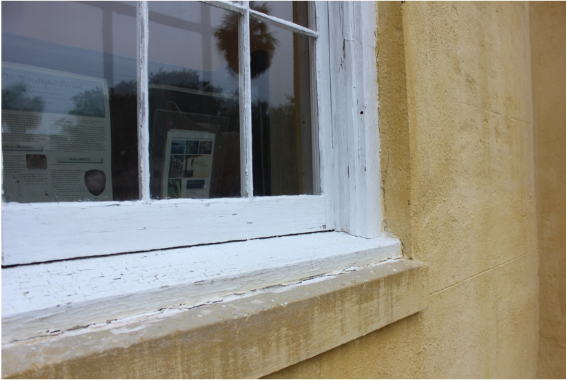
Figure 44: Several dutchman are present within the casing. The casing is soft at the lower portions of the window.
