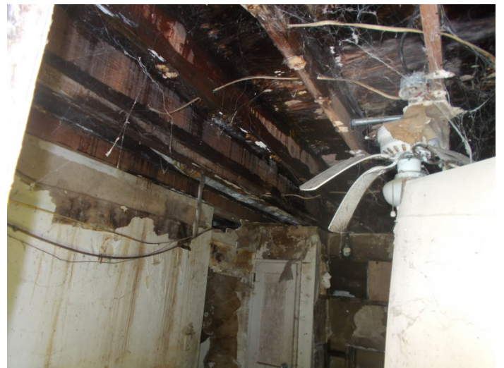
Photo 16 – Fire damage throughout Building 8.
