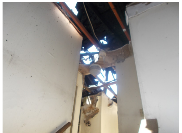
Photo 18 – Fire damage throughout Building 8.
