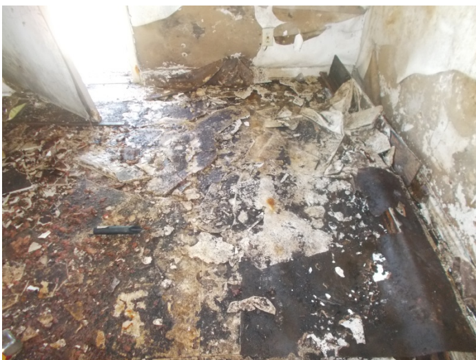
Photo 17 – Fire damage throughout Building 8.
