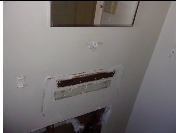
Photo 7 – Typical view of the bathroom sink caulk in buildings 1-6 & 36-38.
