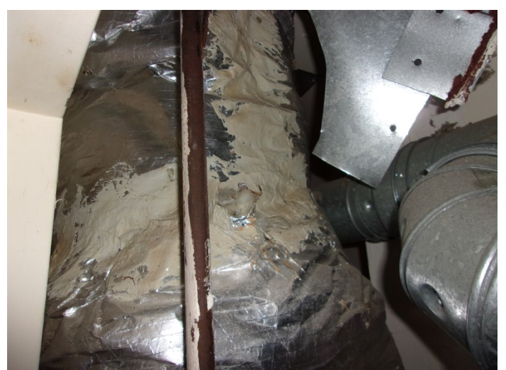
Photo 4 – Beige HVAC mastic above the ceiling and in HVAC closet in building 37.
