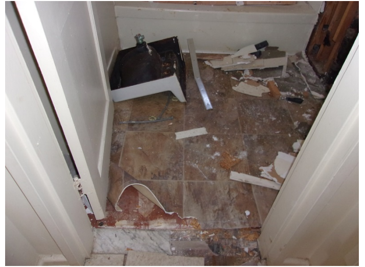
Photo 20 – Typical view of vinyl flooring & mastic in portions of the buildings (no ceramic tile exists).
