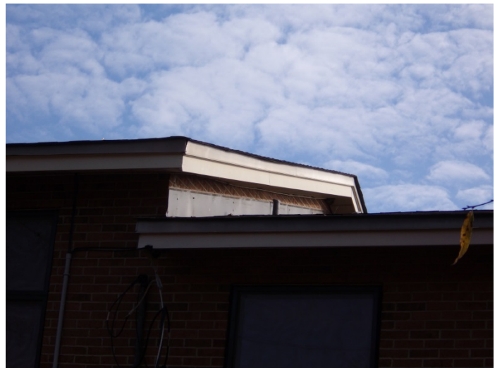
Photo 16 – Typical view of the caulk on the main roof flashing on buildings 1-6 & 36 & 38.
