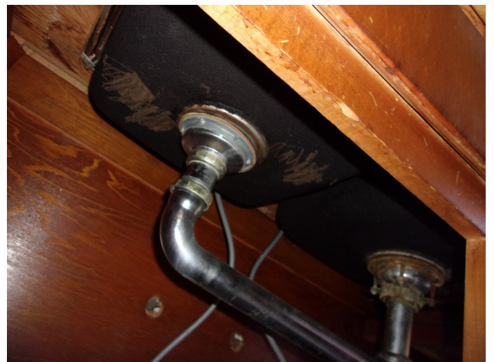
Photo 6 – Typical view of the black kitchen sink coating in buildings 1-6 & 36-38.
