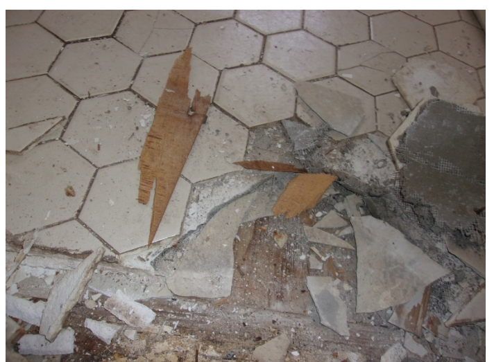
Photo 18 – Typical view of ceramic tile with wood & vinyl flooring beneath throughout buildings 1-6 & 36-38.
