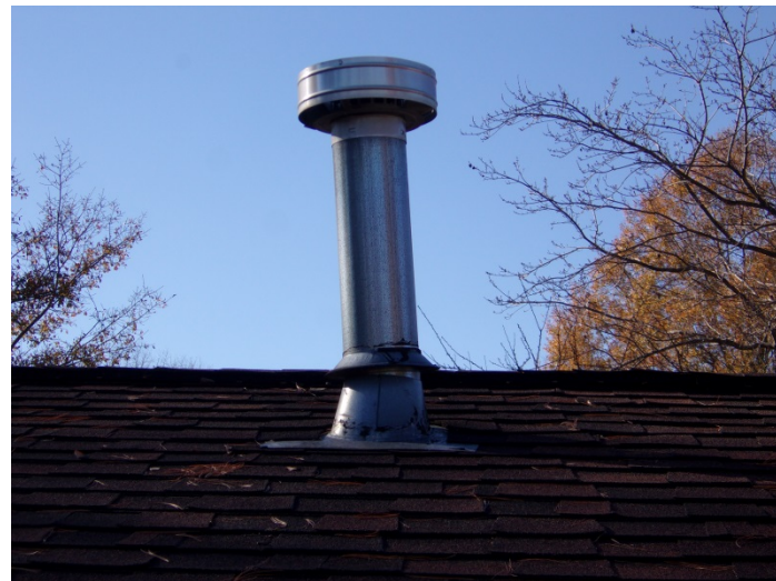
Photo 11 – Typical view of black & black/gray mastic/tar on roof penetrations on buildings 1-6 & 36-38.
