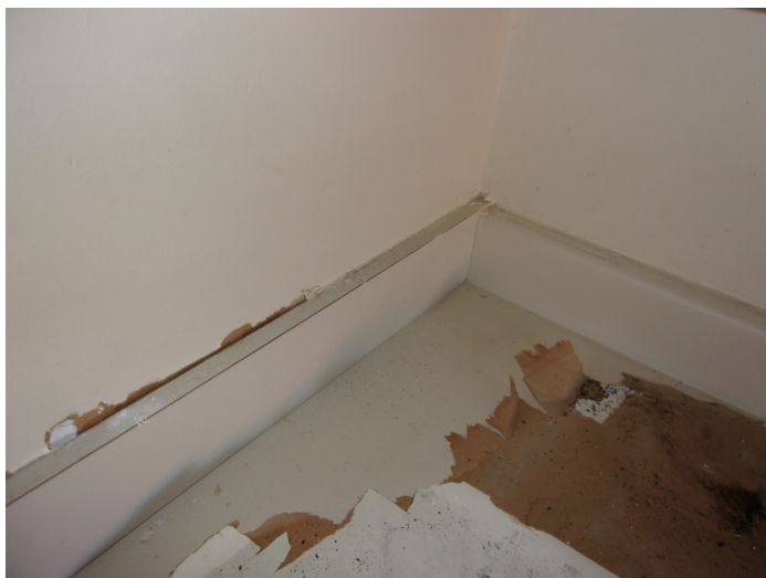
Photo 5 – Typical view of kitchen counter caulk throughout buildings 1-6 & 36-38.
