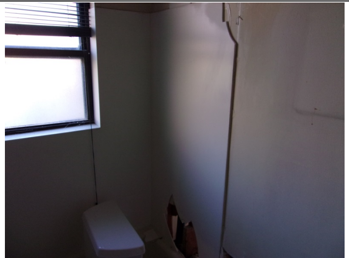
Photo 8 – Typical view of the shower stall caulk in buildings 1-6 & 36-38.
