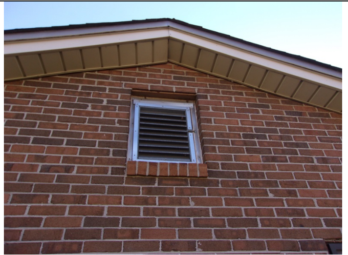
Photo 14 – Typical view of roof gable vents with caulk on buildings 1-6 & 36-38.
