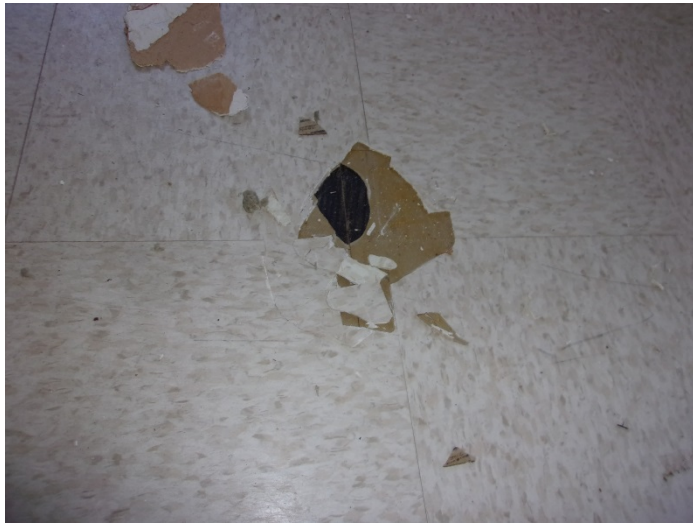
Photo 3 – Typical view of 12'' x 12'' tan speckled floor tile & mastic over 2 nd layer of floor tile & mastic over concrete throughout buildings 1-6 & 36-38.
