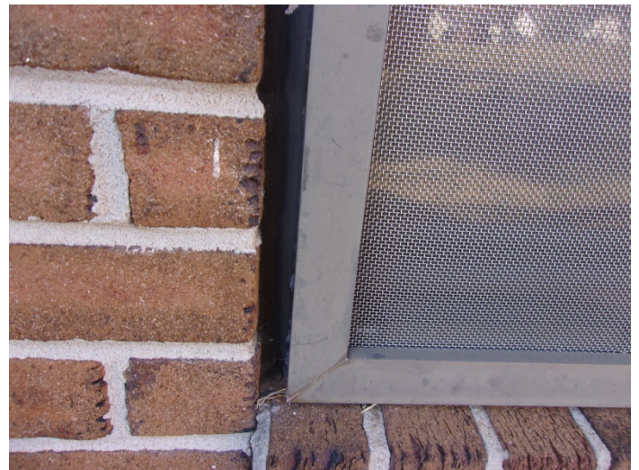
Photo 12 – Typical view of the black and brown interior and exterior window caulk in buildings 1-6 & 36-38.
