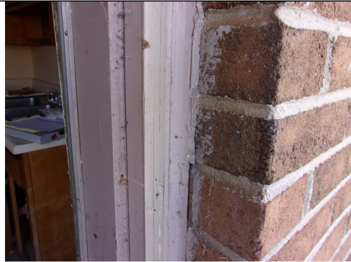
Photo 13 – Typical view of the door caulk in buildings 1-6 & 36-38.
