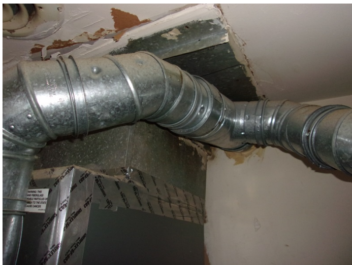
Photo 21 – Typical view of caulk on the HVAC units throughout the HVAC closets in buildings 1-6 & 36-38.
