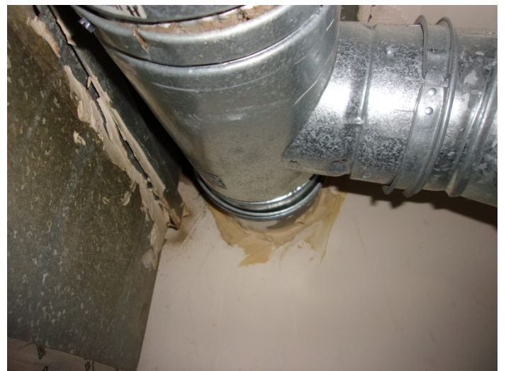
Photo 22 – Typical view of caulk on the HVAC units throughout the HVAC closets in buildings 1-6 & 36-38.
