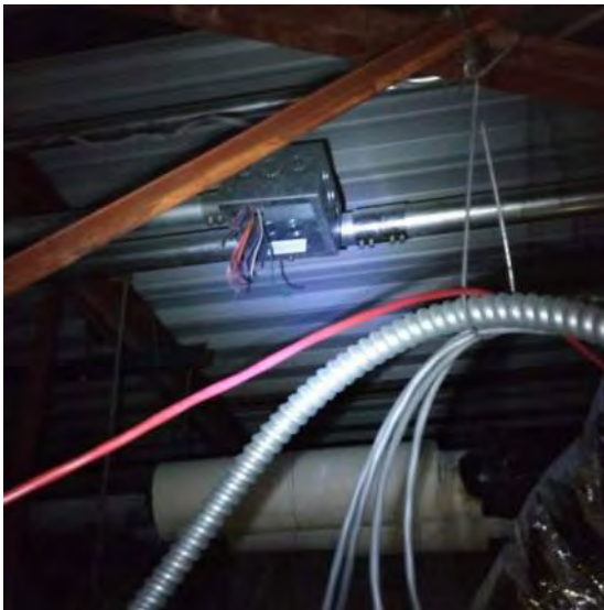
Exposed Wiring above Ceiling
