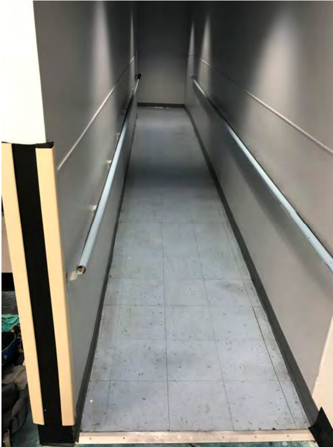
Non-Compliant ADA Handrails and Faded and Damaged Finishes
