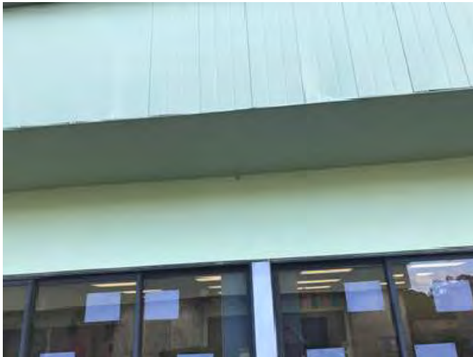
Fascia Allowing Water Infiltration
