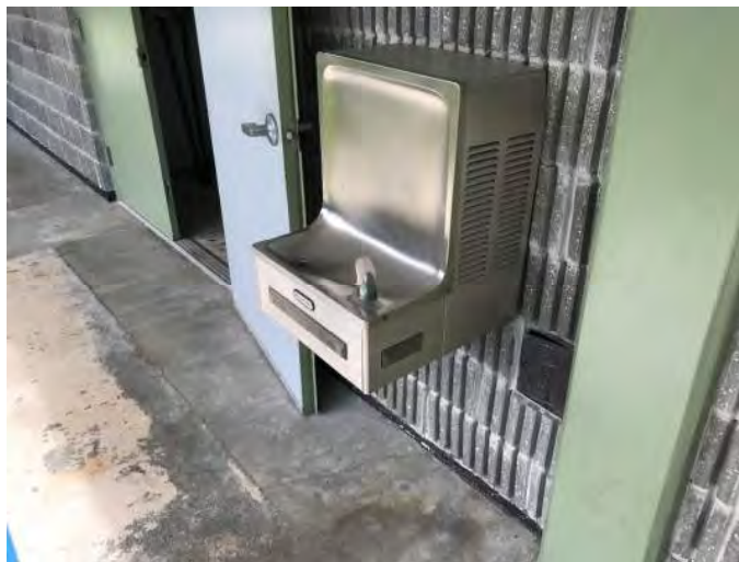
Non-Compliant ADA Drinking Fountain
