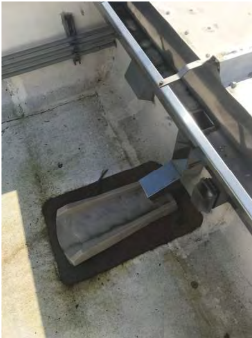
Buildings 2, 3 & 5 Slash Block at HVAC Unit
