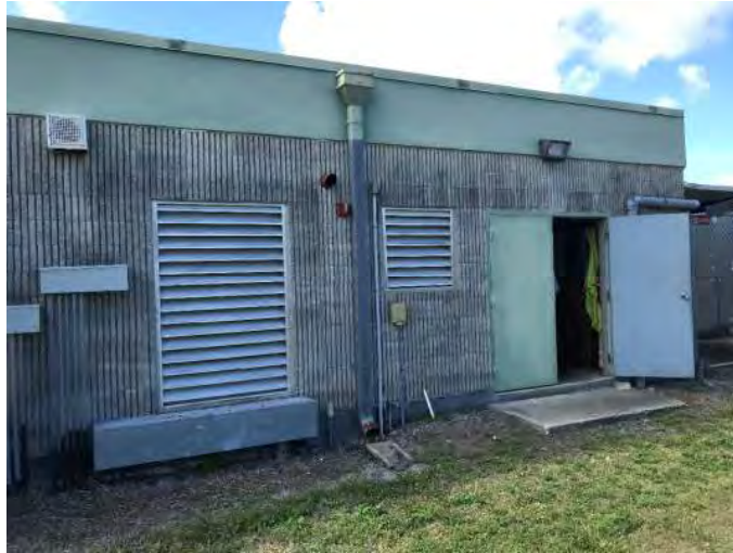
Building 8, Fluted CMU Showing Mold, Corrosion Occurring to Louvers and Door & Non- Compliant ADA Hardware
