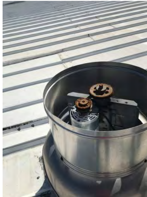
Buildings 2, 3 & 5 Top of Hood Missing
