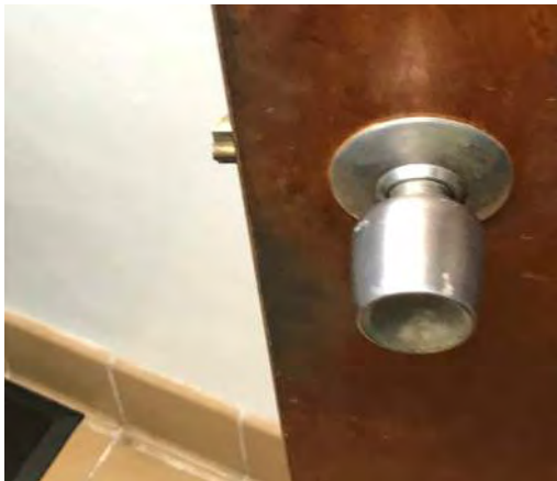
Buildings 2, 3 & 5 Door and Hardware Not ADA Compliant
