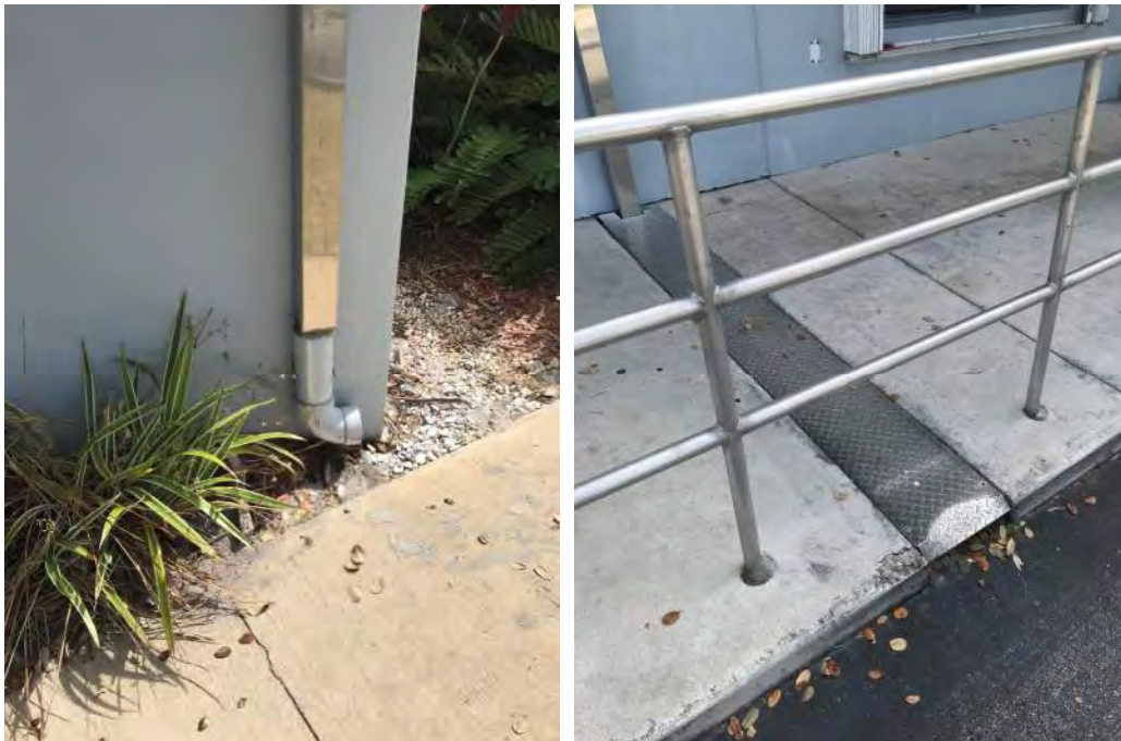
Storm Drainage Not Tied in to the Underground Storm Sewer System
