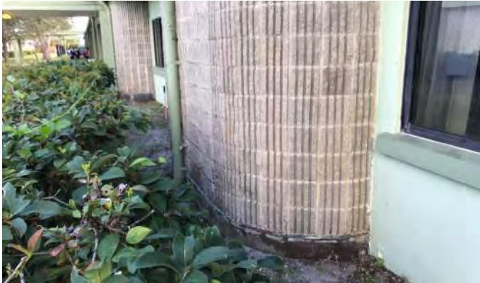
Water Infiltration in Exterior Wall and Corrosion of Fluted CMU Masonry Ledge
