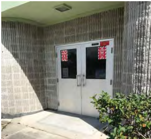
Non-Compliant ADA Hardware
