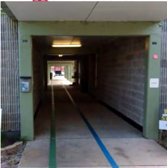
Insufficient Exterior Corridor Lighting
