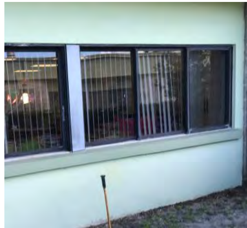
Windows Do Not Meet Current FBC Pressure Requirements
