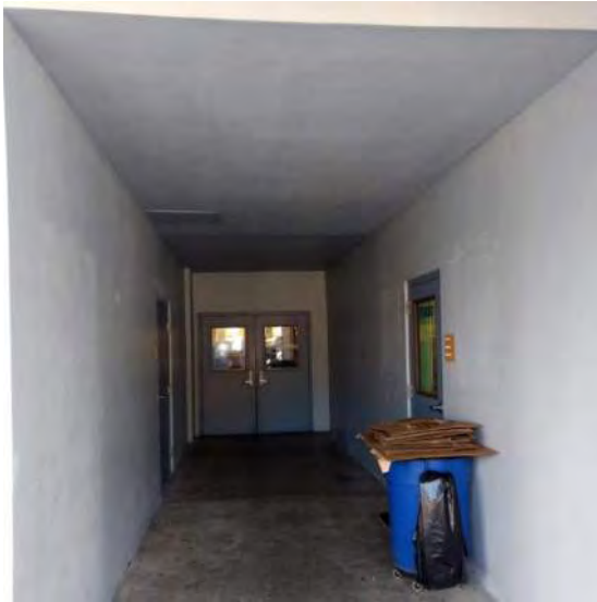
Exterior Lighting Needed
