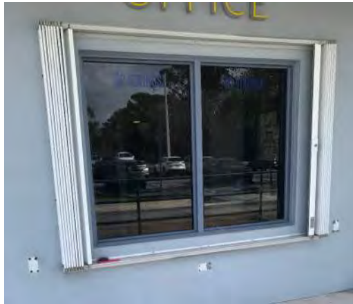
Buildings 2, 3 & 5 Existing Window Does Not Meet FBC Pressure Requirements
