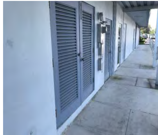
Buildings 2, 3 & 5 Door and Hardware Not ADA Compliant
