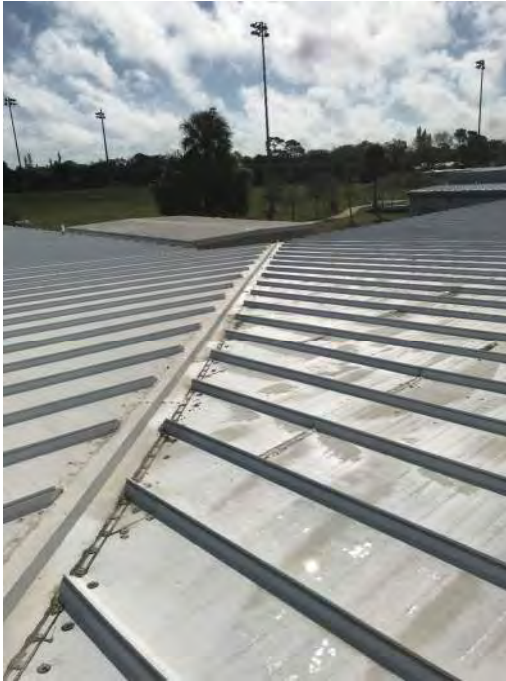
Buildings 2, 3 & 5 Finish Failing
