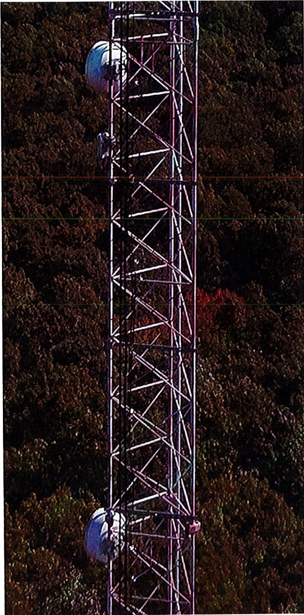
Figure 2 - 240' Microwave Array (Items C, D, E)
