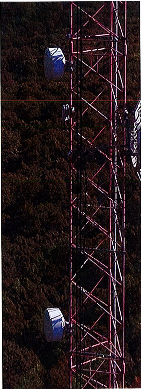
Figure 3 - 140' Microwave Array (Items F, G, H)
