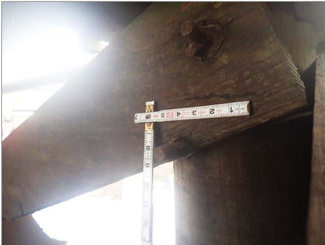
Photo 6: Hardware – Major Corrosion with Section Loss
