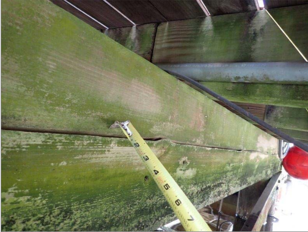
Photo 11: Cap – Major Full Width Split, Station 2+66
