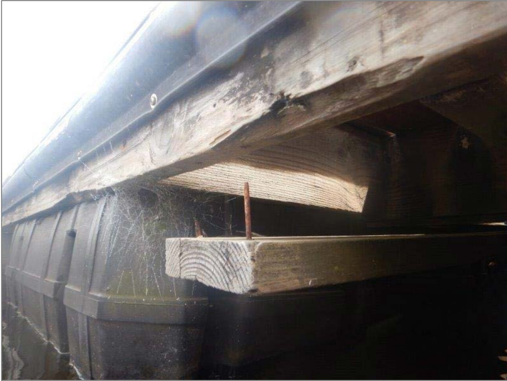
Photo 17: Floating Dock Frame – Connection Failure, Broad St. Floating Dock
