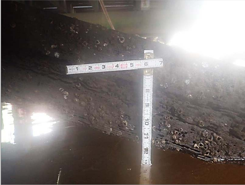
Photo 7: Cross Bracing – Major Marine Borer Activity
