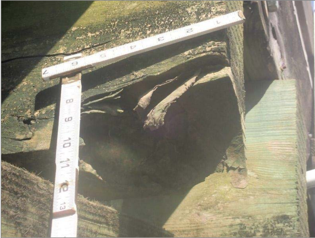
Photo 9: Cap – Major Full Width Split/Shake with Area of Associated Section Loss, Station 0+90
