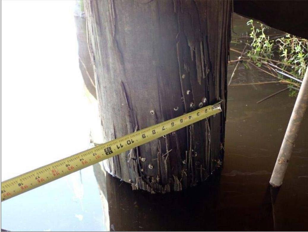
Photo 1: Pile – Minor Rot or Fungal Decay
