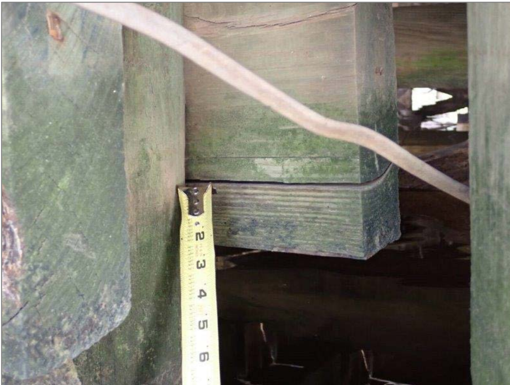
Photo 12: Cap – Major Full Width Split, Station 6+52
