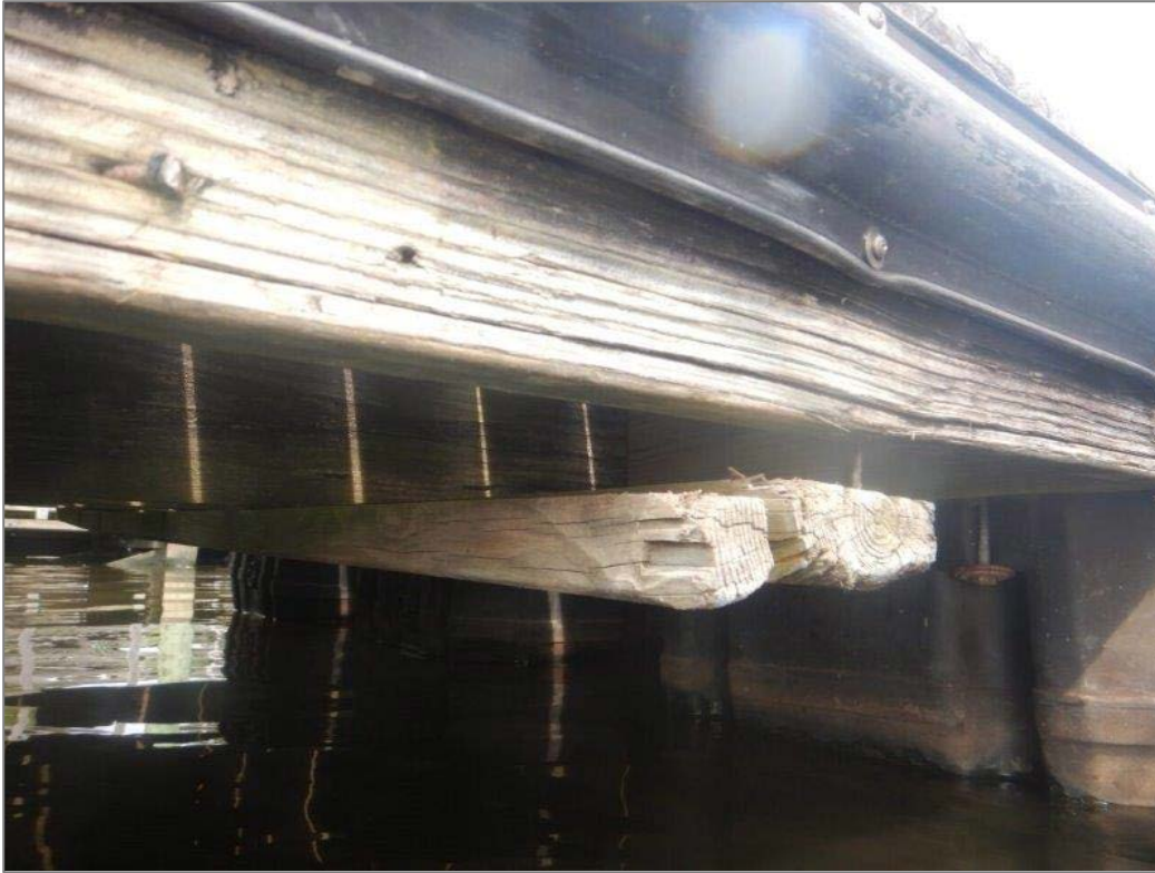
Photo 15: Floating Dock Frame – Minor Checking and Connection Hardware Failure, Screven St. Floating Dock
