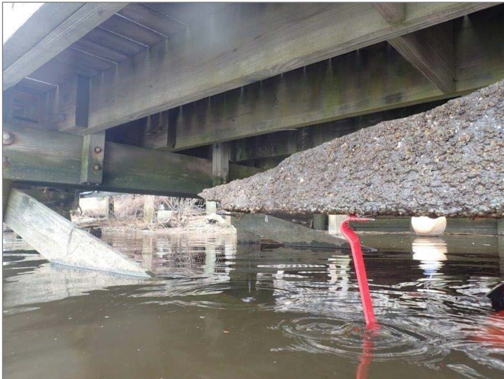
Photo 14: Cross Bracing – Severe Decay with 100 Percent Loss of Section, Station 12+40
