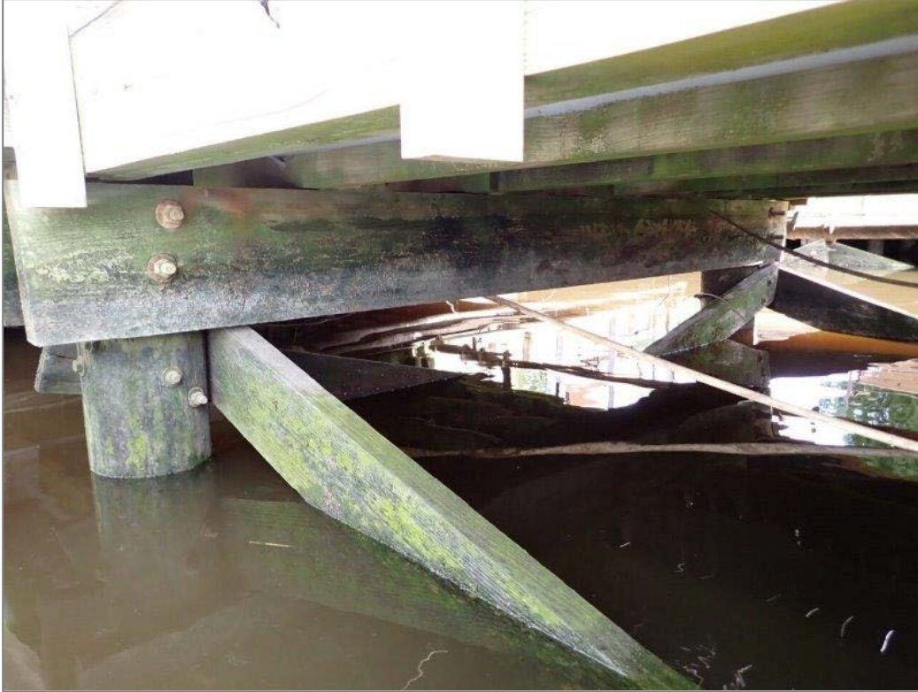
Photo 3: Cap – Minor Rot or Fungal Decay
