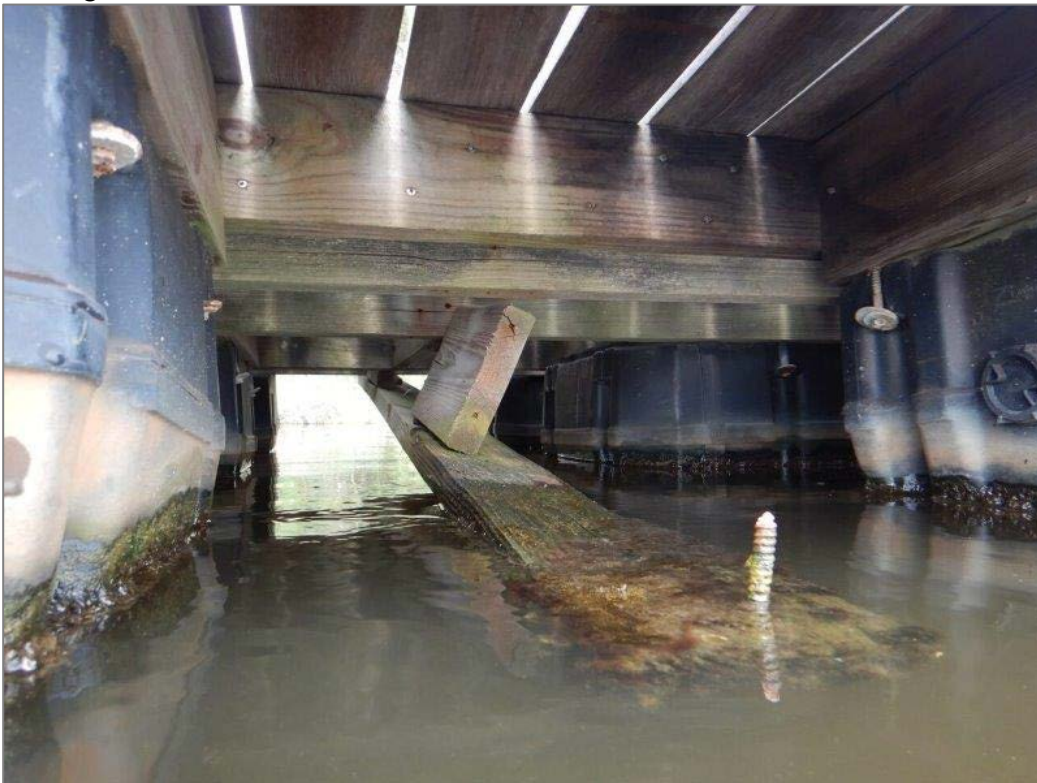
Photo 16: Floating Dock Frame – Connection Failure, Screven St. Floating Dock
