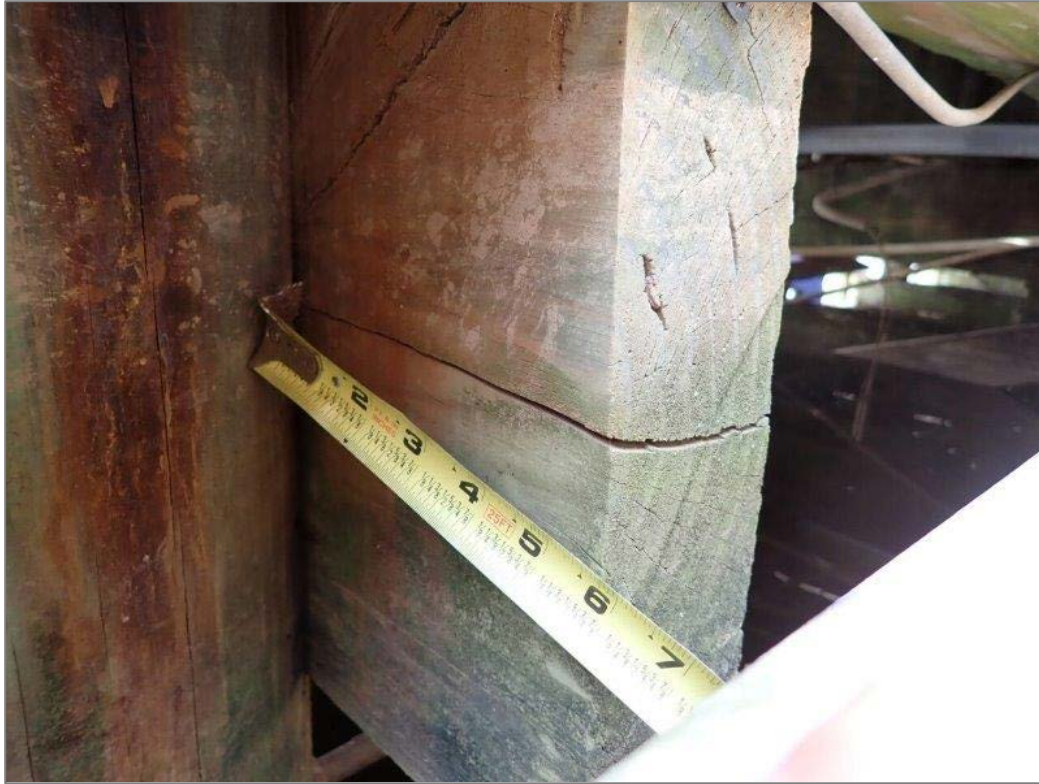
Photo13: Cap – Major Full Width Split, Station 9+26
