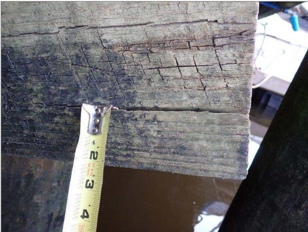
Photo 10: Cross Bracing – Major Full Width Split, Station 2+50
