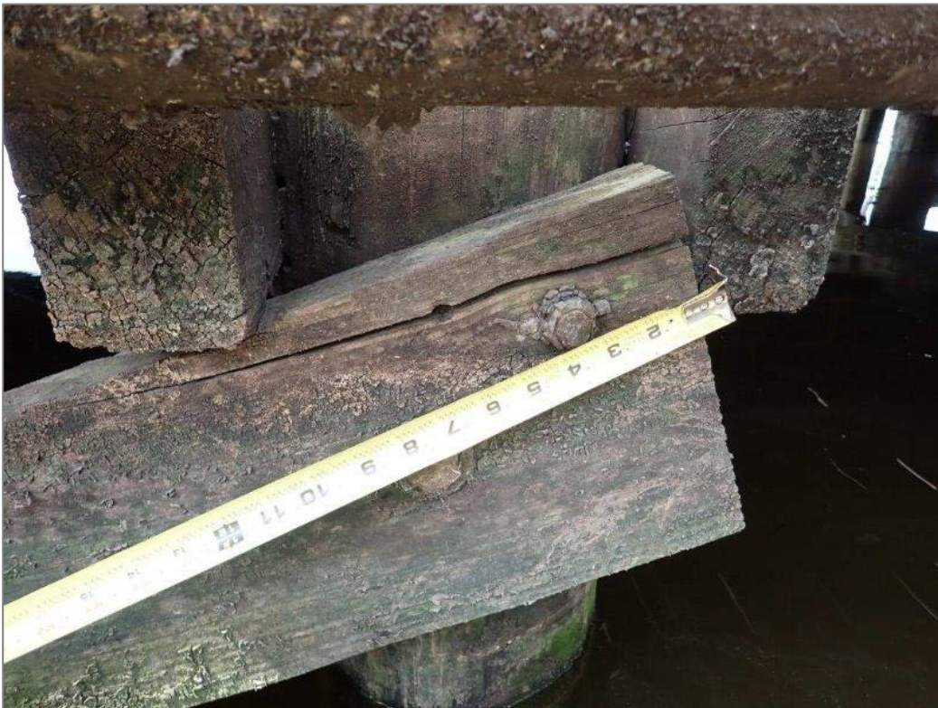
Photo 8: Cross Brace – Moderate Decay or Fungal Rot
