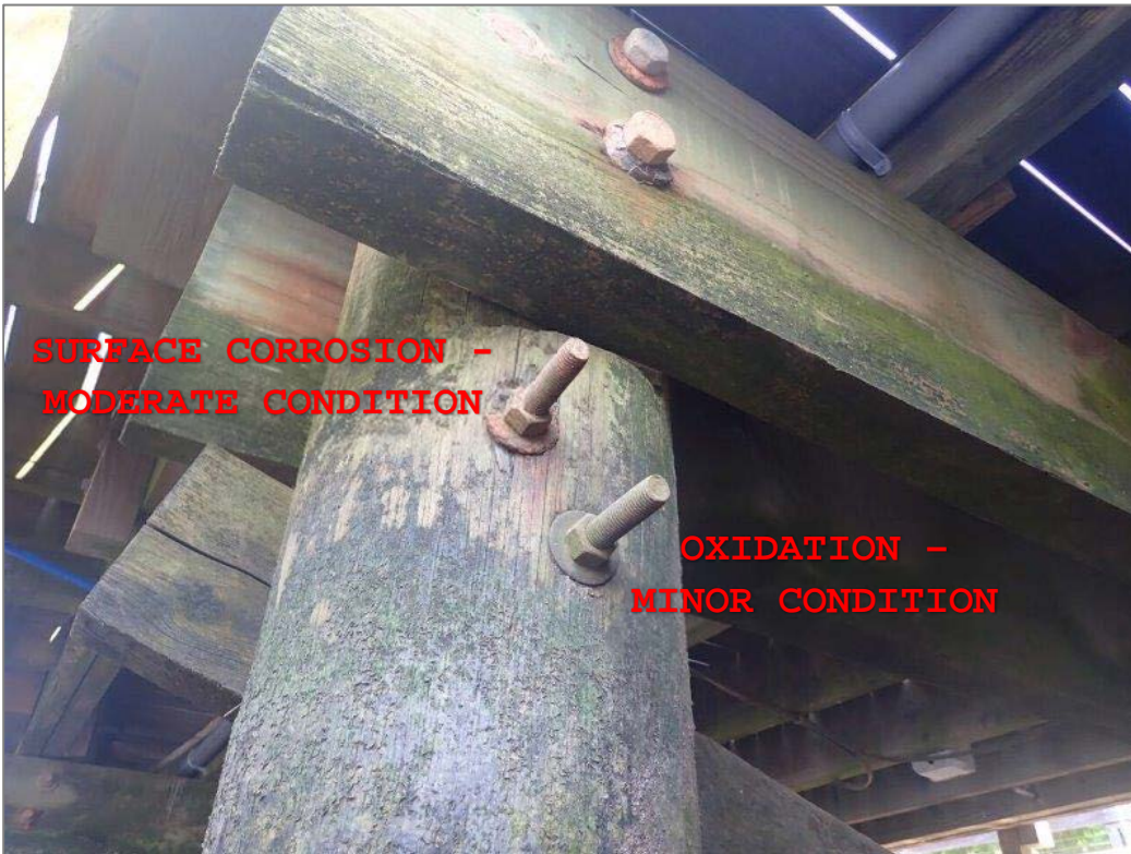
Photo 4: Hardware – Minor Surface Corrosion
