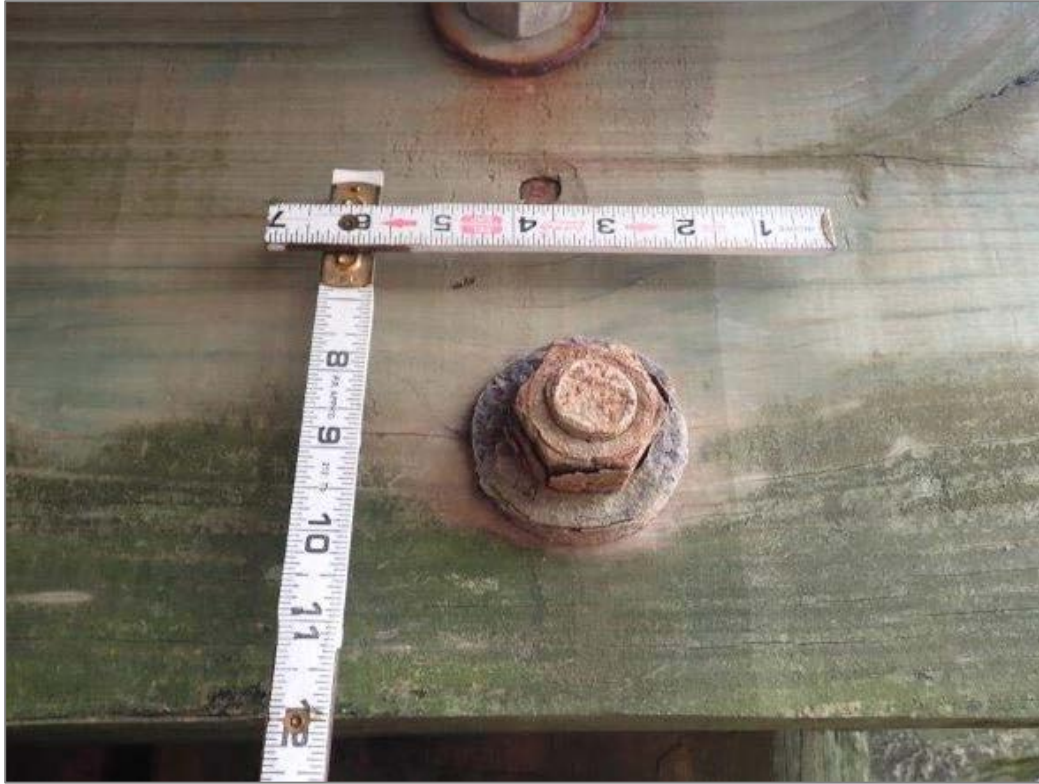
Photo 5: Hardware – Moderate Flaking Corrosion
