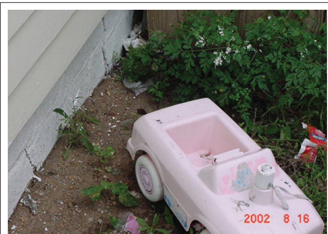
FIGURE 5.9 Soil lead hazard at dripline
