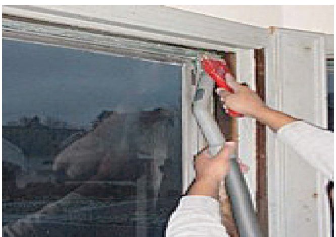
FIGURE 11.12 Vacuum window again.
