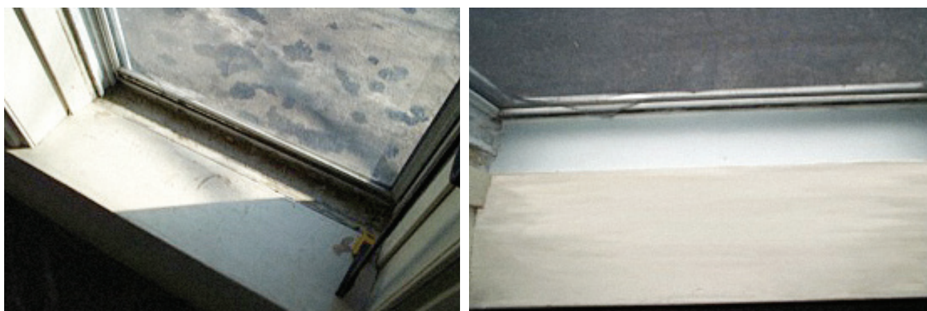
FIGURE 11.20 Turning a Window Sill and Trough Into a Smooth and Cleanable Surface. Window pre-treatment (left) and post-treatment (right).
