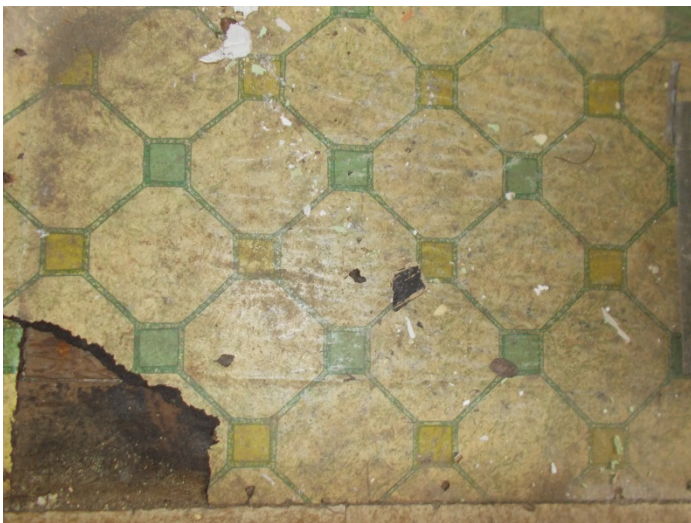
Photo 11 – Yellow/Green pattern vinyl floor with mastic.
