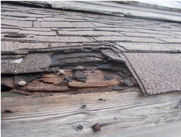
Photo 3 – Roof shingles (6 layers) and no felt.
