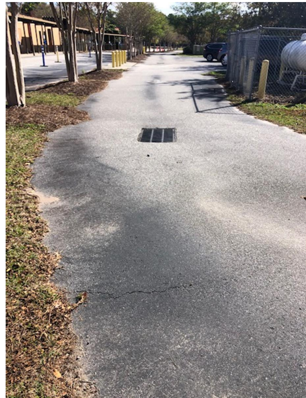
Figure 4: Low severity edge cracking
