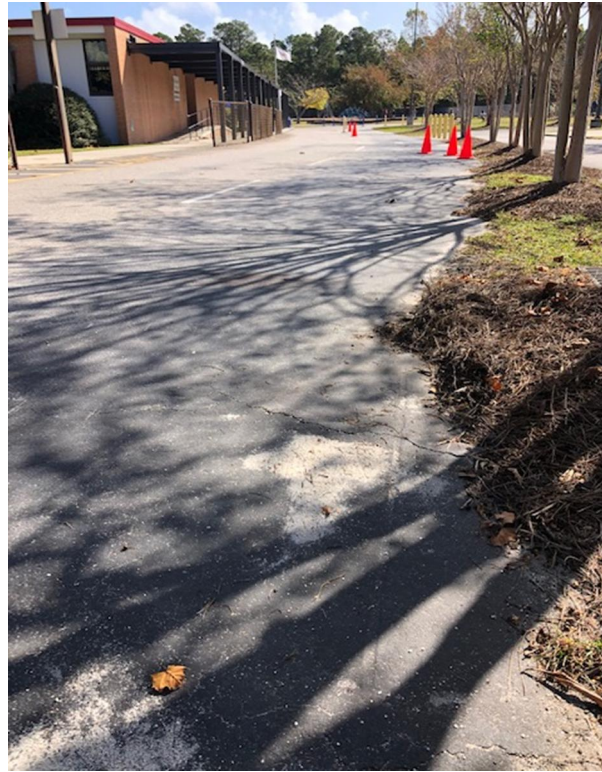
Figure 3: Low severity edge cracking
