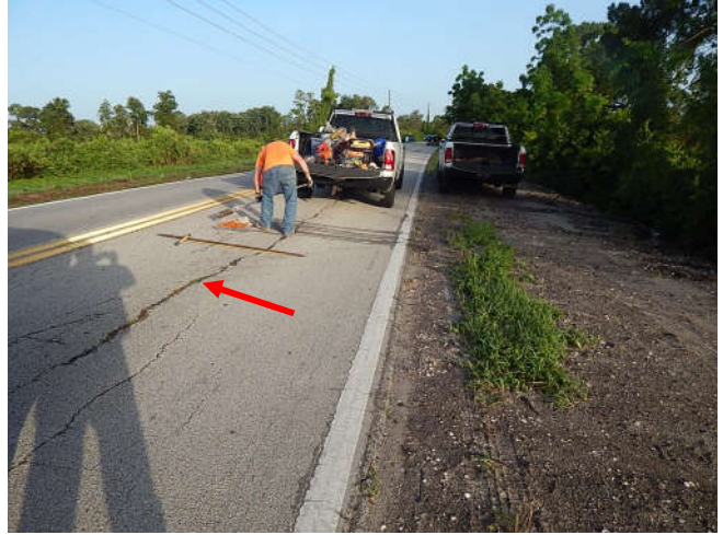
Photo 2: Location of Core No. 2 looking west (note porous longitudinal crack allowing water to enter asphalt pavement)
