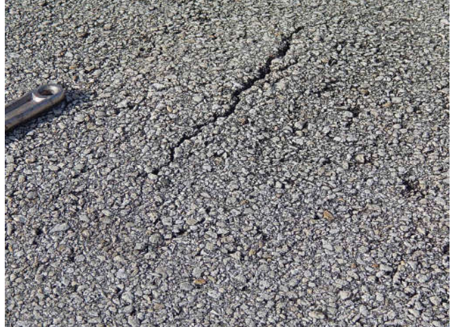
Photo 12: Close-up of Photo 11, note porous surface of asphalt
