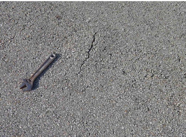
Photo 11: Release of water trapped between lifts causes uplift of asphalt
