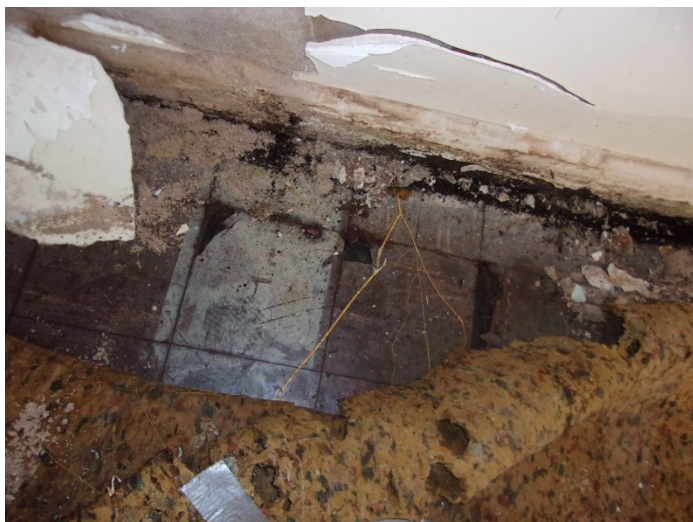
Photo 11 – 9" x 9" black floor tile & black mastic in the left big room under carpet
