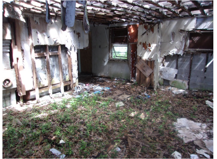
Photo 14 – View of right room with the damaged ceiling & missing lining/roof & large amount of leaf litter on floor
