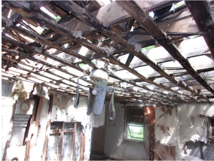
Photo 13 – View of right room with the damaged ceiling & missing lining/roof
