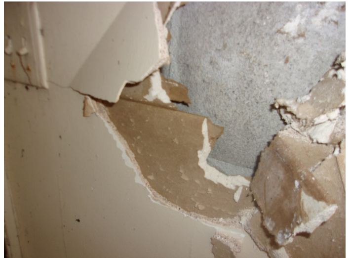
Photo 8 – Unfinished drywall beneath the plaster walls throughout
