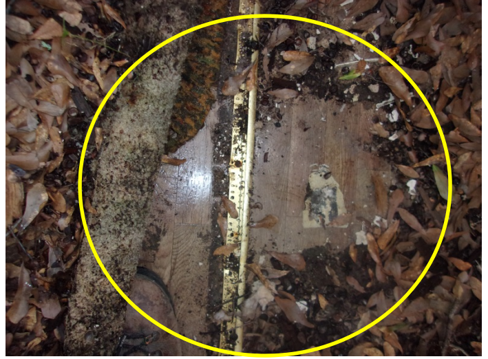
Photo 12 – Wooden plank pattern vinyl floor & mastic in the kitchen landing, bathroom, right big room under carpet & front door entry
