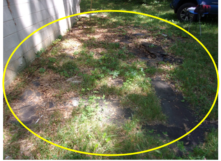
Photo 6 – Roll roof shingles & built-up roofing debris pile on the ground to the right side of the front of the house
