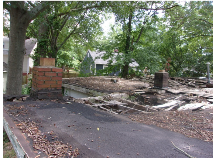
Photo 4 – Tar on 2 chimney's & 4 vents & roll roof shingles with felt & tar on the house roof
