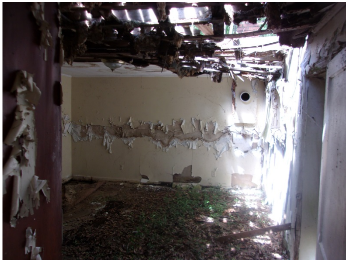
Photo 15 – View of the left room with the damaged & collapsed ceiling/roof & large amount of leaf litter on floor
