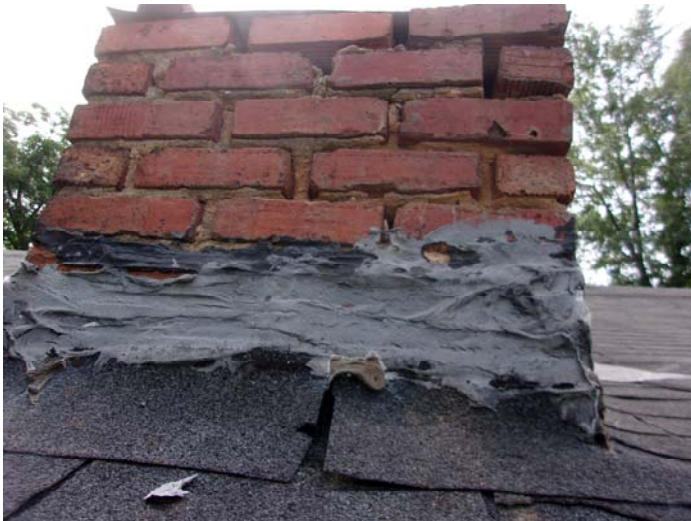
Photo 3 – Chimney with tar
