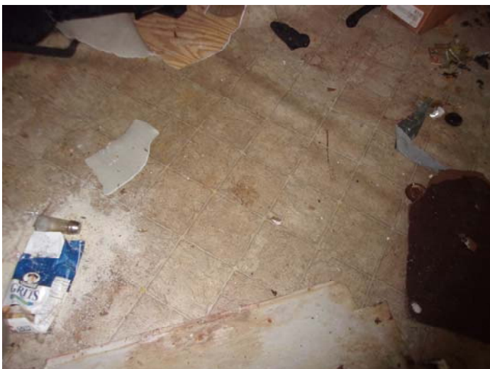
Photo 11 – Tan square pattern vinyl floor with no mastic in the kitchen
