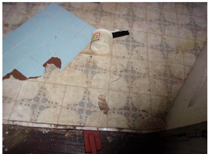
Photo 12 – Tan square & blue flower pattern vinyl floor & mastic in the bathroom
