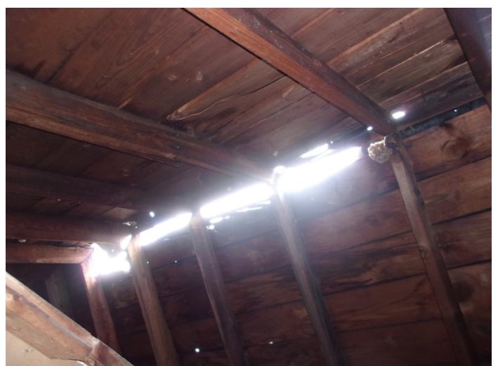
Photo 24 – View of damage to roof & ceiling
