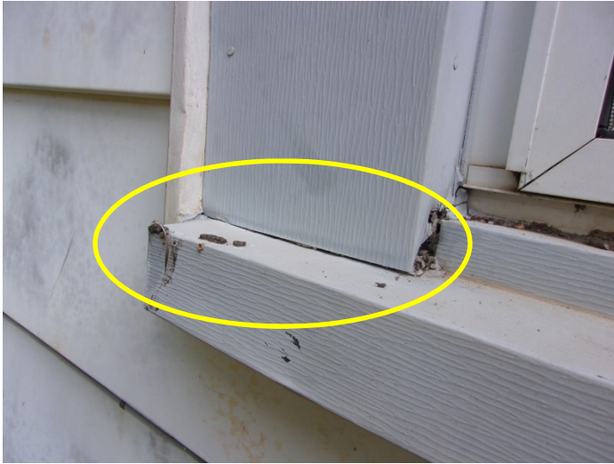
Photo 7 – Gray caulk on the metal wrapping over window casings
