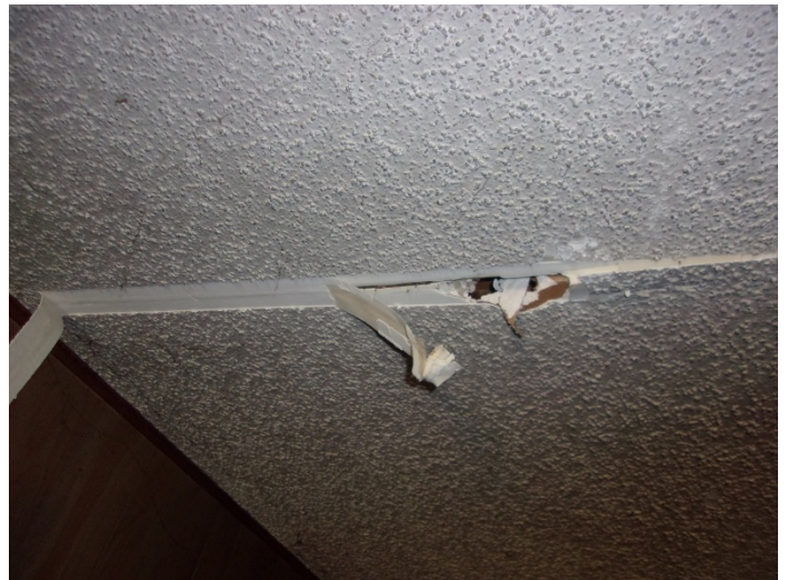
Photo 12 – Drywall with joint compound & tape throughout 1 st floor ceilings; 1 st floor back hallway & bathroom walls & ceilings; 2 nd floor front bedroom ceiling
