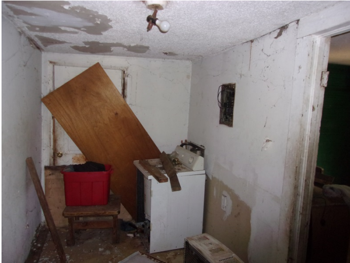
Photo 13 – Drywall with joint compound & tape throughout 1st floor ceilings; 1st floor back hallway & bathroom walls & ceilings; 2nd floor front bedroom ceiling
