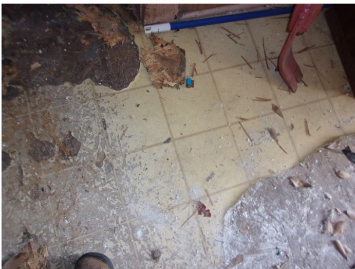
Photo 15 – Yellow medium square pattern vinyl floor & mastic in the front hallway
