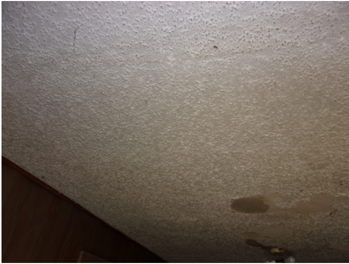
Photo 9 – Popcorn ceiling texture throughout 1 st floor except in bathroom
