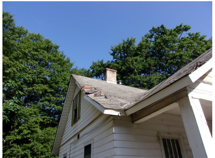
Photo 4 – Chimney with tar – assumed positive
