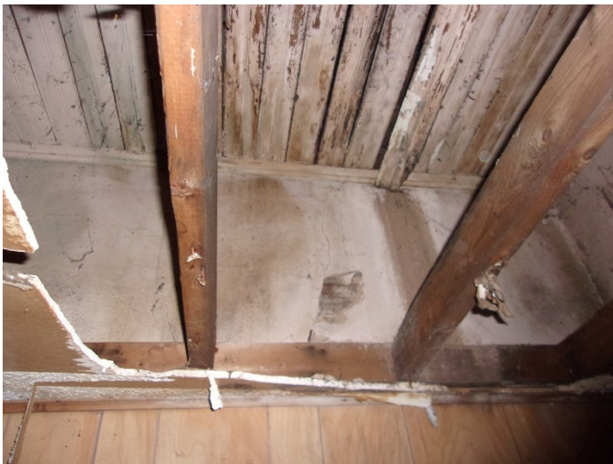
Photo 11 – Plaster with no finish throughout the 1 st floor
