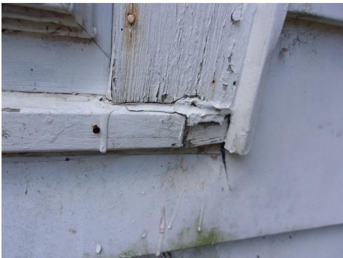
Photo 5 – White caulk on wooden window casing with no metal wrapping
