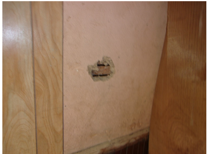
Photo 10 – Plaster with no finish throughout the 1 st floor
