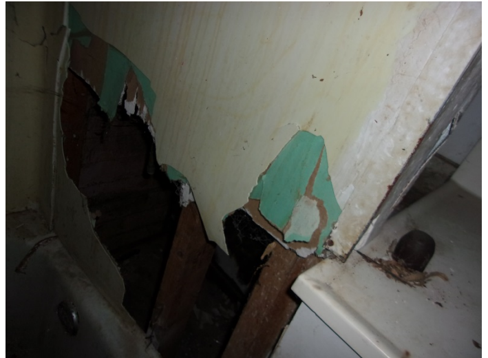
Photo 14 – Mastic beneath bathtub surround in the bathroom
