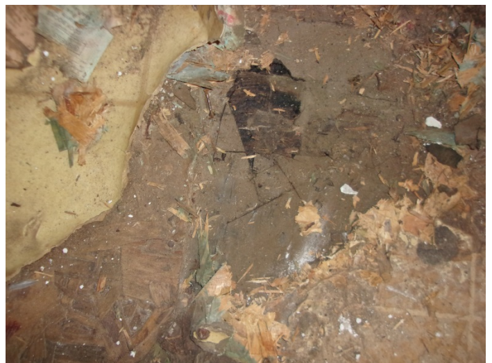
Photo 16 – Black vinyl floor & mastic in the front hallway under wood
