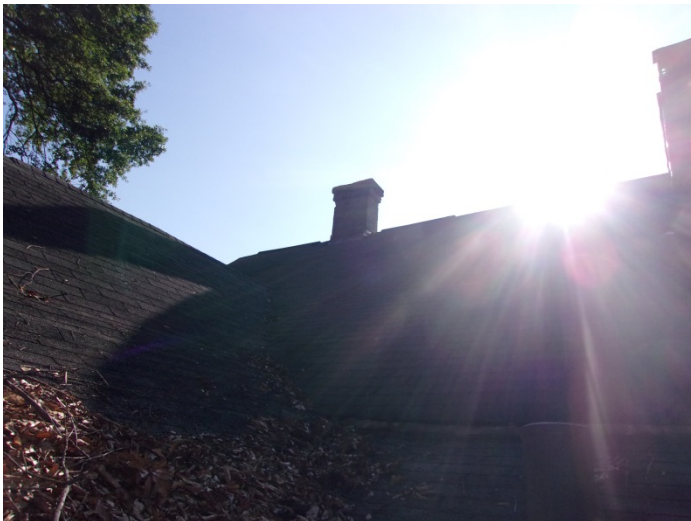
Photo 3 – Chimney with tar – assumed positive
