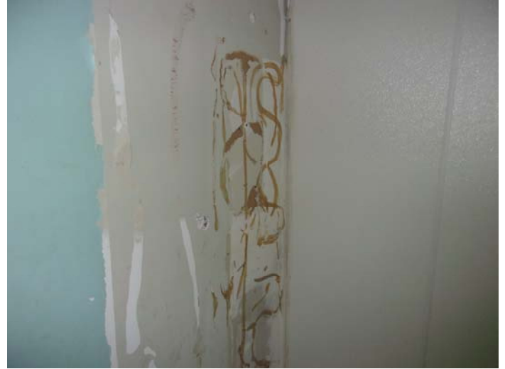
Photo 14 – Mastic under tub/shower surround in the main level - bathroom
