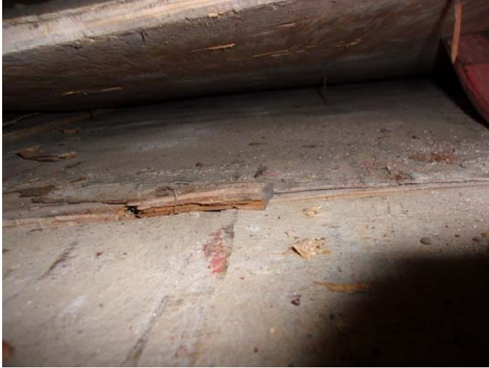
Photo 13 – Dark flooring with no mastic in the main level – kitchen under wood
