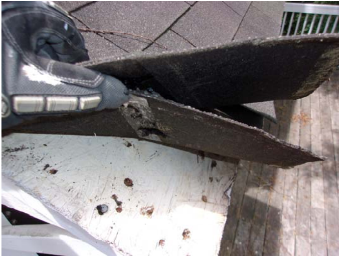
Photo 3 – Roof shingles & no felt on the front door awning
