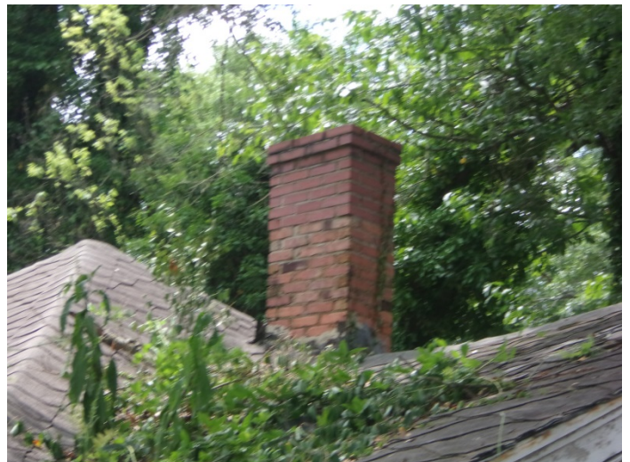
Photo 6 – Chimney tar on 1 of 2 chimneys
