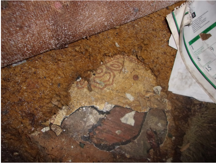
Photo 13 – Orange pattern vinyl floor & mastic over brown vinyl floor with felt backing in the dining room (1st & 2nd layers)
