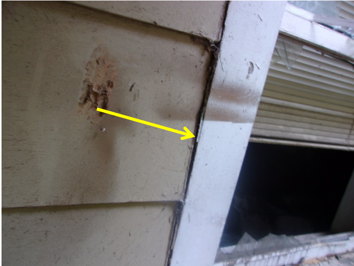
Photo 9 – Window caulk on the wooden casings
