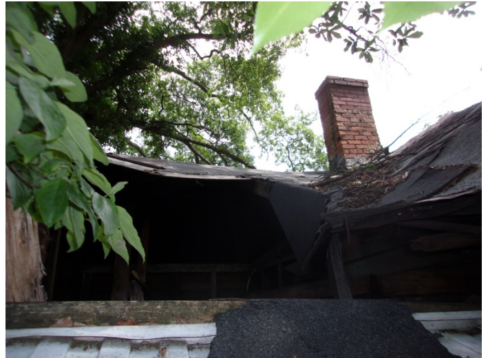
Photo 4 – Roll roofing & felt on the front porch roof & adjacent area & back portion of the house roof
