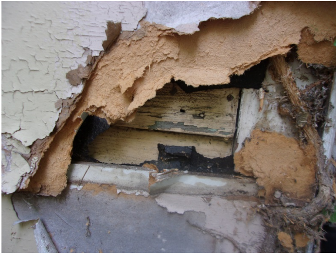
Photo 7 – Felt paper beneath wooden pressboard siding
