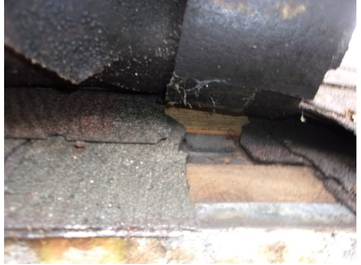
Photo 2 – Roof shingles & no felt on the roof
