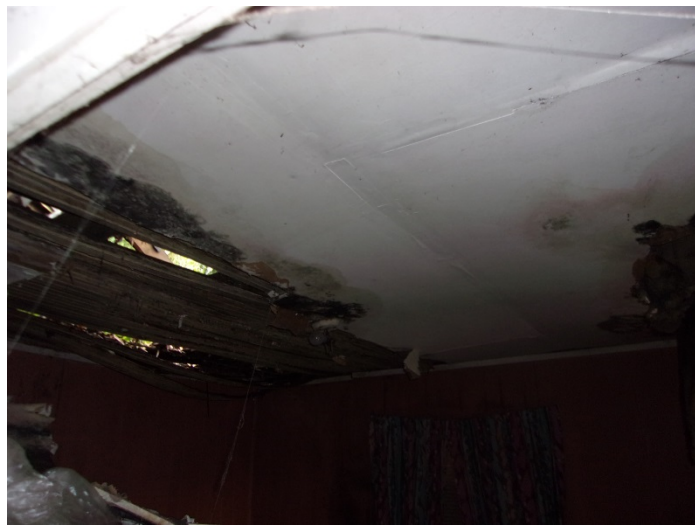
Photo 19 – Typical view of unstable & collapsed ceiling
