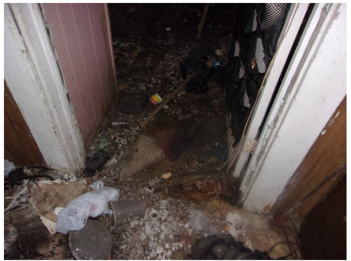
Photo 20 – Typical view of unstable & collapsed flooring
