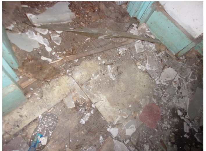
Photo 16 – Grey square pattern vinyl floor & mastic in the bathroom hallway (partially under wood)
