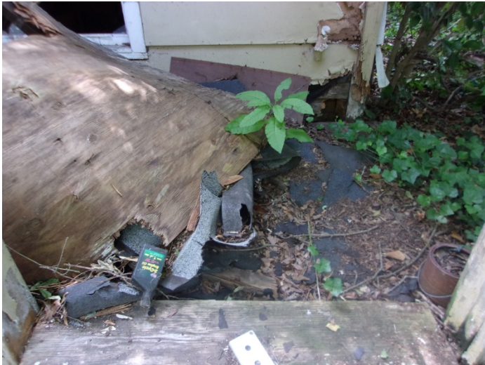
Photo 3 – Roll roofing & felt on the front porch roof & adjacent area & back portion of the house roof
