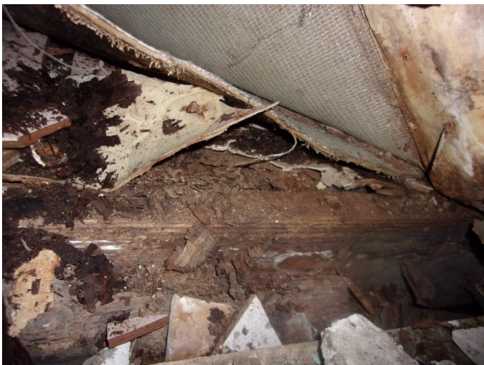
Photo 17 – White pattern vinyl floor with no mastic in the bathroom under carpet
