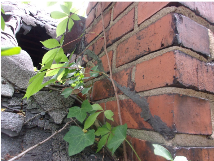
Photo 5 – Chimney tar on 1 of 2 chimneys
