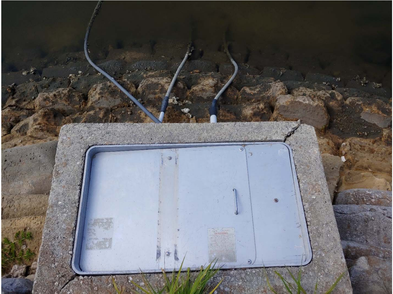
Pull box with power and fiber for the credit card machine on the floating dock.
