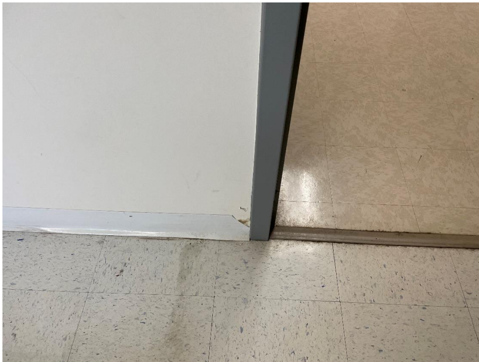
Photograph 6: View of floor at clerk office doorway.
