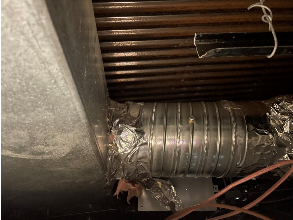
Photograph 7: View of the roll board connected to the furnace.
