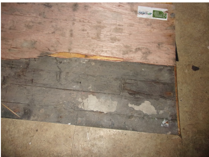
Photo 11 – felt paper in the kitchen under wood.
