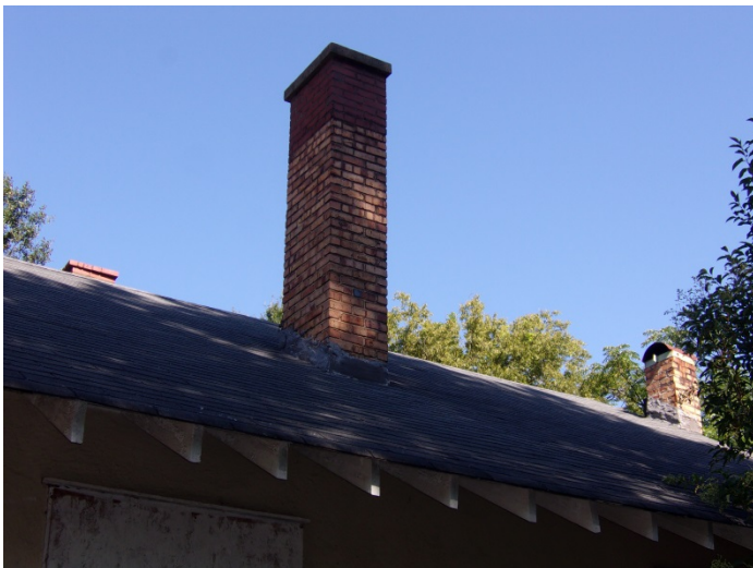
Photo 5 – Mastic on 2 chimneys assumed positive.
