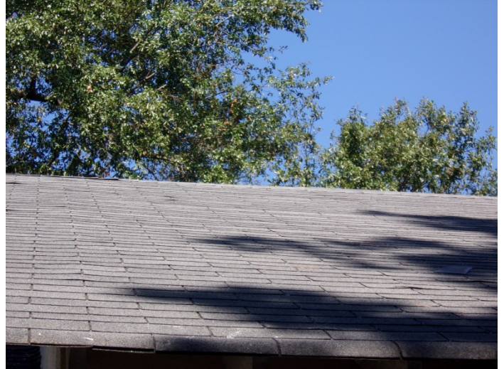
Photo 2 – Roof shingles and no felt.
