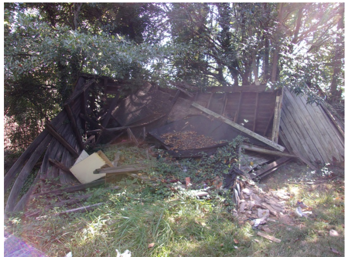
Photo 4 – Collapsed exterior shed with roofing materials.
