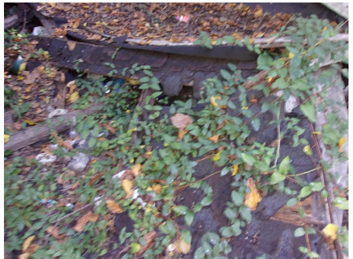
Photo 6 – Collapsed exterior shed with roofing materials.
