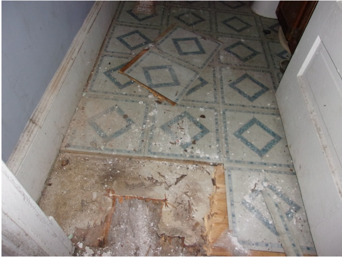
Photo 13 – 12" x 12" blue self-stick floor tile with mastic (top layer over wood) over beige vinyl flooring with mastic 2 nd layer under wood) in the bathroom.
