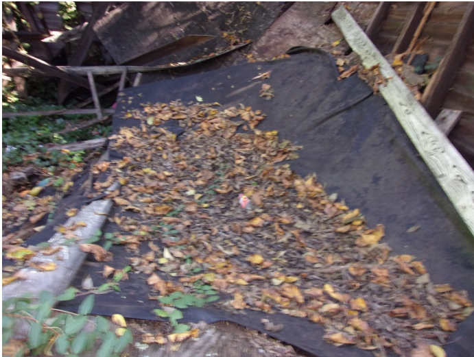
Photo 7 – Collapsed exterior shed with roofing materials.
