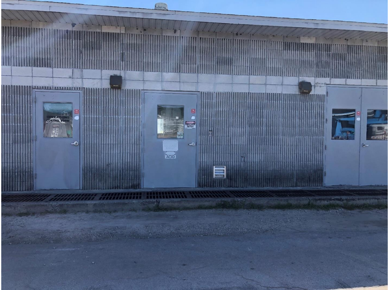
Figure 1UV-UPS Front Entrance
