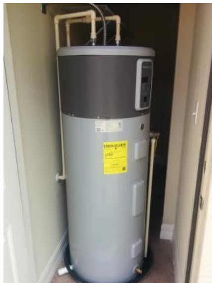
Electric Storage Tank
