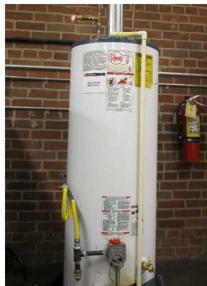
Gas Storage Tank
