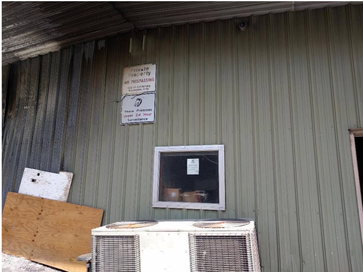
Picture of window with LBP on frame
