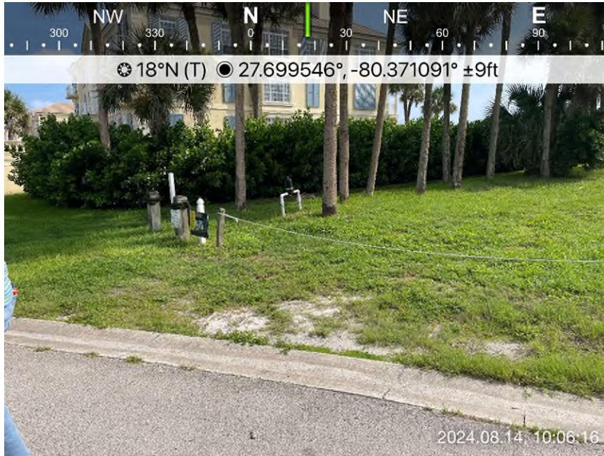
Photo 2. Taken from Sea Court looking north at 1 Sea Court and pedestrian access. Note the above grade irrigation plumbing.
