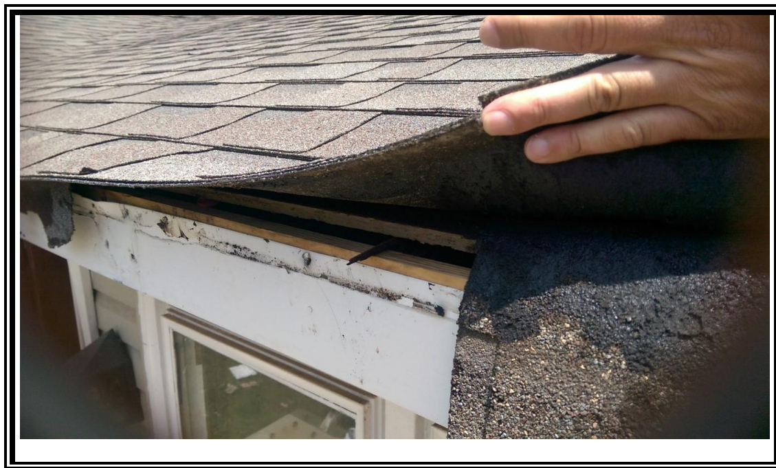
3. View of the shingle and felt paper on the roof of 880 California Blvd.
