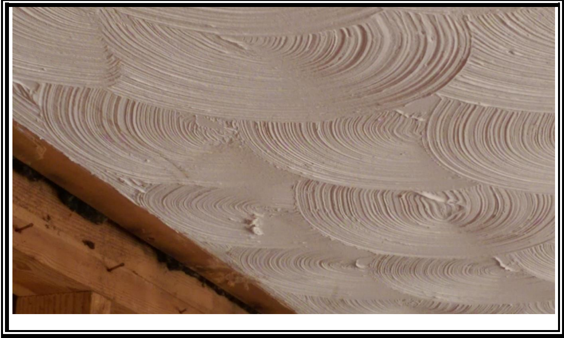
5. View of the ceiling texture in the living room and kitchen of 880 California Blvd.
