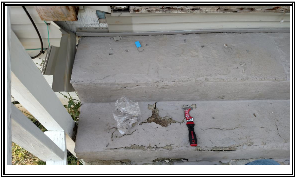
2. View of the lead-paint sample on the rear stairs of 880 California Blvd.
