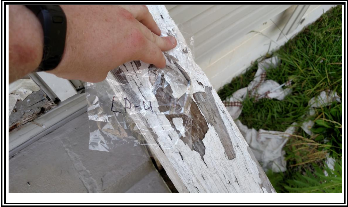
1. View of the lead-paint sample on the rear stair railing of 880 California Blvd.
