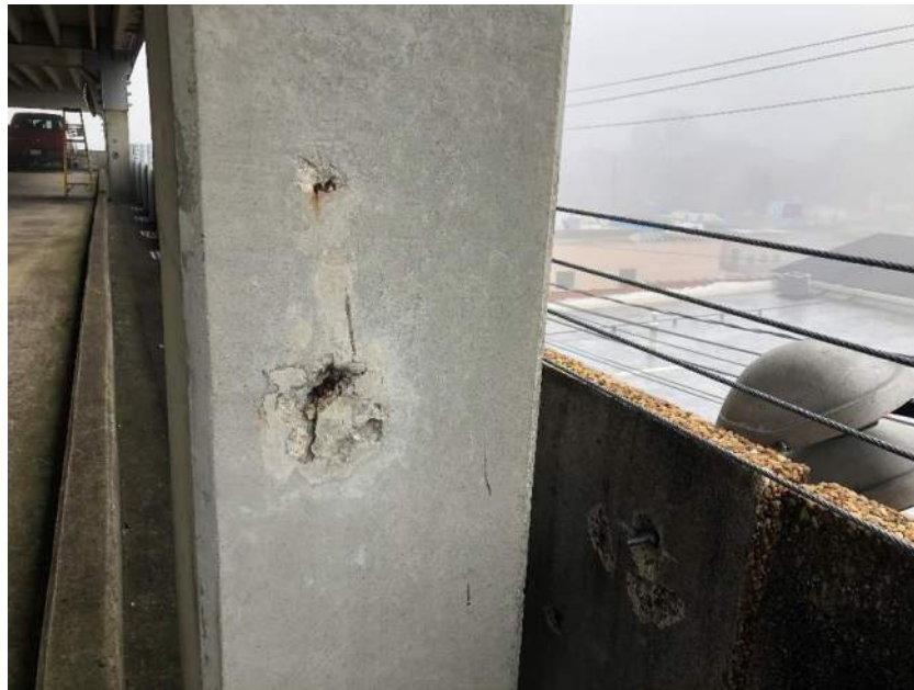
Photo 5A Column Spalling Concrete
