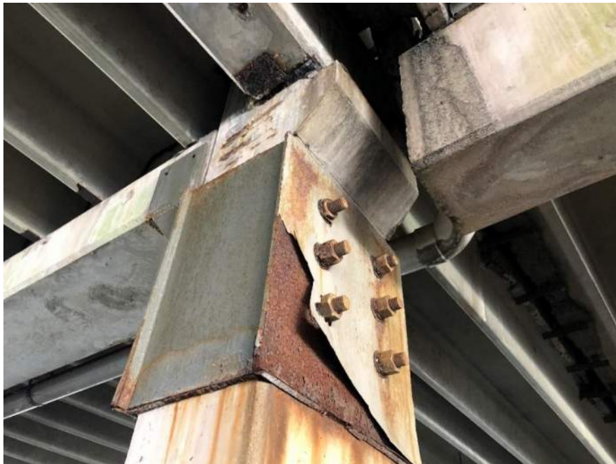
Photo 6A Paint Exposed Steel Reinforcements (Competed by Others)
