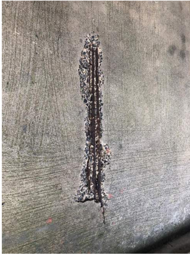
Photo 5B Spalling Deck
