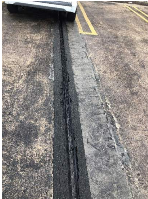
Photo 1 Existing Expansion Joints to be Completely Removed and Rebuilt
