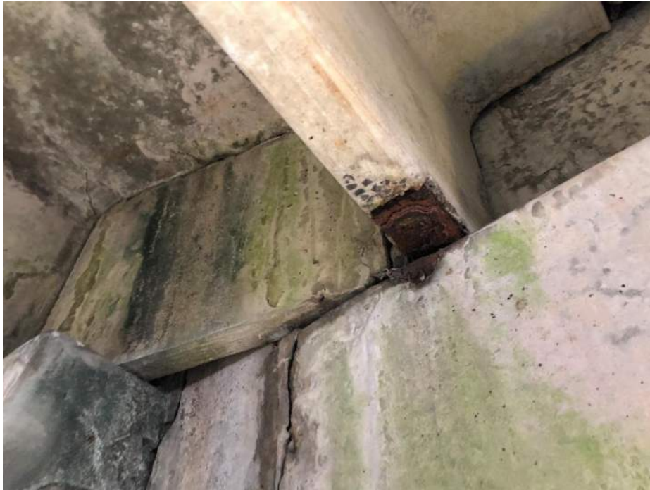
Photo 6 Paint Exposed Steel Shimes
