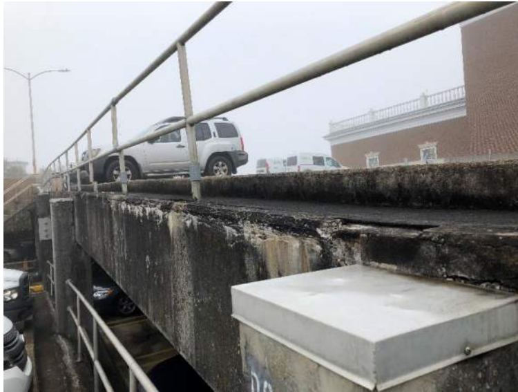
Photo 4 Top Concrete that need to be sealed
