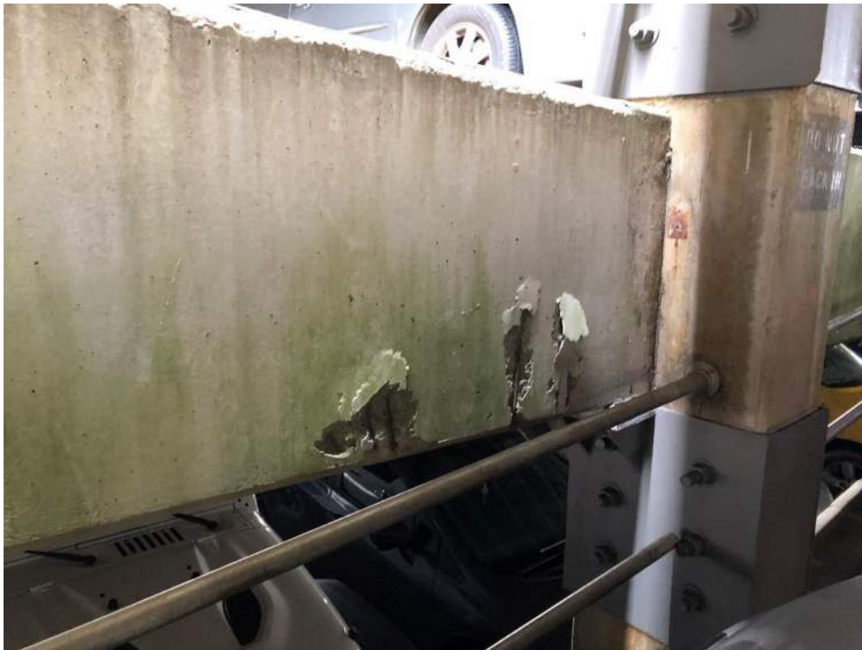
Photo 2A Aluminum Handrail and Spalling Concrete
