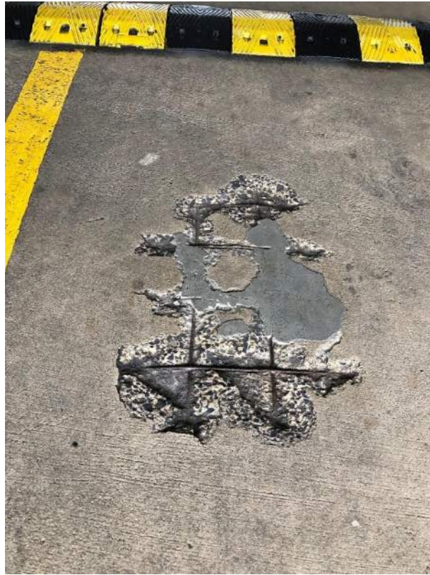
Photo 5 Deck Spalling Concrete
