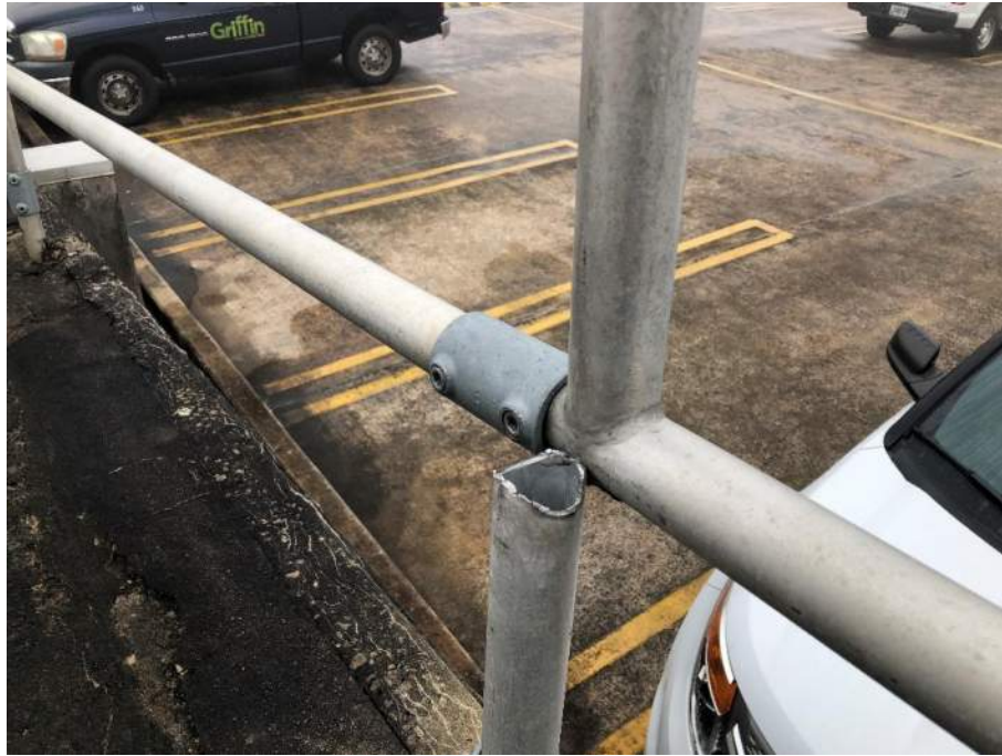
Photo 2 Existing Aluminum Handrail to be Repaired
