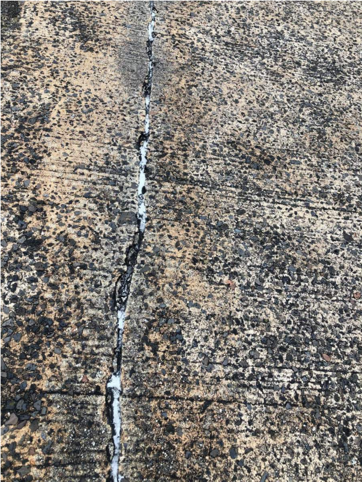
Photo 3 Crack in need of Recaulking
