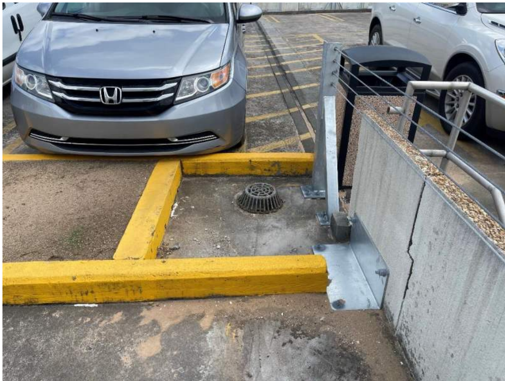
Photo No. 2: Area drain isolated by concrete curbing at southeast corner of Level 4A
