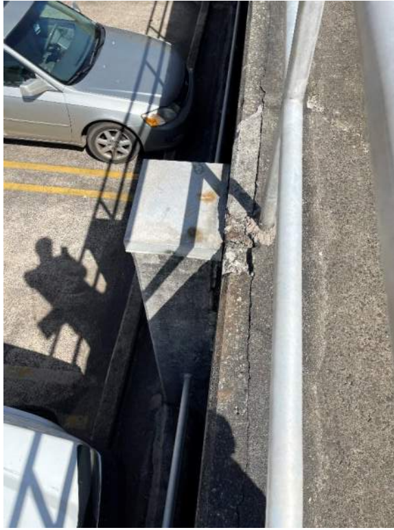
Photo No. 31: Spalled/failing concrete at guardrail post
