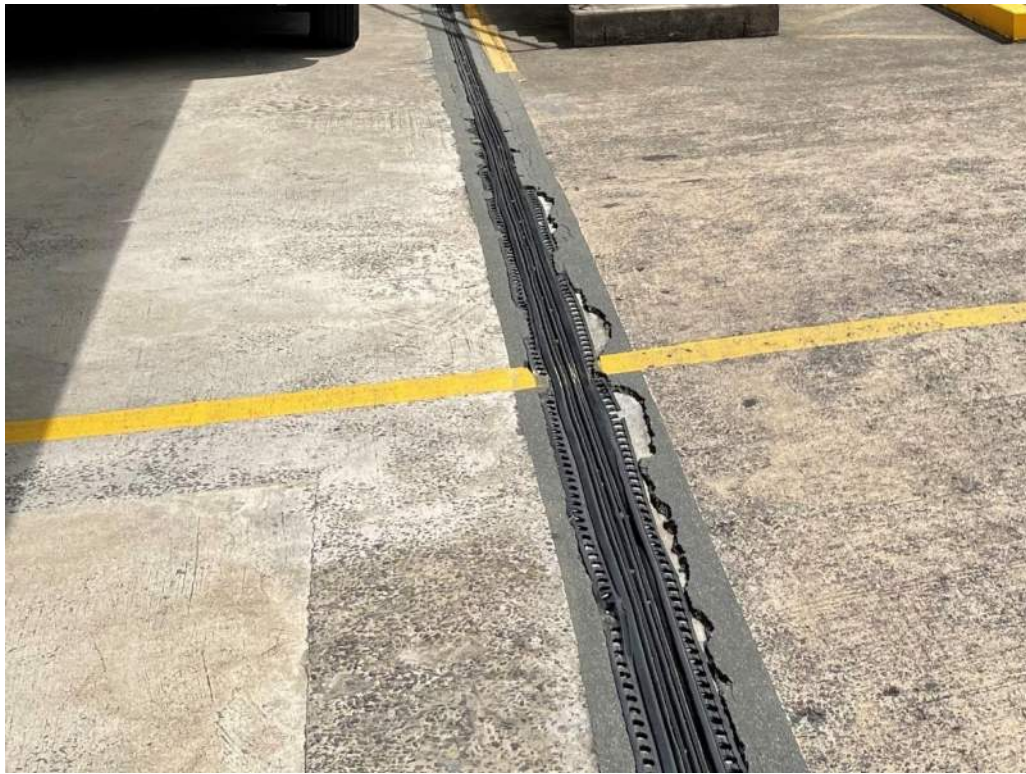
Photo No. 25: Typical failed expansion joint – Level 3A shown
