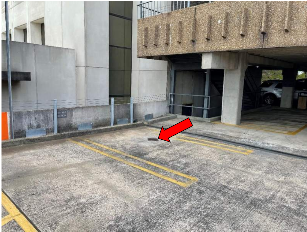
Photo No. 9: Area drain near northwest corner of ramp at Level 3A
