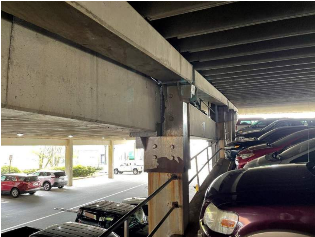
Photo No. 24: Corroded bracket supporting Level 2 framing at gridline 2-F
