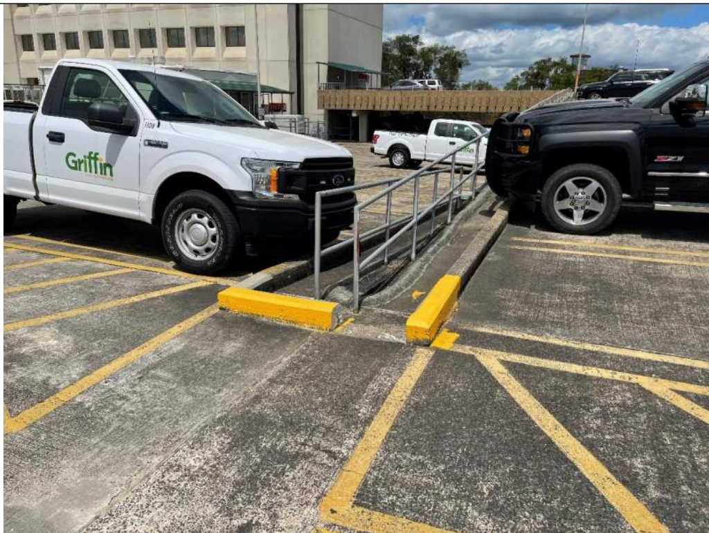
Photo No. 6: Concrete curbing/wheel stop at Level 3 near grid line J-2 – note section of curbing previously cut out and addition of concrete at edge of ramps
