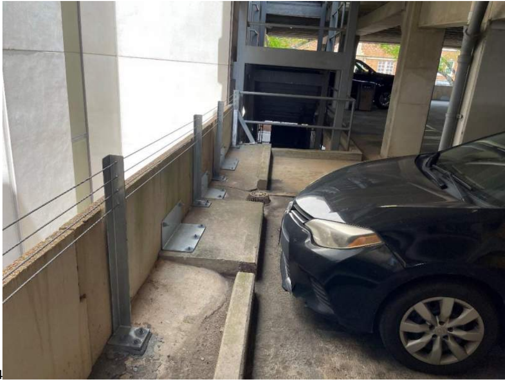
4 Photo No. 19: Partially isolated area drain at Level 2A west of column at gridline D-1
