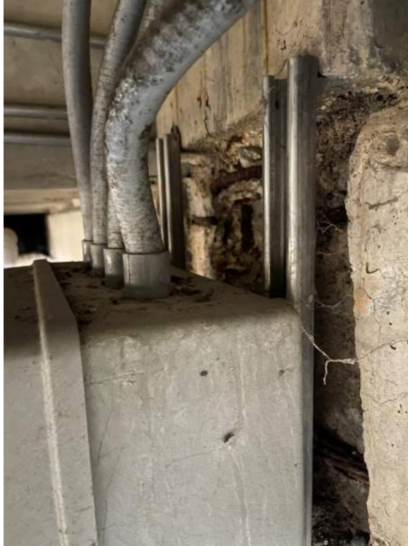
Photo No. 28: Spalled concrete on west face of concrete column at gridline 1-E below Level 1A
