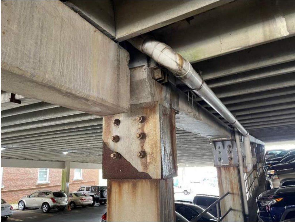
Photo No. 23: Corroded bracket supporting Level 2 framing at gridline 2-D
