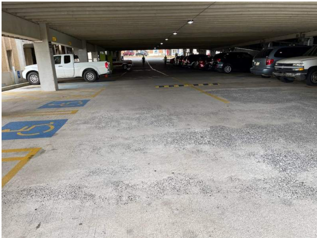
Photo No. 22: Level 1A ramp – view facing north toward on-grade portion of deck structure
