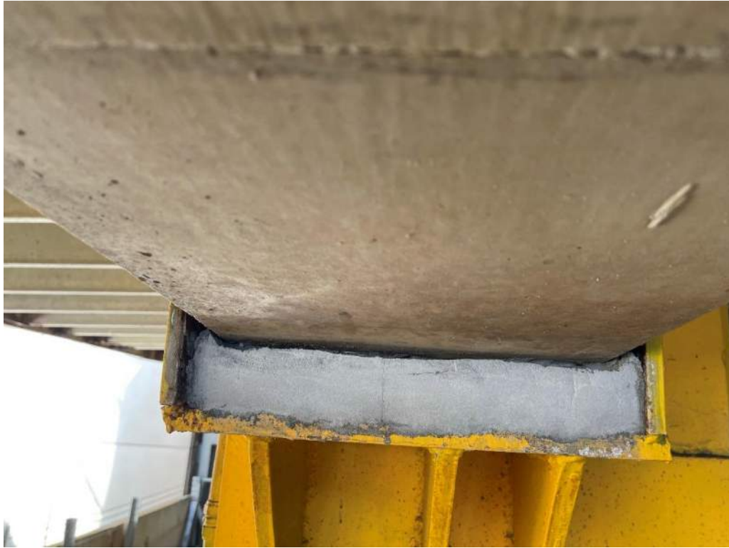
Photo No. 29: Gap at recently grouted steel bracket
