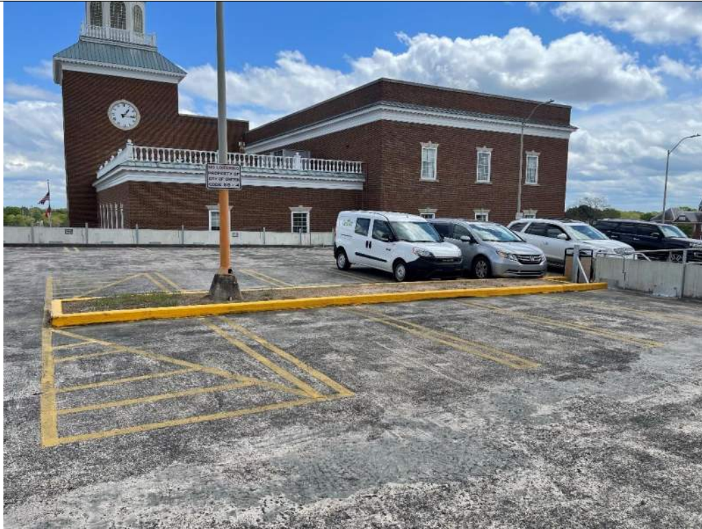
Photo No. 1: Overview of Level 4A and north end of Level 3B – note concrete curbing and island
