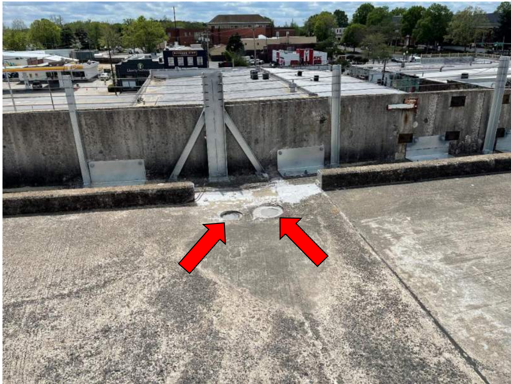
Photo No. 8: Existing (right) and newly installed drains at Level 3 near gridline K-2
