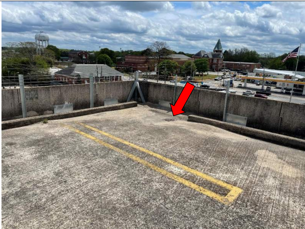
Photo No. 4: Area drain at southeast corner of Level 3B reported to have been recently cleared of sandy, granular debris
