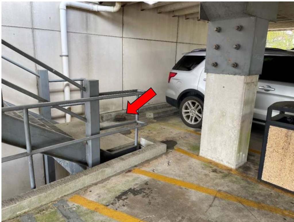
Photo No. 12: Partially isolated area drain at level 3A west of column at gridline B1
