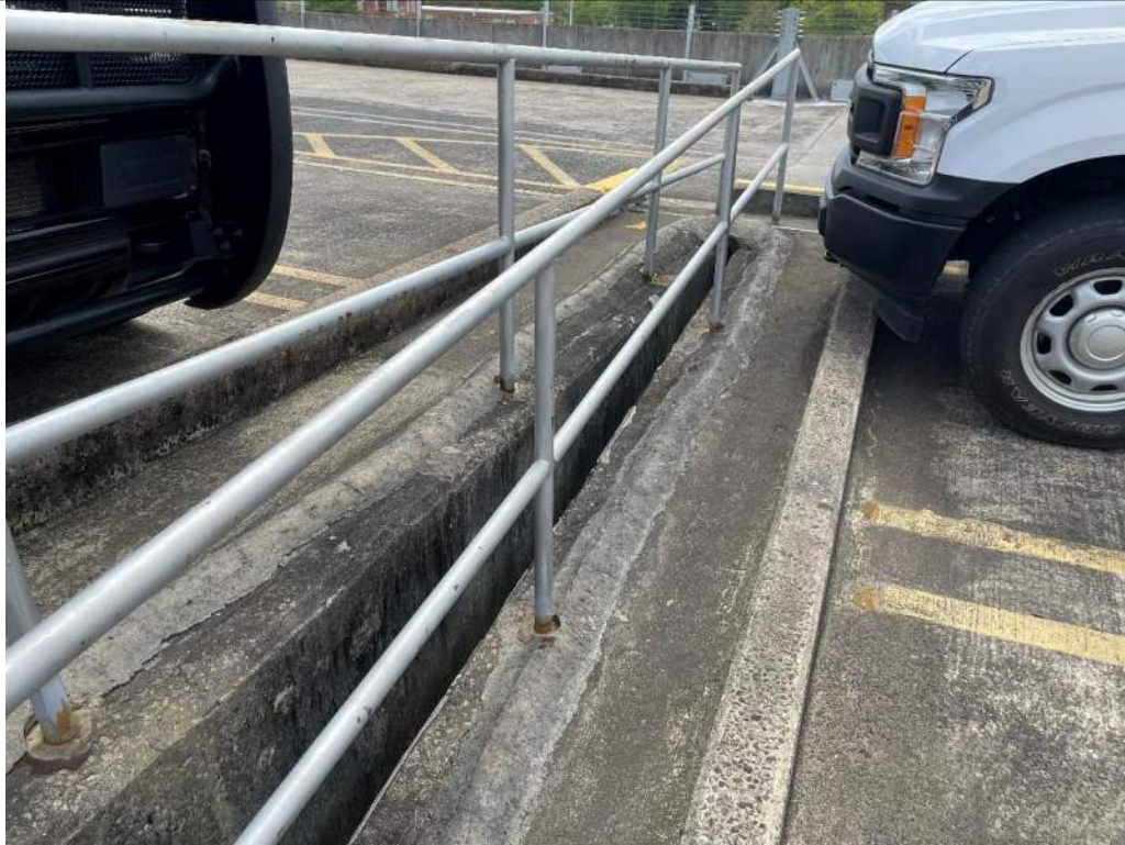
Photo No. 7: Alternate view of concrete added at edges of Level 3 ramps shown in Photo 6 above
