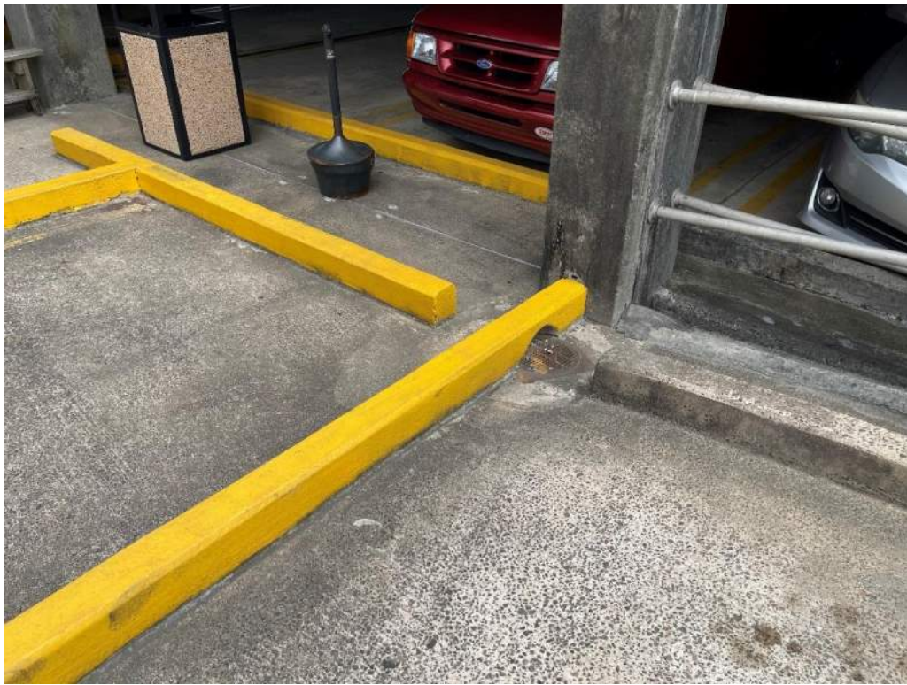
Photo No. 11: Partially isolated area drain at location shown in Photo 10 above
