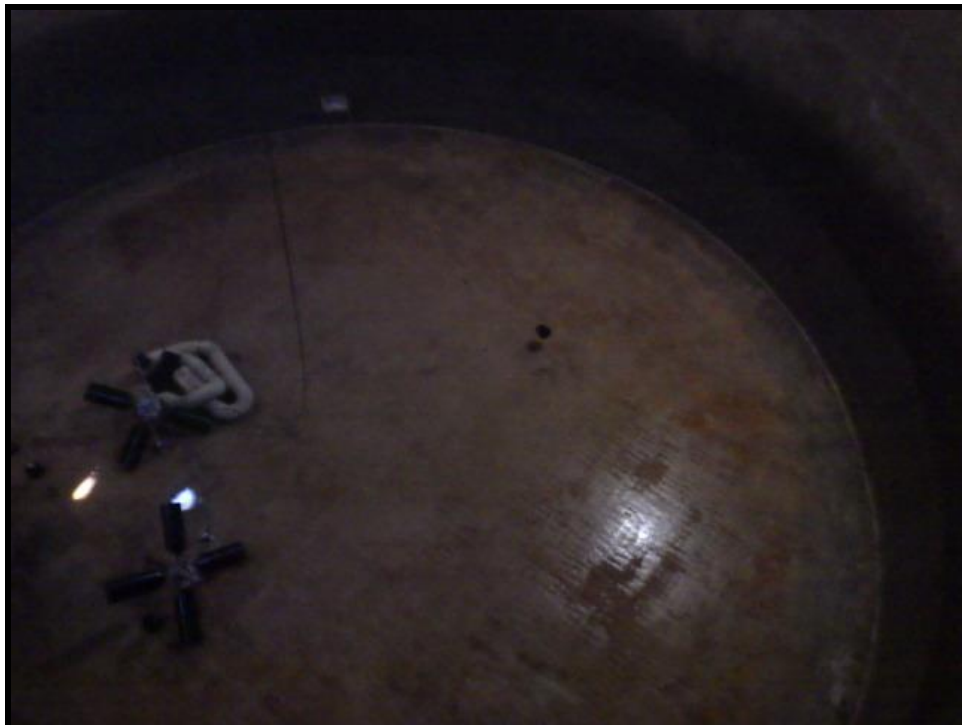
Photo 21. Interior – After Washout
