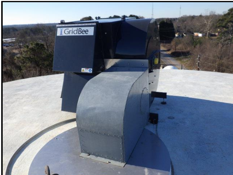
Photo 7. Powered vent system
