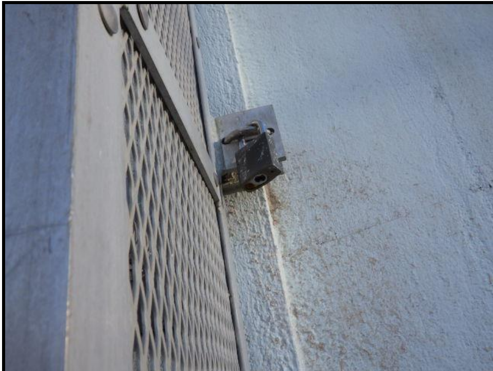
Photo 23. Ladder Gate Locked
