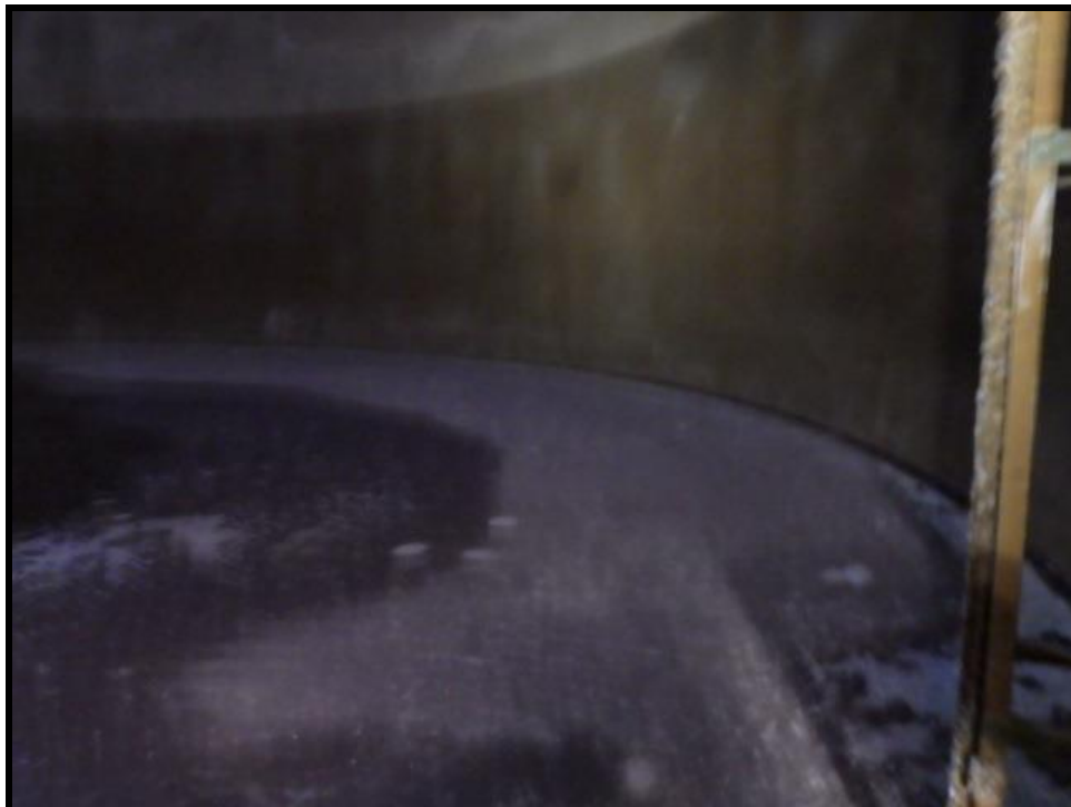
Photo 11. Interior ladder and sediment on floor before washout
