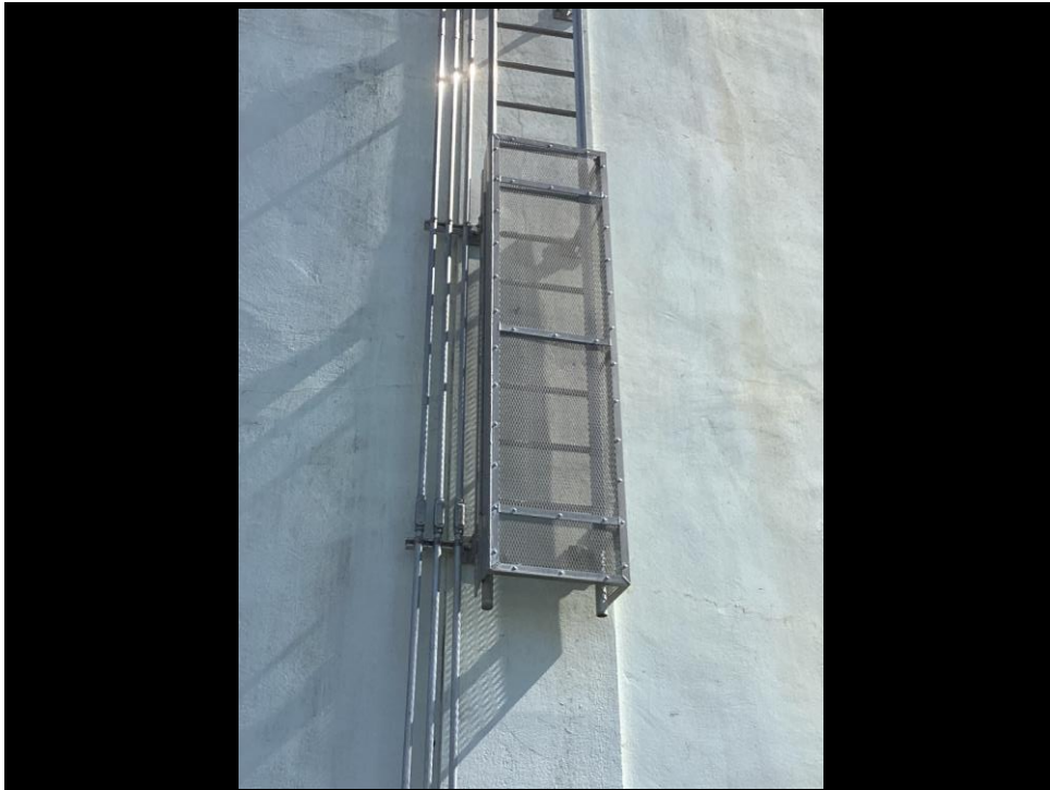
Photo 23. Ladder Gate Locked
