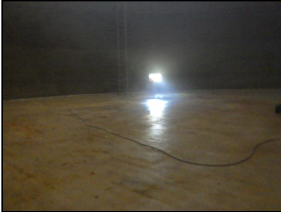
Photo 18. Interior – After Washout
