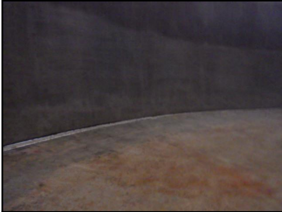
Photo 20. Interior – After Washout
