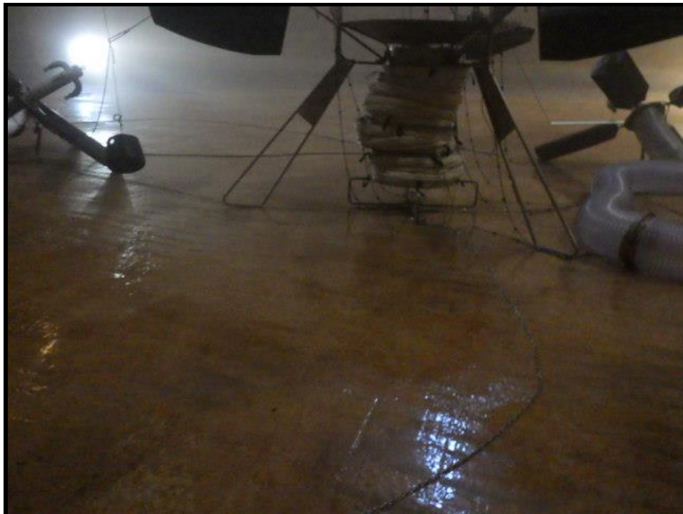
Photo 17. Interior after washout
