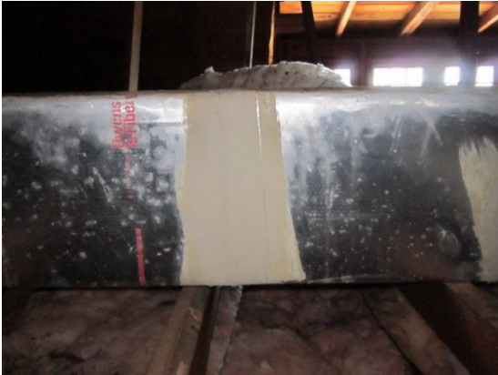
Photo #7 Gray mastic reported to be ACM.
