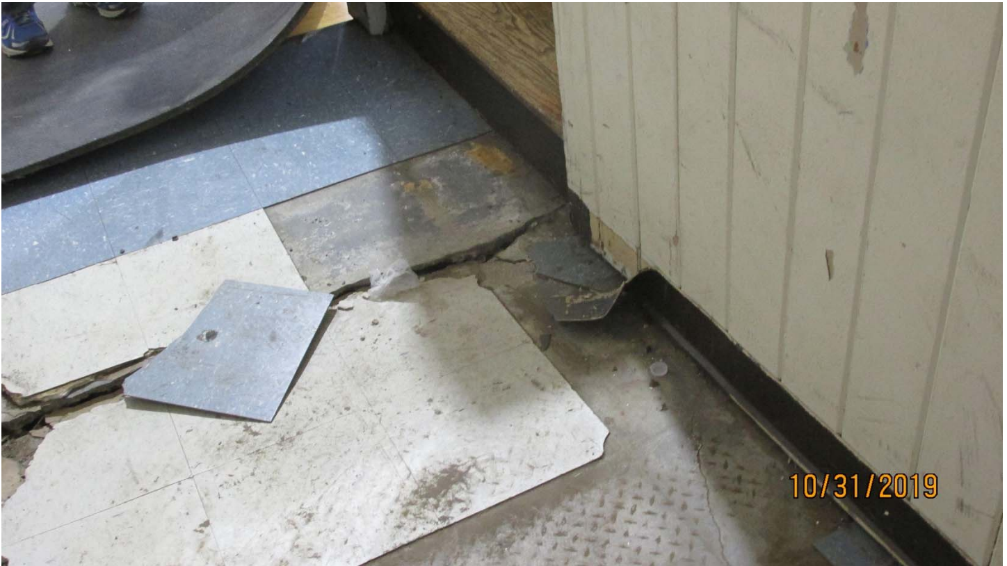
Picture #12: Concrete floor in bleacher area subsidence (DL-3)
