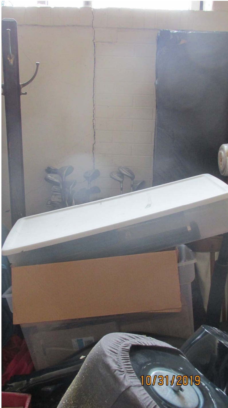
Picture #16: Cracks in Exterior Brick Wall – South End of Gymnasium underneath bleachers (DL-3)
