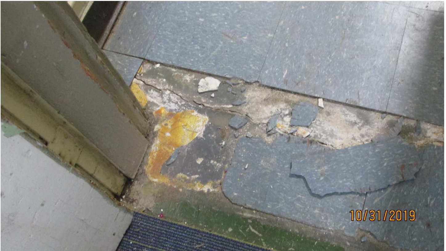
Picture #13: Concrete floor in bleacher area subsidence (DL-3)
