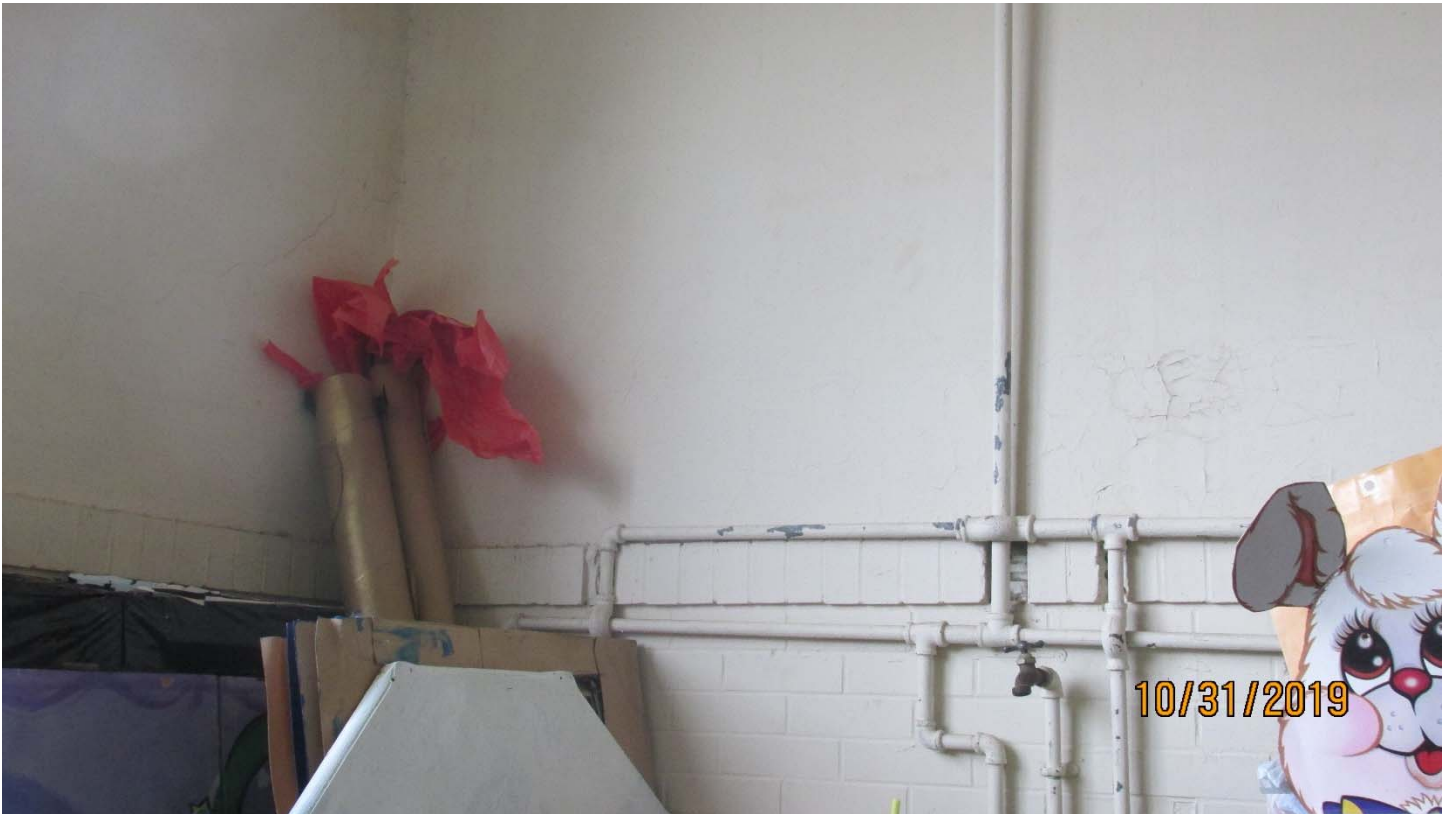
Picture #18: Cracks in Exterior Brick Wall – South End of Gymnasium underneath bleachers (DL-3)
