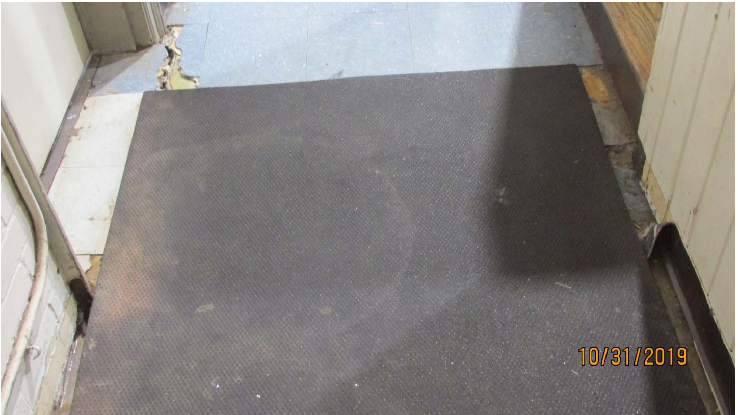
Picture #09: Concrete floor in bleacher area subsidence (DL-3)
