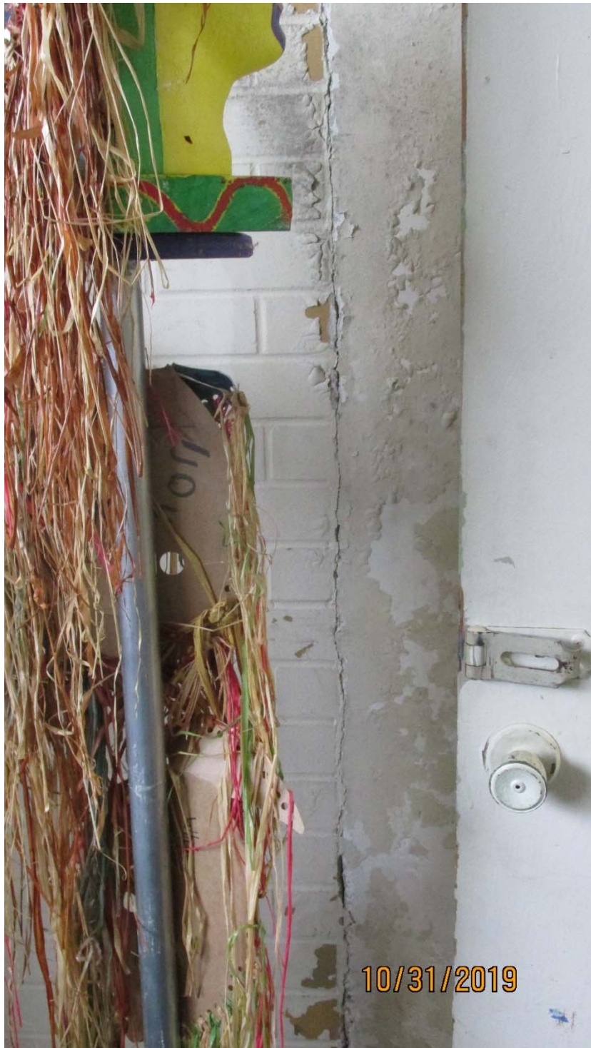
Picture #15: Cracks in Exterior Brick Wall – South End of Gymnasium underneath bleachers (DL-3)
