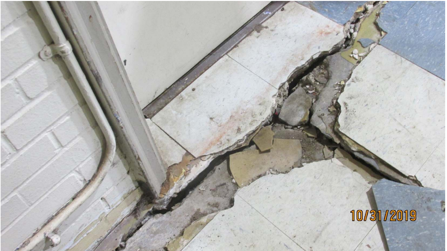
Picture #10: Concrete floor in bleacher area subsidence (DL-3)
