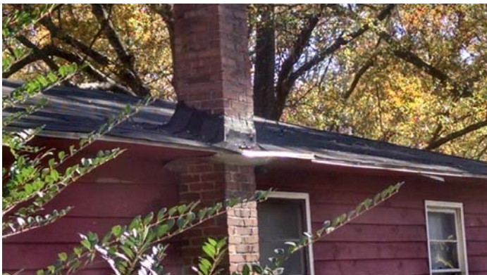
Photo 5 – One chimney with tar assumed. Two layers of roofing shingles and one layer of felt on the roof.
