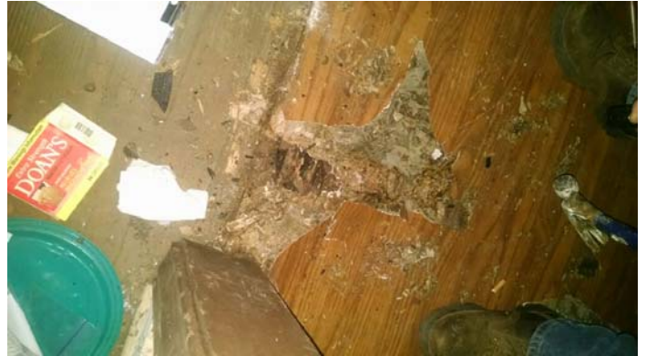
Photo 2 – Flooring under roll wood pattern vinyl and layer of sub-floor in kitchen.
