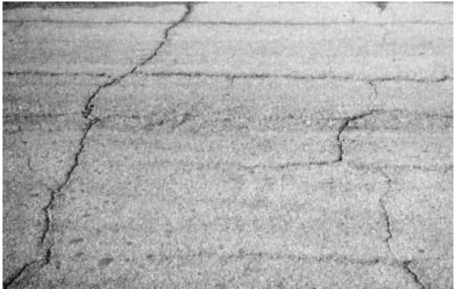
▶ Intermediate-size block cracking, 1'-5' across with open cracks.
