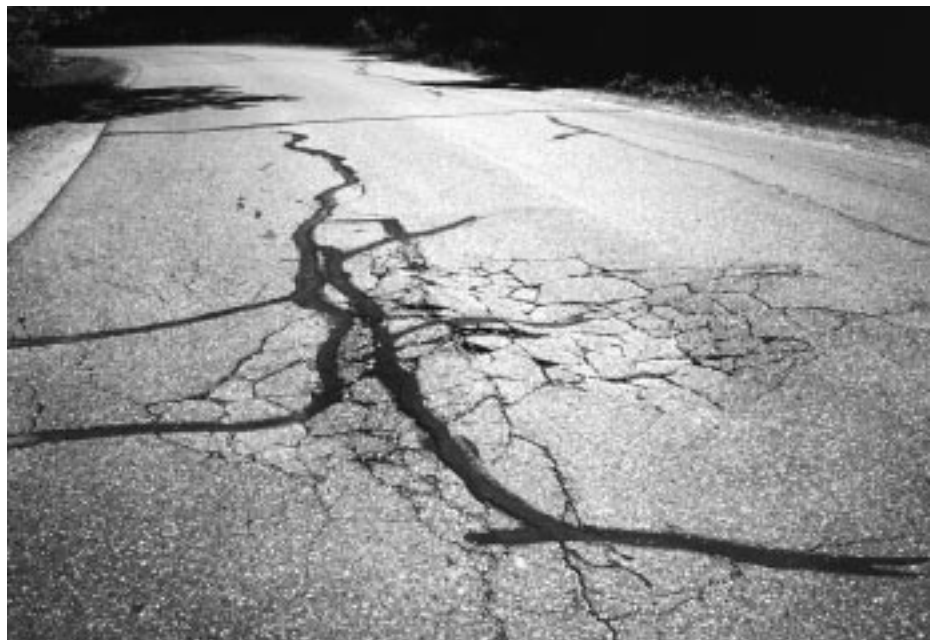
► Frost heave damage from spring break-up.
