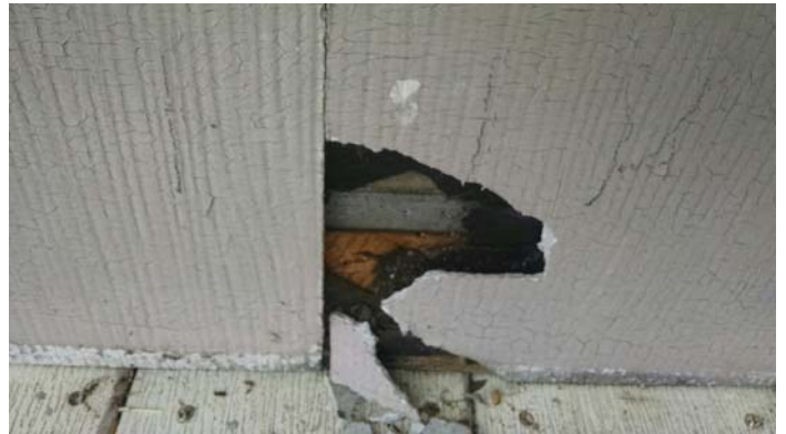
Photo 4 – Cement board siding with felt behind.
