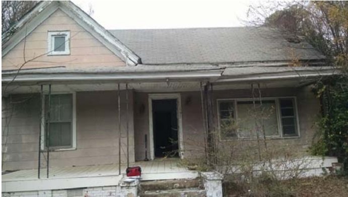
Photo 1 – 592 Farley Avenue with two layers of shingles and no felt on the roof.
