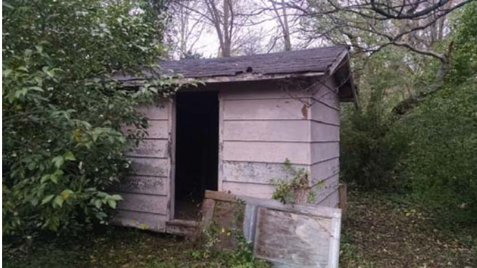
Photo 7 – Exterior shed with two layers of shingles and one layer of felt.
