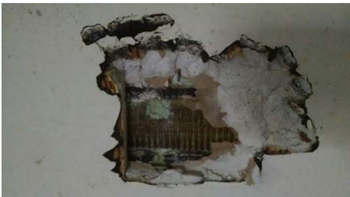
Photo 11 – Kitchen drywall with mastic.
