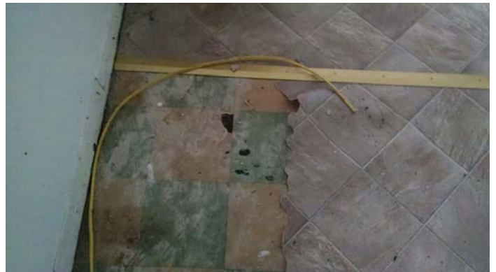
Photo 12 – Tan roll vinyl over 9"x9" green and yellow pattern flooring in the bathroom
