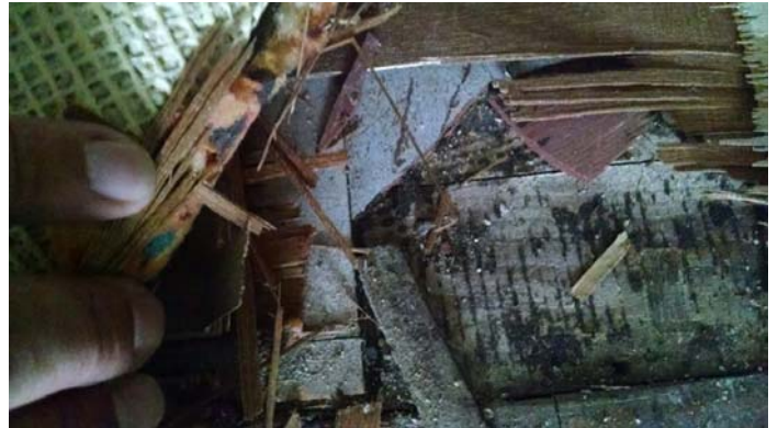
Photo 10 – Flooring and mastic under carpet and layer of subfloor between living room and hall outside bathroom.
