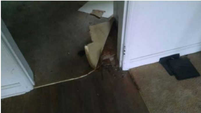
Photo 9 – Flooring and mastic under carpet and layer of subfloor between living room and hall outside bathroom.
