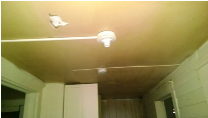
Photo 9 – Drywall with joint compound & no tape in the pantry & living room.
