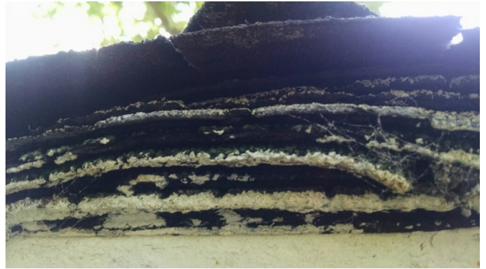
Photo 2 – 6 layers of roof shingles with no felt.
