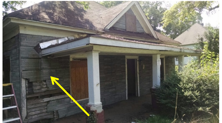
Photo 4 – Asphalt siding over wooden siding.
