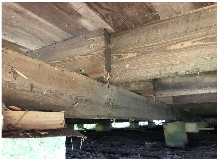
Picture showing joists to beam connection and beam to beam scenario over CMU pier
