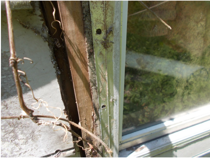
Photo 7 – Putty/Caulk on exterior shed window casing.
