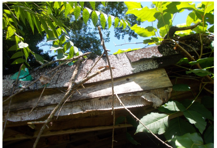
Photo 6 – Roll roofing (1 layer) and no felt on exterior shed roof addition.
