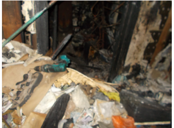
Photo 14 – Fire/structural damaged interior of house and debris piles.
