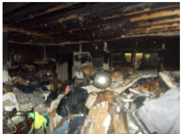
Photo 12 – Fire/structural damaged interior of house and debris piles.
