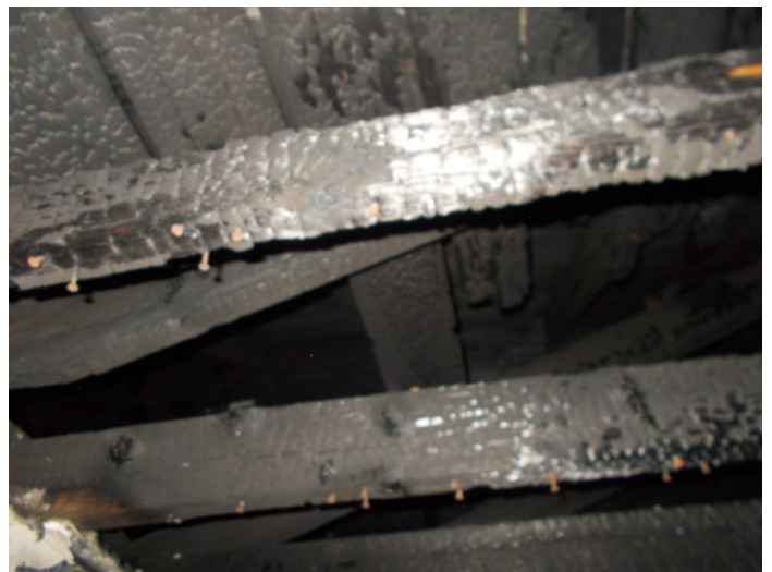
Photo 16 – Fire/structural damaged interior of house and debris piles.
