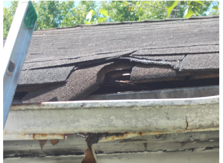
Photo 8 – Roofing shingles (5 layers) and no felt on main house roof.
