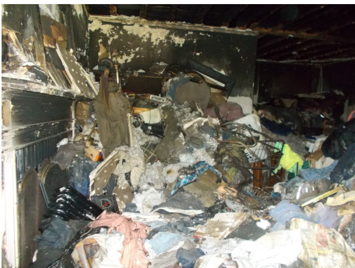
Photo 11 – Fire/structural damaged interior of house and debris piles.
