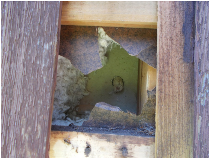
Photo 9 – Siding paper beneath framing studs.
