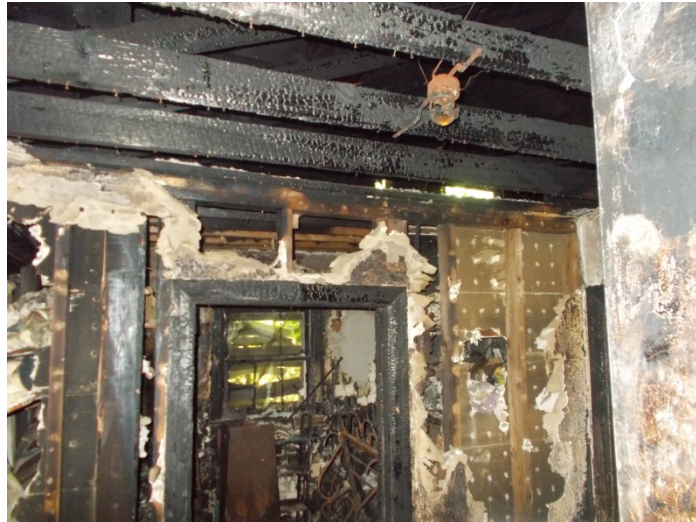
Photo 13 – Fire/structural damaged interior of house and debris piles.
