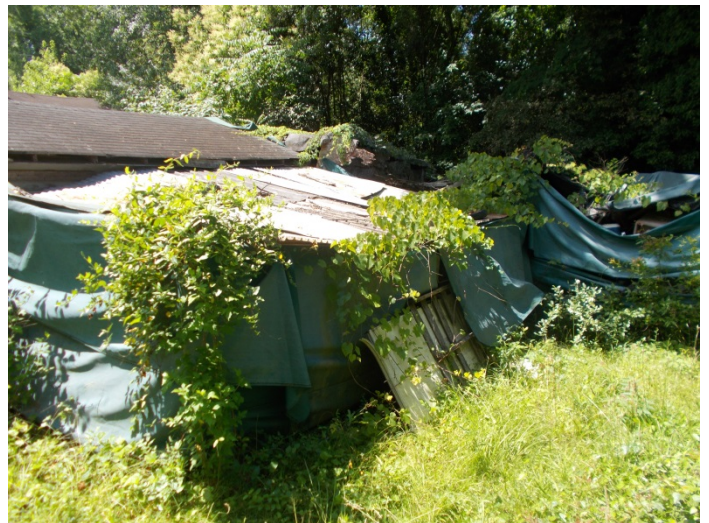
Photo 4 – Debris stacked behind shed.
