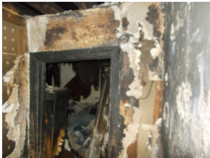
Photo 15 – Fire/structural damaged interior of house and debris piles.
