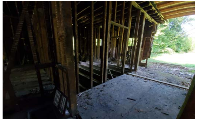
Photo 10 – Missing floor back left area of structure.
