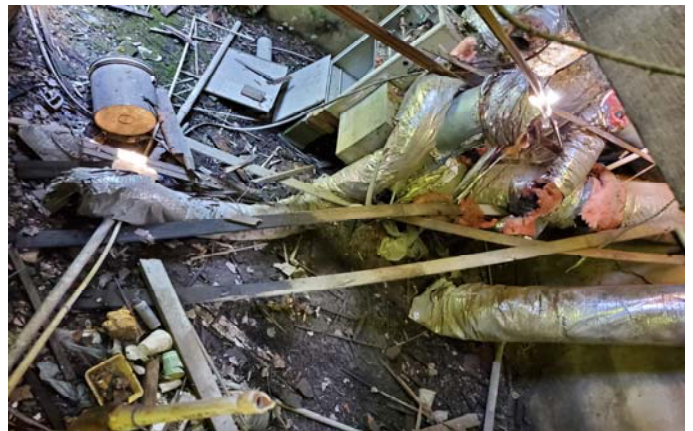
Photo 12 – Debris scattered in back crawl space.
