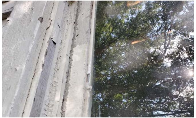
Photo 4 – Exterior window caulk.
