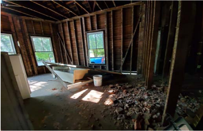
Photo 7 – Debris scattered throughout structure.
