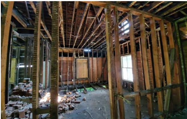
Photo 9 – Remnants of fireplace and missing floor front right area of structure.
