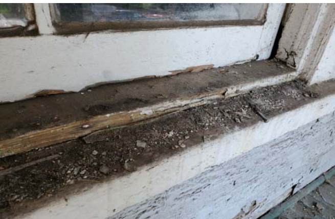
Photo 5 – Remnants of glazing between sill and sub sill of window.
