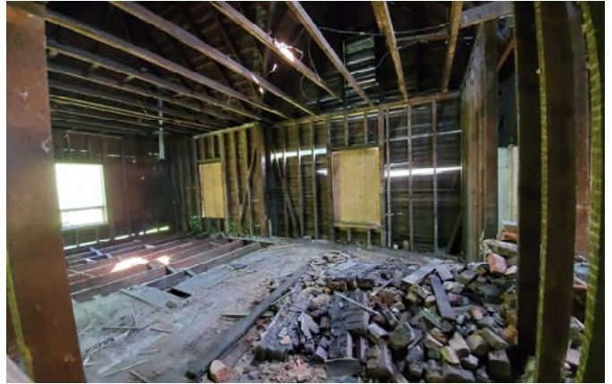
Photo 8 – Remnants of fireplace and missing floor back right area of structure.
