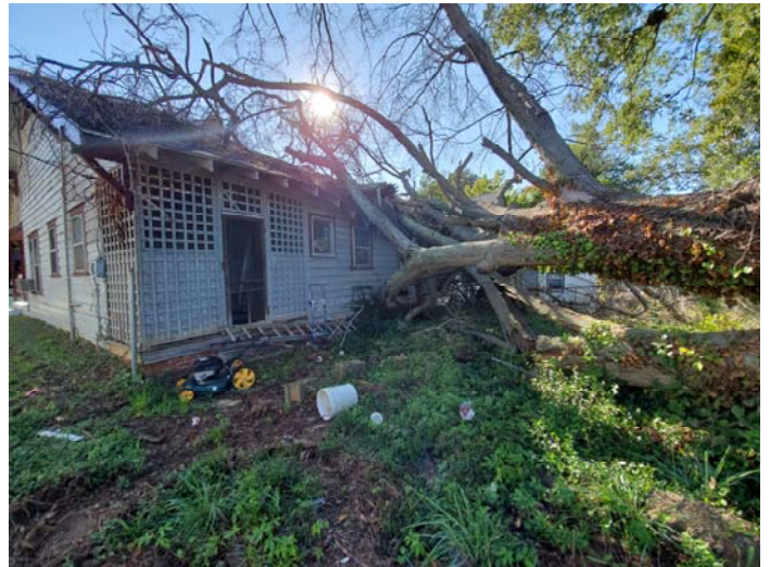
Photo 2 – Damage to back portion of house.
