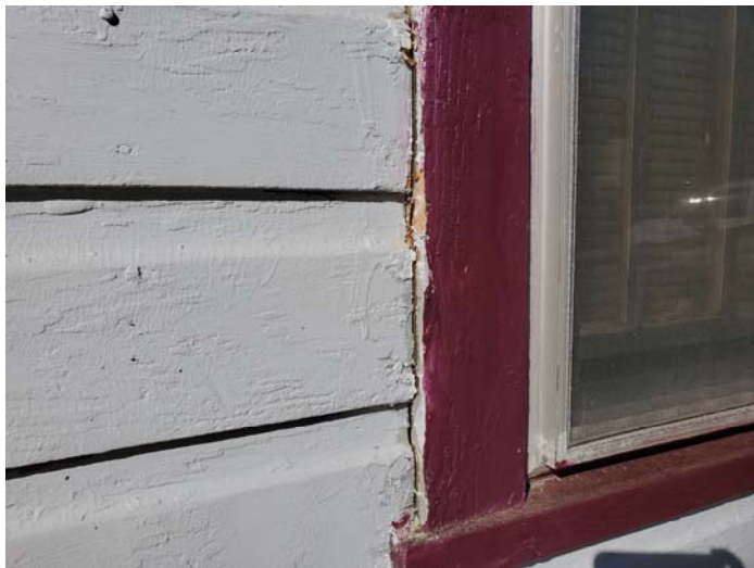
Photo 5 – Casing caulk on doors and windows.
