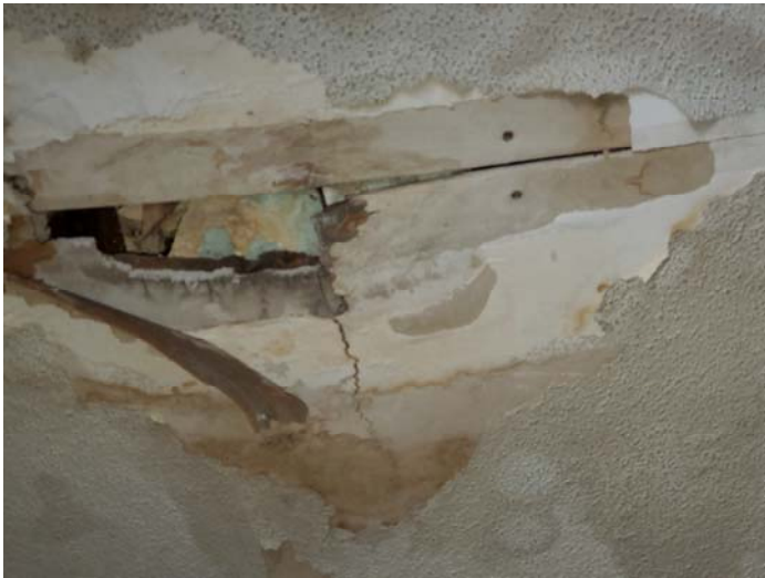
Photo 7 – Ceiling texture, drywall, joint compound & tape throughout ceilings.
