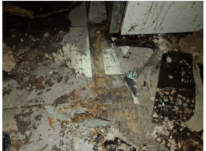
Photo 10 – 12"x12" brown square pattern flooring and associated mastic in kitchen, pantry and hallway is ACM.
