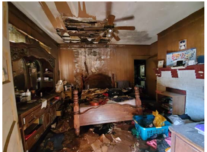
Photo 12 – Damage to ceiling throughout the house.
