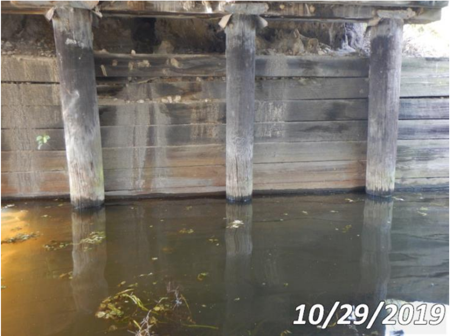
Photo 228-S01 (Unit 0: Timber Pile)
