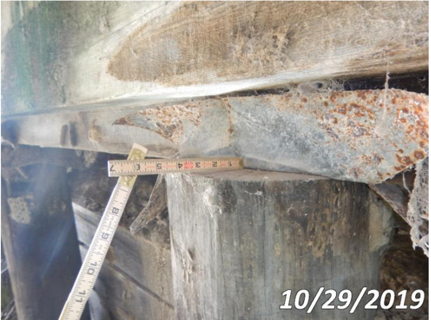
Photo 228-S04 (Unit 0: Timber Pile)
