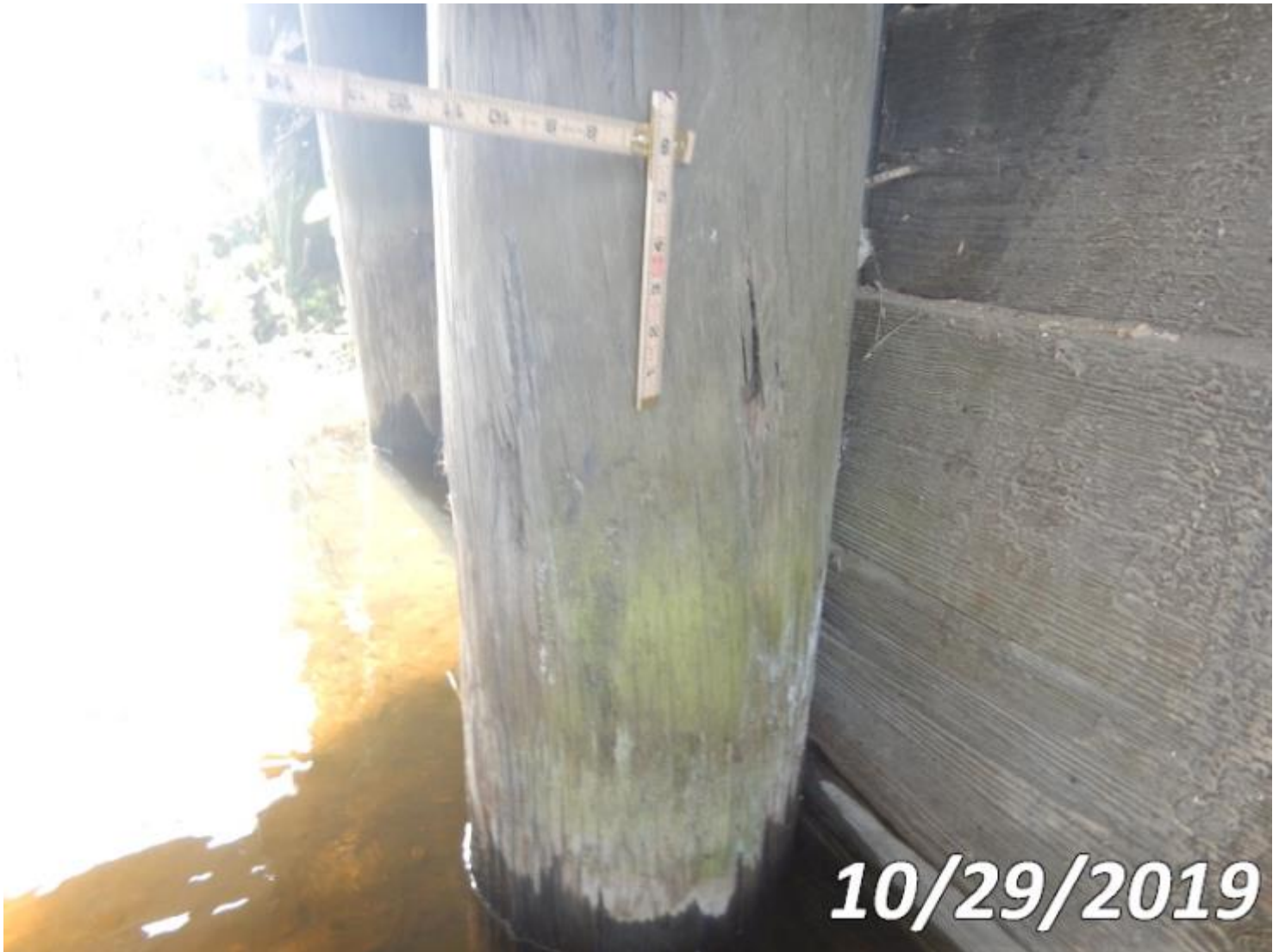
Photo 228-S02 (Unit 0: Timber Pile)
