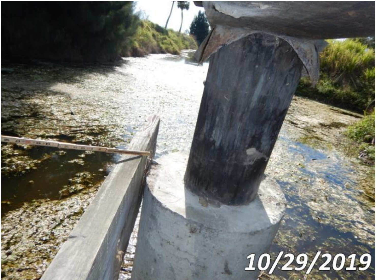
Photo 228-S03 (Unit 0: Timber Pile)
