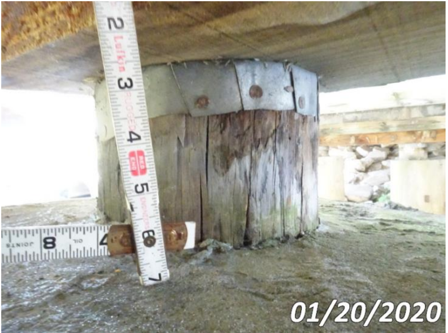
Photo 228-S01 (unit 0: Timber Pile)
