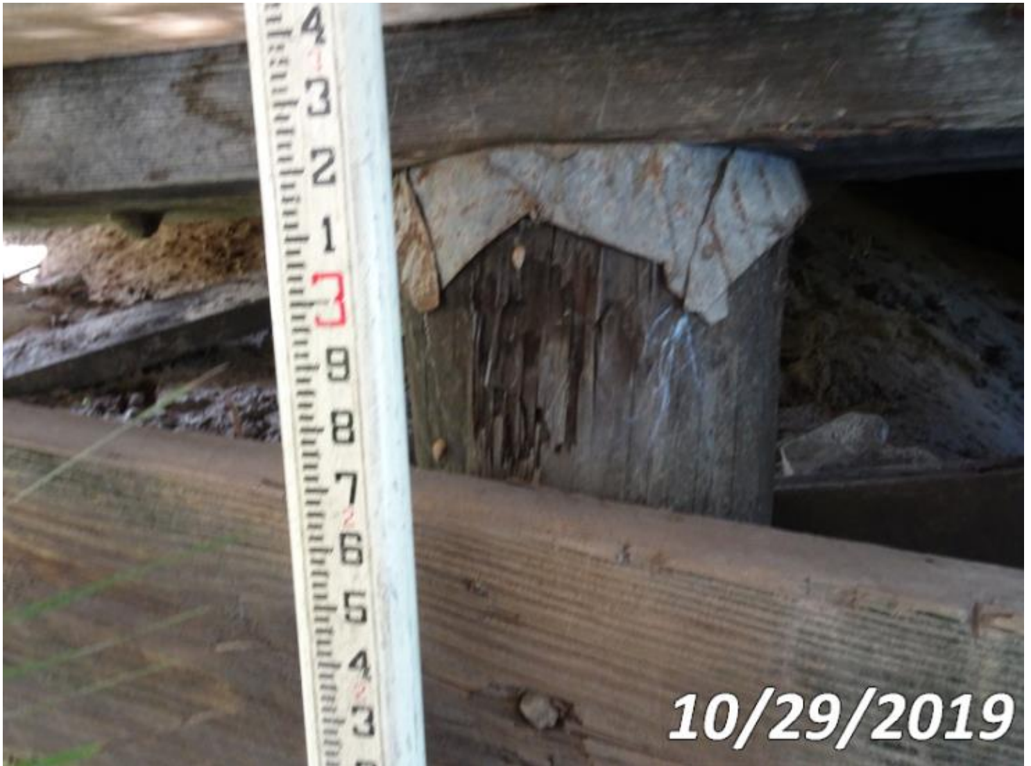
Photo 228-S02 (Unit 0: Timber Pile)
