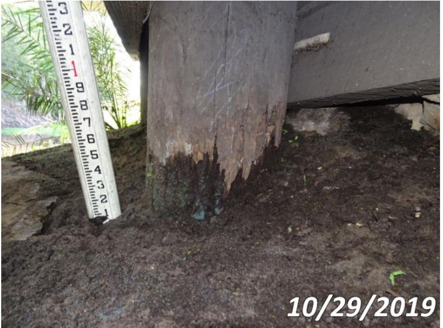
Photo 228-S01 (Unit 0: Timber Pile)
