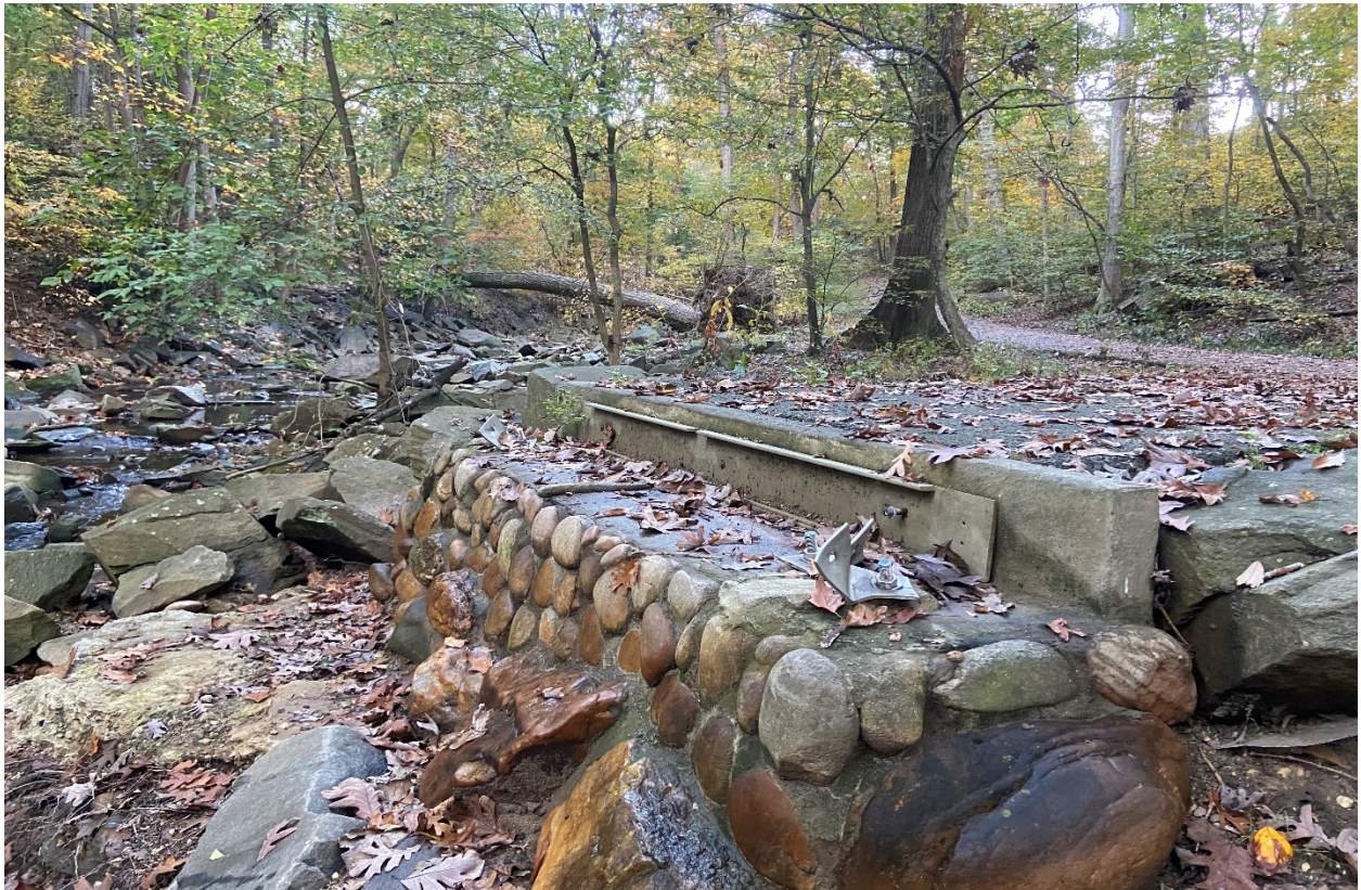
Picture 2: Right and Left Abutment remains after the existing bridge has been washed out. (Picture taken 10-22-2020)
