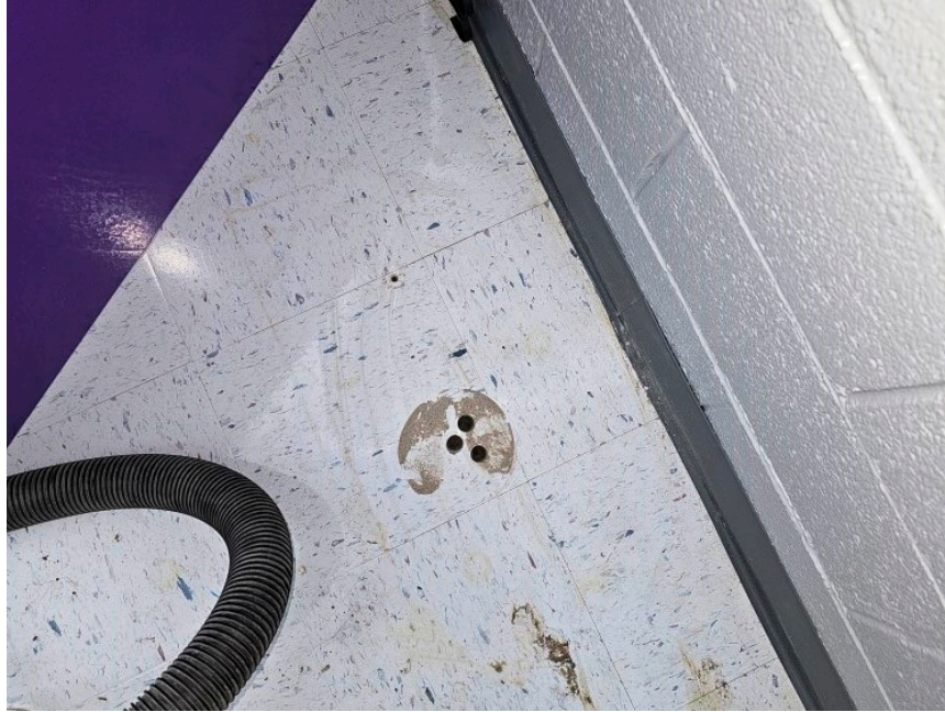
Figure 2: View of Test Suction Point B (Room #26)
