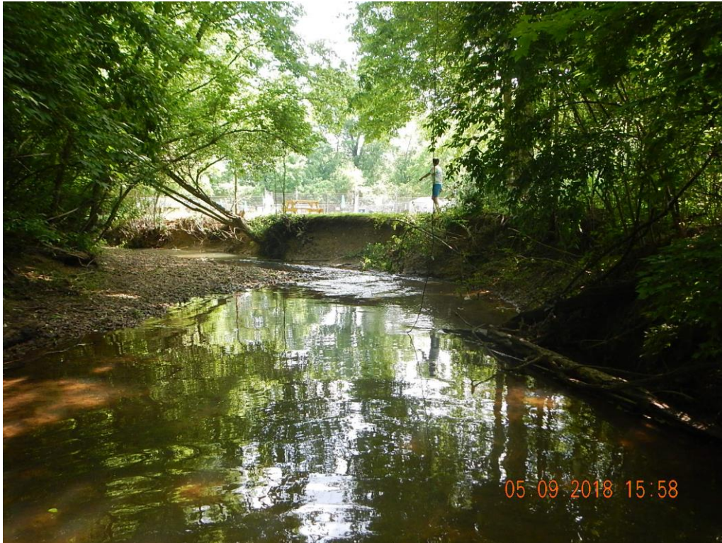
Figure 2 Downstream view from broken pipe looking at the right bank erosion
