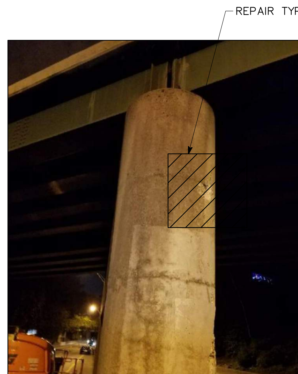
6 REPAIR PHOTO SCALE: NOT TO SCALE
