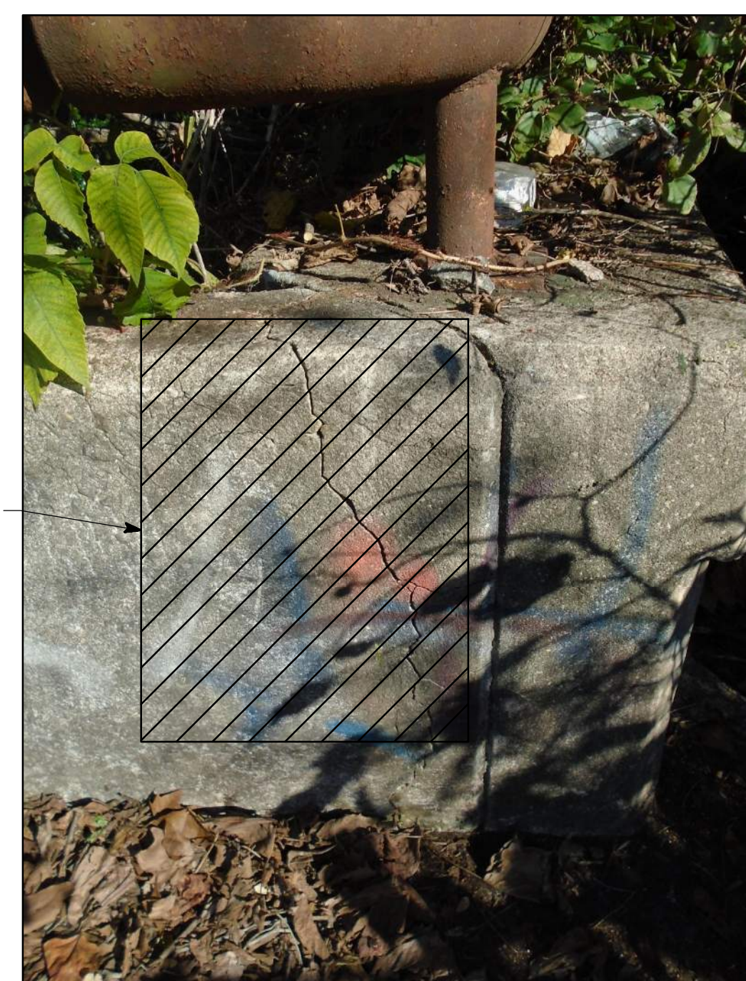
7 REPAIR PHOTO SCALE: NOT TO SCALE
