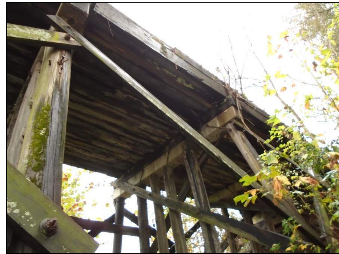
4 REPAIR PHOTO SCALE: NOT TO SCALE
