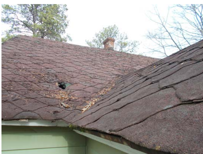
Photo 5 – Six layers of roof shingles and no felt (red diamond shaped shingles).
