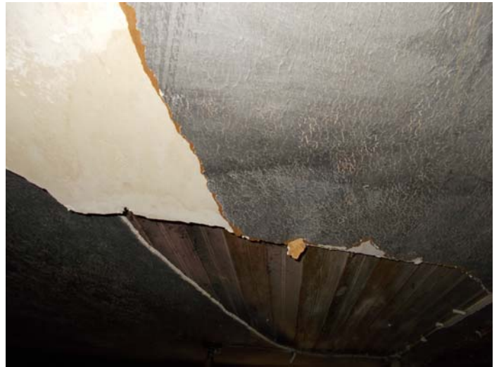
Photo 14 – Light ceiling texture in the back left bedroom.
