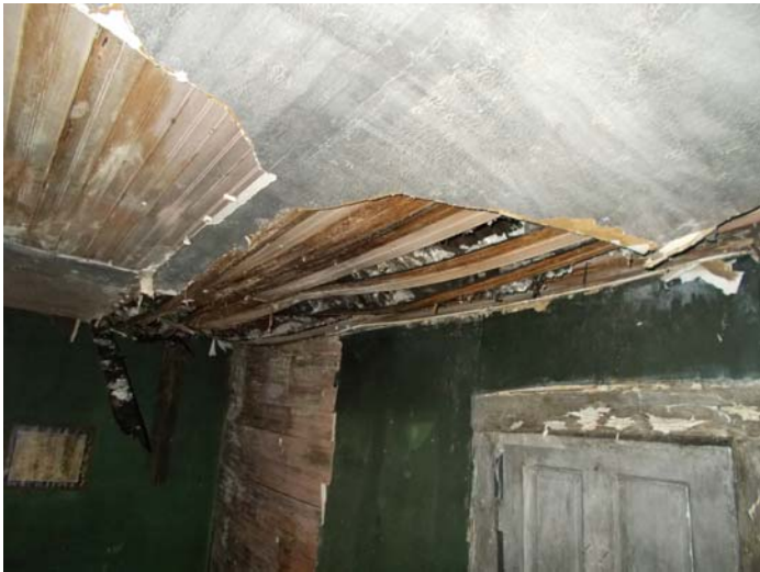
Photo 19 – Drywall, joint compound and tape throughout.
