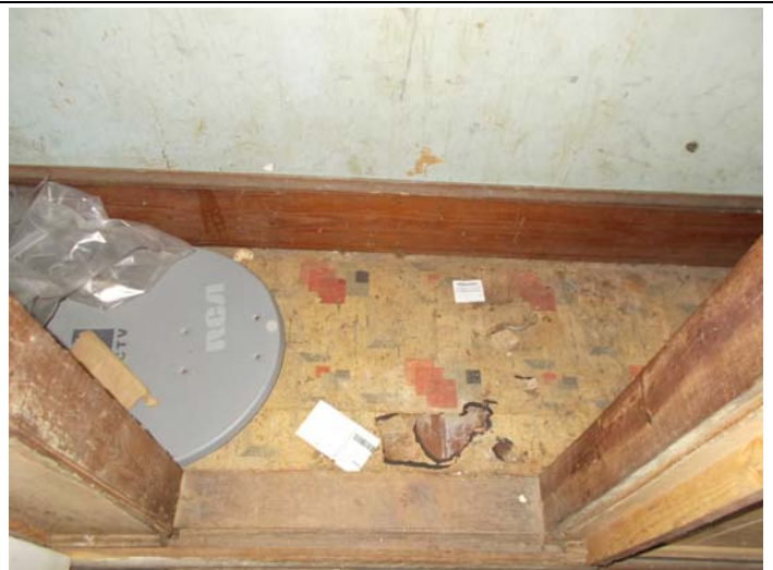
Photo 16 – Two layers of vinyl flooring with no mastic in the closet of the large middle room in front of the kitchen.
