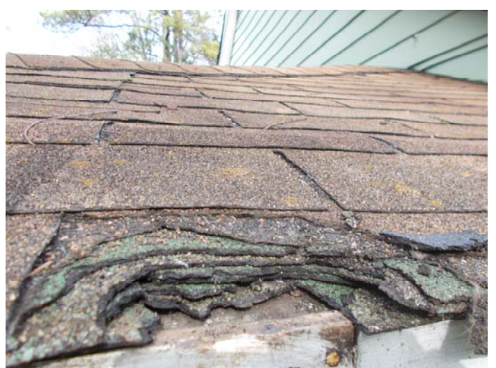
Photo 6 – Eight layers of roof shingles and no felt (brown rectangular shaped shingles).
