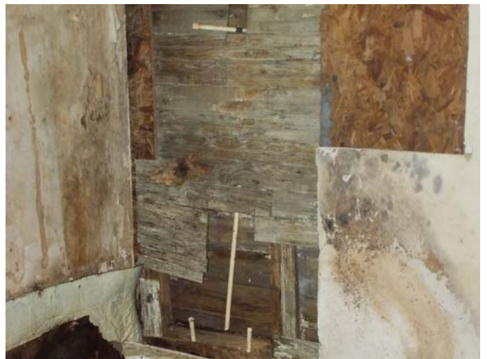
Photo 18 – Wall panel mastic in the bathroom.
