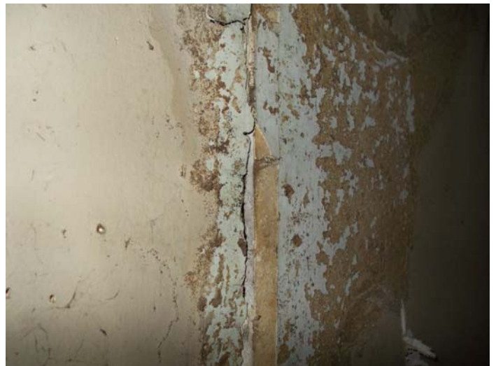
Photo 22 – Drywall, joint compound and tape throughout.
