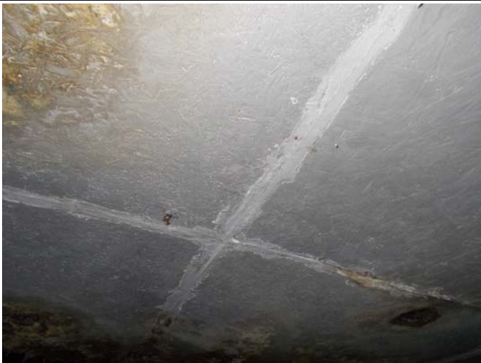
Photo 21 – Skim coating on seams of plywood ceiling in the large middle room in front of kitchen.
