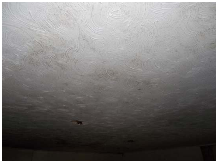
Photo 12 – Swirl ceiling texture on the living room ceiling.
