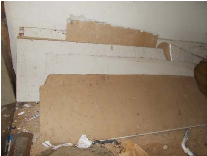
Photo 3 – Unfinished drywall inside the shed.
