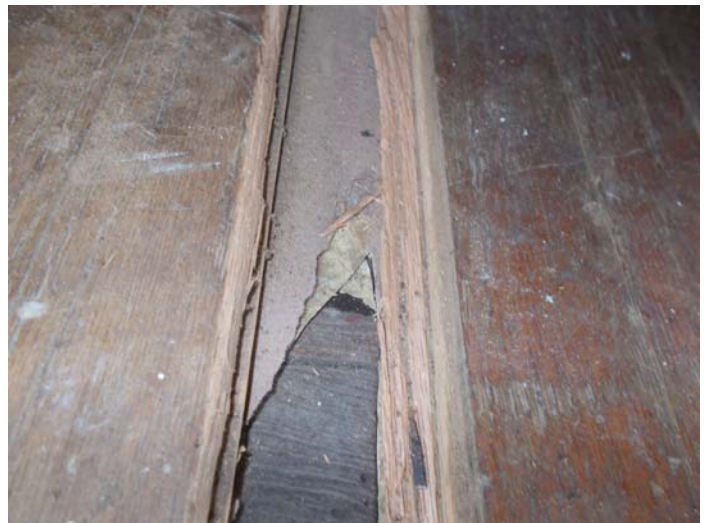
Photo 10 – Tan pattern vinyl flooring with brown paper and no mastic under wood in the living room.
