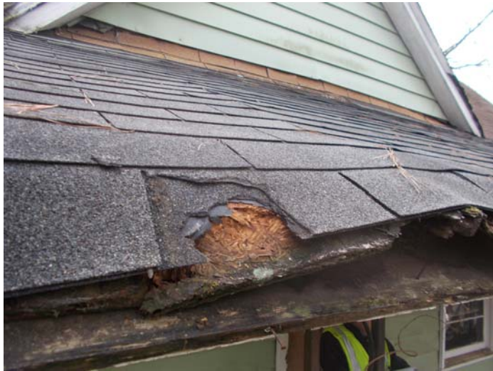
Photo 7 – Two layers of roof shingles and one layer of felt on front porch roof.
