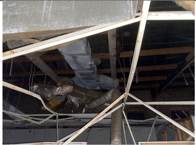
HVAC (Fiberglass) – North Office Section
