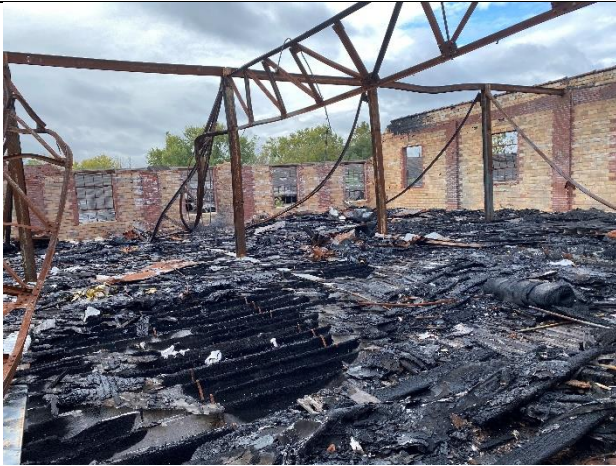
Fire Damaged 2 nd Floor – NE Section
