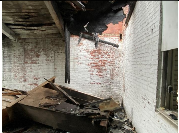
South Bay of Facility – Damaged Roof
