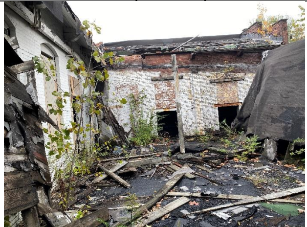
Fire Damaged South Section of the Facility
