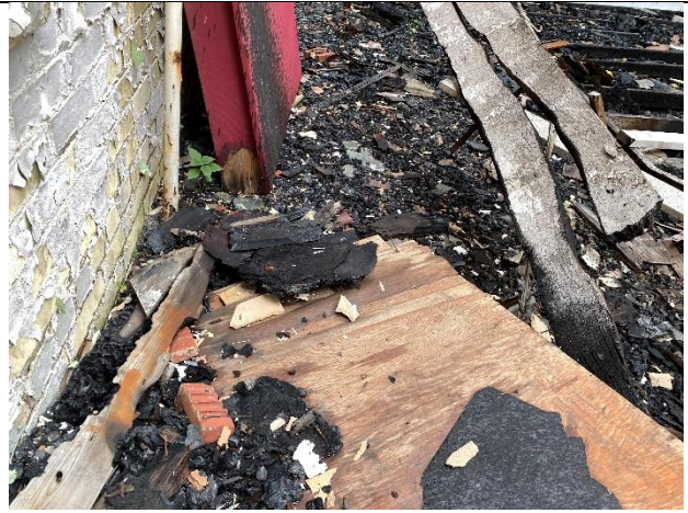
Fire Damaged Roof – NE Section of Facility
