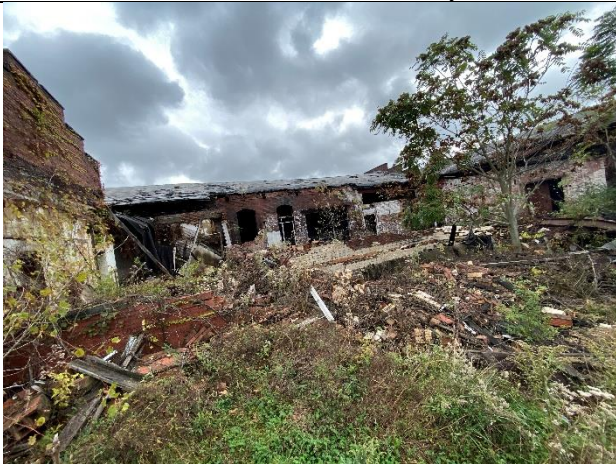
West Fire Damaged Section of Facility
