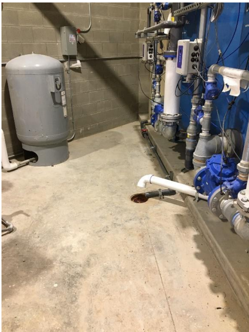
View inside tank room:
