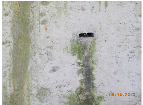
Bent 3 cap has a 1" x 3" void from a piece of wood from construction, extending all the way through the cap. ( Specialized )
