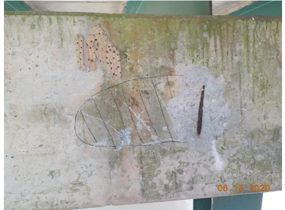
Bent 3 cap, rear face has a 10" x 14" x 2" D spall with exposed rebar and a 18" x 12" area of delamination under beam 1. ( Specialized )
