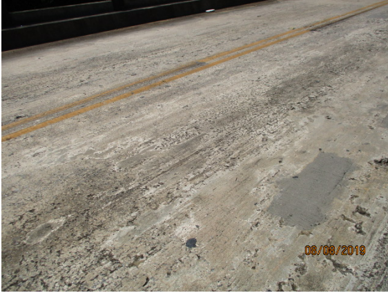
Span 2 showing delamination and abrasion.
