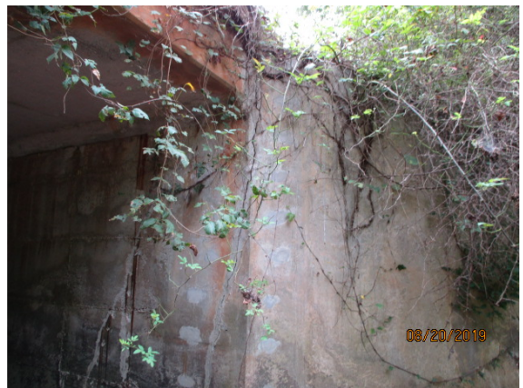
Cracking at the rear inlet wingwall
