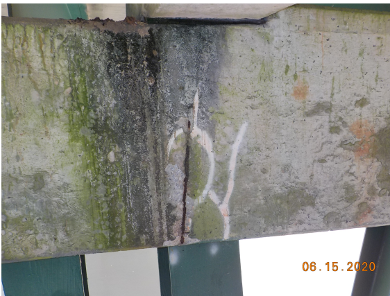
Bent 3 cap, rear face has a 4" x 19" x 1" D spall with exposed rebar under beam 2. ( Specialized )
