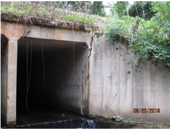
Crack has re-opened in rear outlet wing
