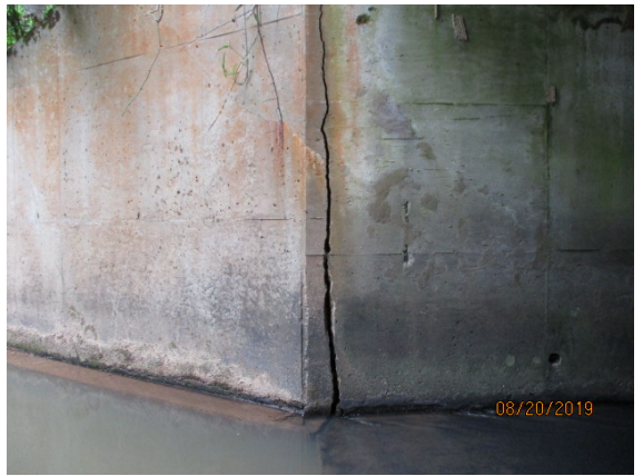
Crack measuring 3" wide x 11' tall
