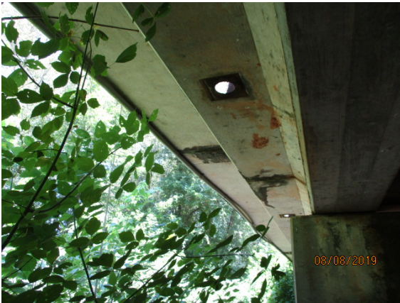
1.5" PVC Telephone conduit left side under the edge of the overhang.
