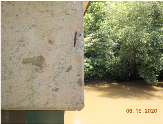
Bent 3 cap, right rear corner has a 4" x 14" delamination with a 3" x 6" x 1.5" D spall with exposed rebar. ( Specialized )
