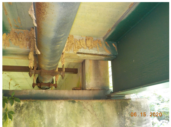
Span 4 bay 4 forward edge beam has a spall with 24" of exposed rebar. ( Specialized )
