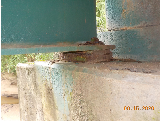
Span 3 rear, bearing 5 has moderate corrosion. ( Specialized )
