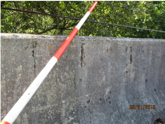
Typical spall with exposed rebar in the barrier walls in span 2
