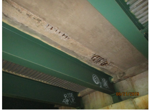
Spall/delamination with exposed rebar in deck underside in span 4.
