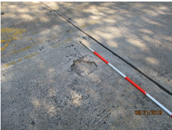
Spall in span 4
