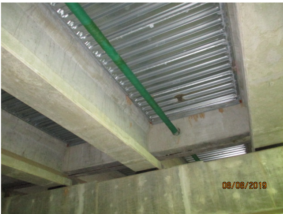
Gas line bottom left between beams 1 and 2.
