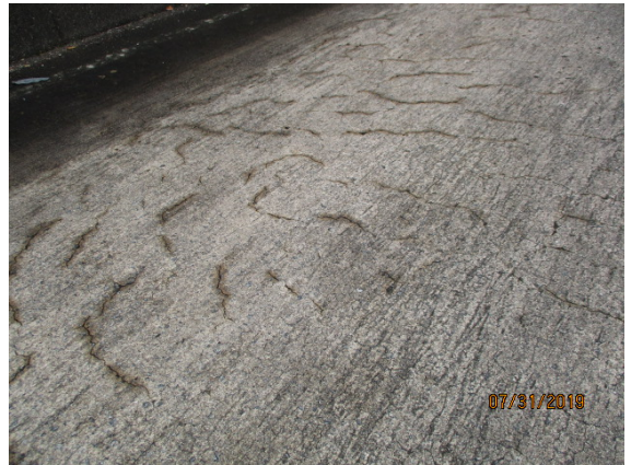
Typical cracking in the deck top. Span 2 shown.
